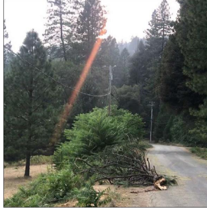
Figure 4: Image of Vegetation Related Damage in Nevada County – Falling Treetop Damaged Primary Overhead Conductor and Broke Crossarm
