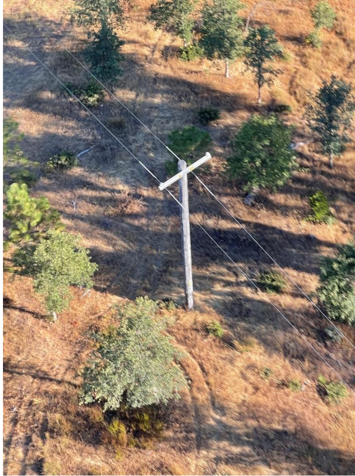
Figure 15: Vegetation-Damage in Shasta County – Broken tie wire
