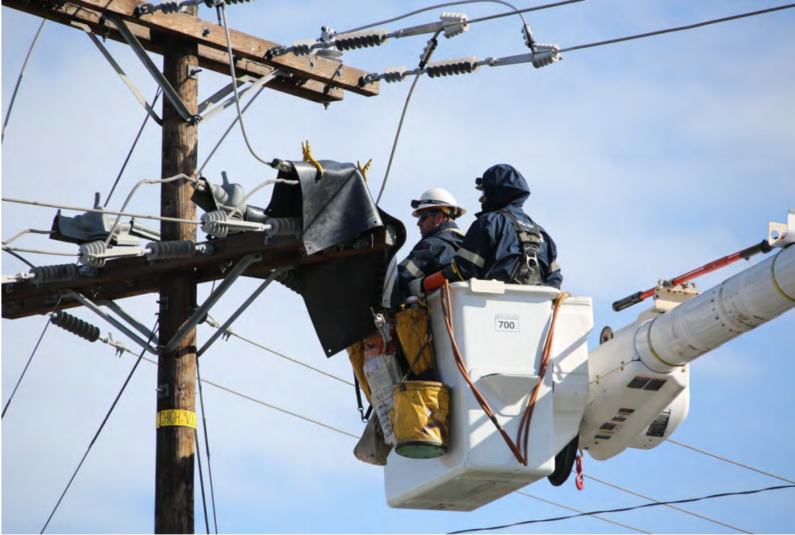
Photo B-2. Example of Utility Conducting Pole Top Repairs from a Utility Bucket Truck
