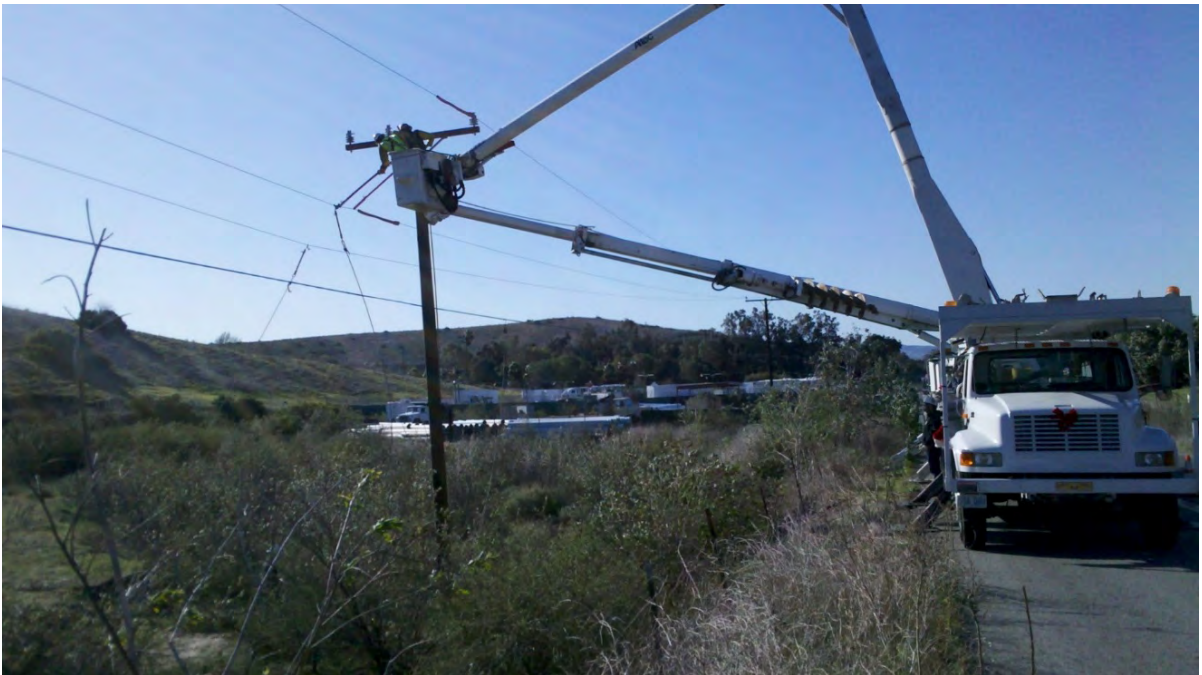
Photo B-12. Use of Line and Boom Truck to Pull Existing Pole from Ground and Place New Pole in Existing Hole
