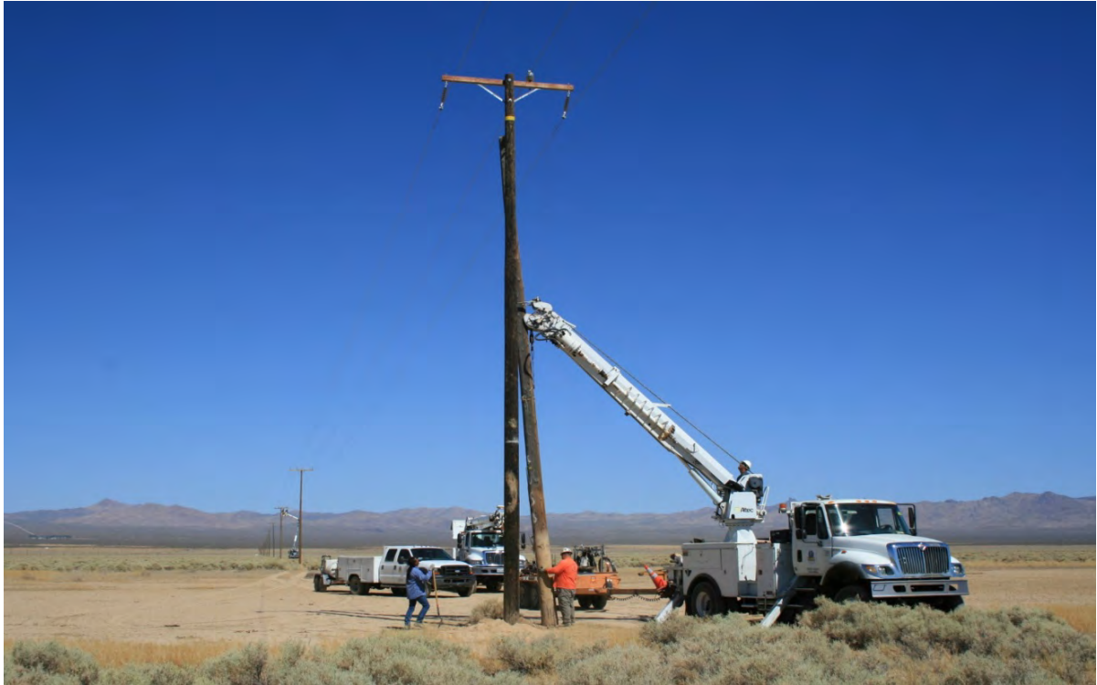
Photo B-13. Use of Line and Boom Truck to Pull Existing Pole from Ground and Place New Pole in Adjacent Hole
