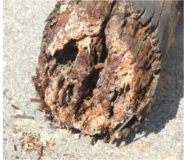
Photo B-6. Pole Split inside a Pole
