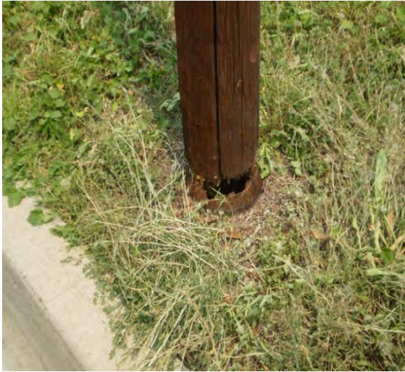
Photo B-5. Examples of Pole Decay at Base of a Pole
