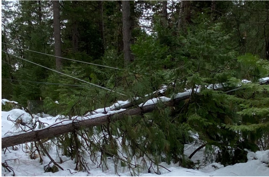
FIGURE PG&E-22-11-3: COVERED CONDUCTOR EFFECTIVENESS – EXAMPLE 3
