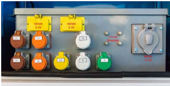
Figure 3-6 Export Power Panel
