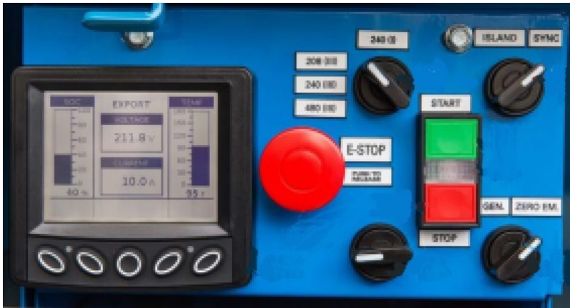
Figure 3-8 Export Power Unit (EPU) Control Panel
