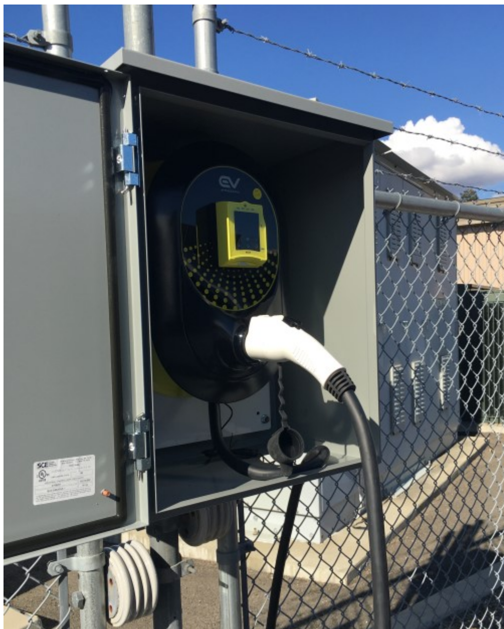
Figure 22. Commercial Integrated NGM EVSE - San Ramon ATS
