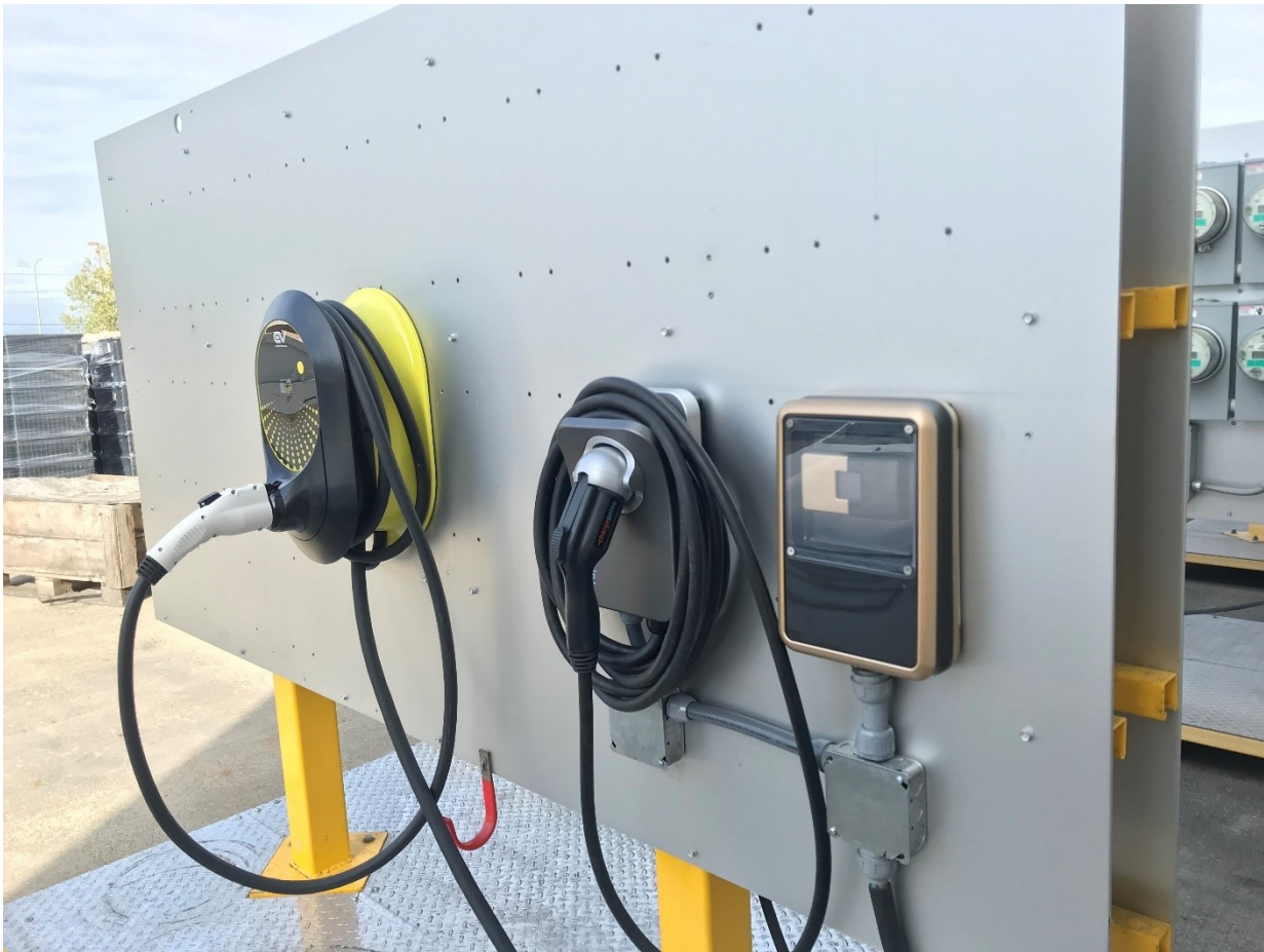
Figure 21. Integrated and Retrofit NGM EVSE Installs - Fremont Meter Farm
