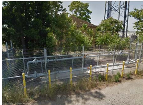
Figure 10 – District Regulator Station — Above Ground
