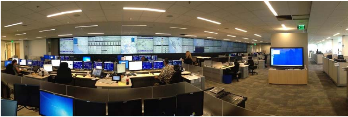
Figure 38 – PG&E’s Gas Control Center features a 90 foot-long video wall with current operational information to augment the Gas SCADA system
