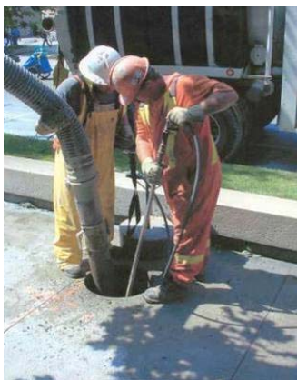
Figure 56 – PG&E Crew Using “Keyhole” equipment to access facilities in a minimally invasive manner.
