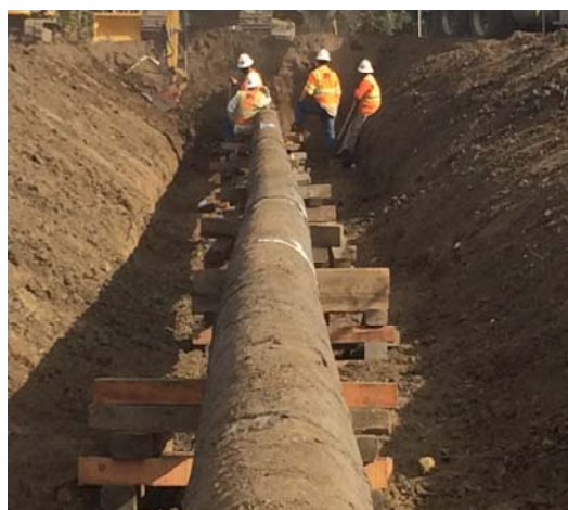
Figure 26 – Pipeline 2BA As-found Condition After the 2014 Napa Earthquake
