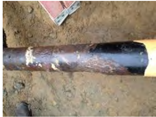
Figure 24 – Example of Corroded Pipe
