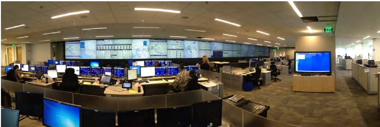
Figure 38 – PG&E's Gas Control Center features a 90 foot-long video wall with current operational information to augment the Gas SCADA system
