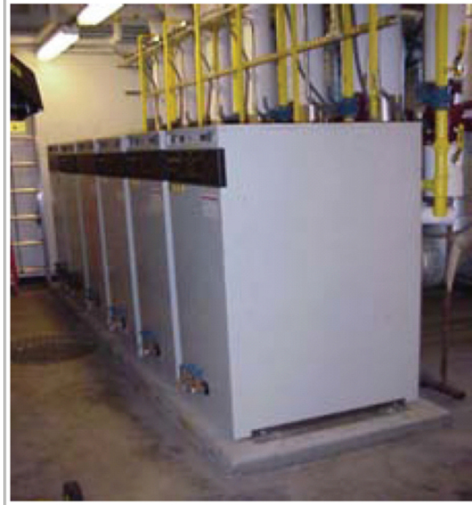
Figure 6.02 LBNL replaced two boilers with 11 modular boilers to maximize part-load efficiency. (Source: LBNL)
