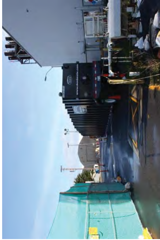
GWTS storage tanks throughout site.
