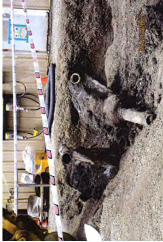
ACM transite pipe with thrust blocks.
