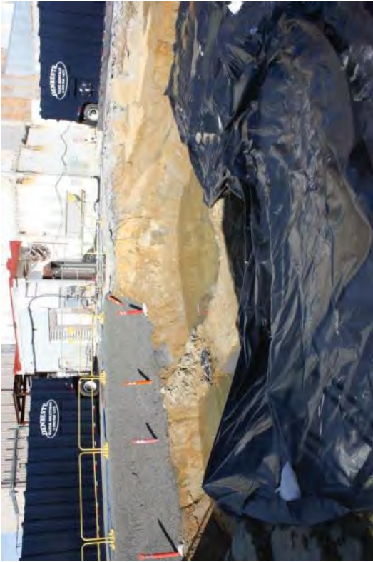
GWTS storage tanks throughout site.
