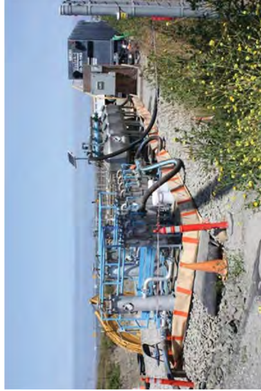
New sand filters for the GWTS.
