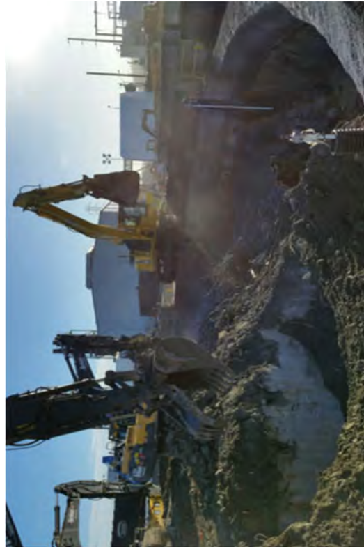
Accessing the West Suppression Chamber.
