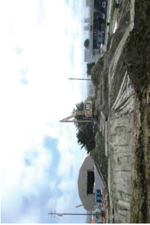
12kv electrical power lines were rerouted to allow for higher stockpiling.
