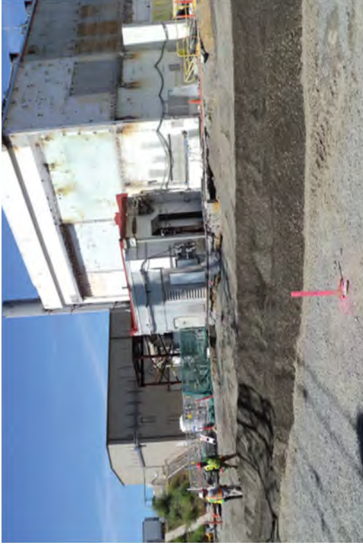
The backfill of this supplemental work area next to the PEG room nearly complete. This completes the portion of CSM Unit 2 pre-trench section.
