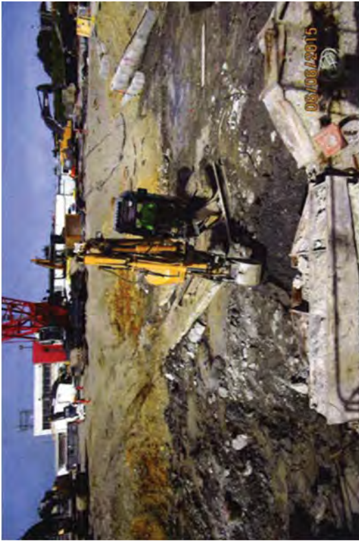
Grading the west end of the excavation to prepare it for FSS.
