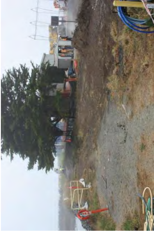
The Discharge Canal and GWTS area ready for the pretreatment system installation.
