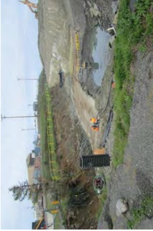
There was a constant in-flow of water from a spring and the underground water table.
