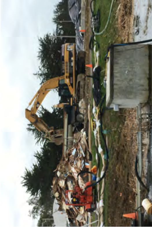
Loading out concrete demolition waste from the Assembly Building to be processed.
