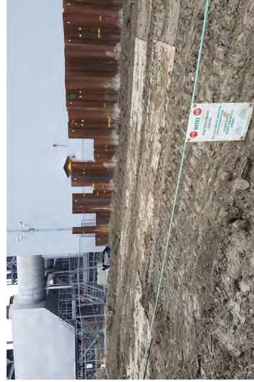
Sheet piles ready to be removed after the are was compacted and the FSS is complete.
