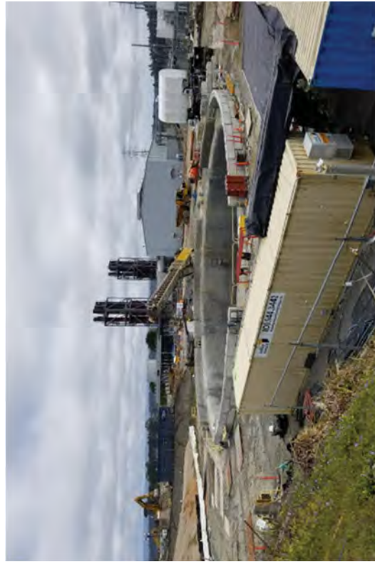
The layout of the Caisson excavation area after demobilizing the removal equipment to allow for remaining backfill operations.
