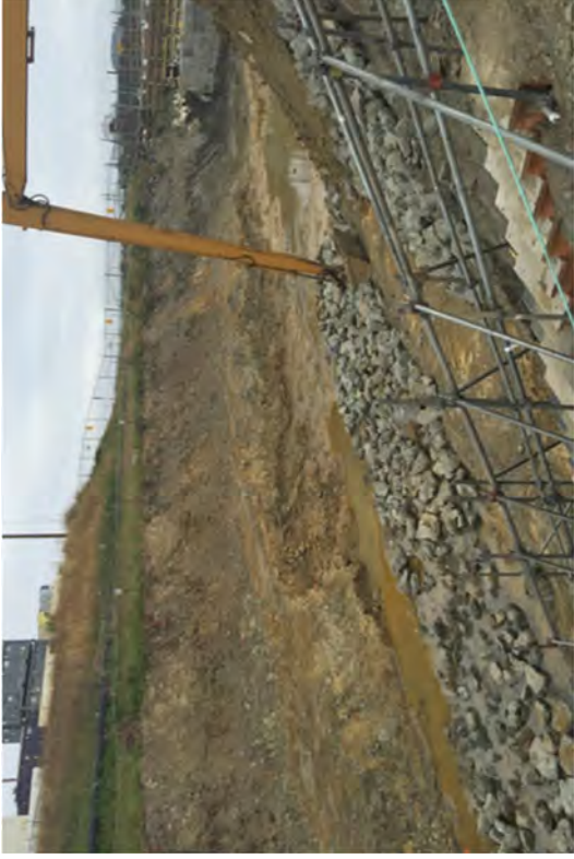
Installing reused riprap into the bottom of Canal after it cleared FSS.
