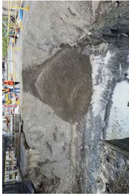
Backfilling the SAS excavation with a stone fill that was specified by the engineering staff.
