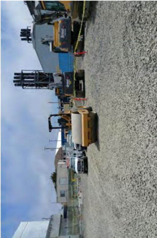
The equipment that was used to compact the work surfaces for the large hydromills.
