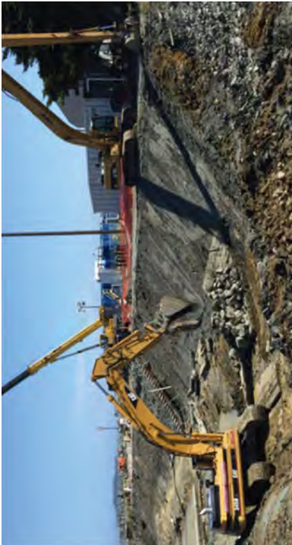
Smoothing the slope and removing the last pieces of riprap from the South east end of the canal.
