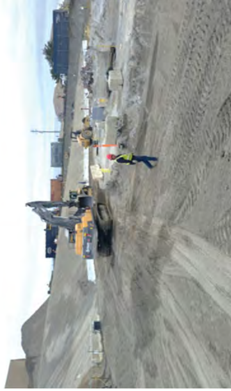
Excavation for the utility trench and grading so that the impermeable layer could be laid down.
