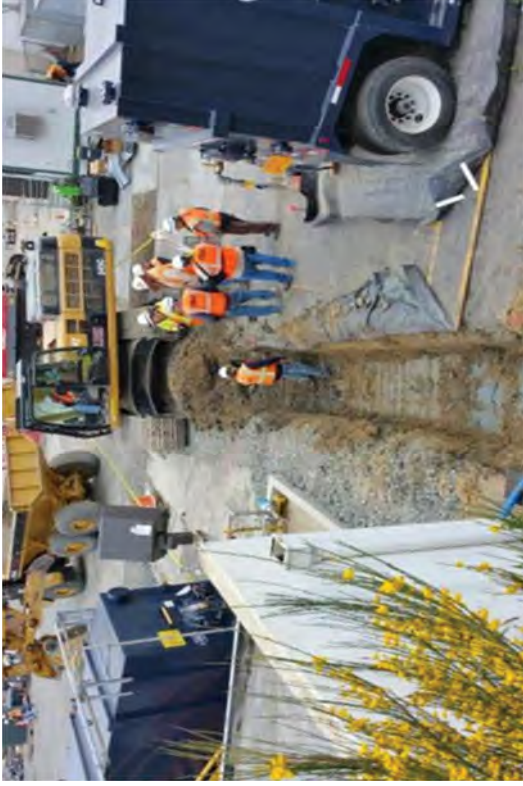
Digging an electrical trench to route powerlines for CSM and CLSM equipment.
