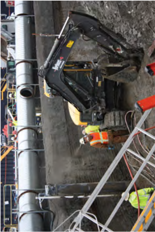
Applying a second layer of shotcrete to the shotcrete collar down to approximately -2' EL.
