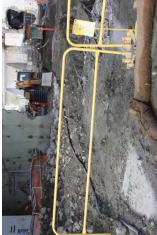
Debris from the first demolition phase of the RFB was placed into below-grade voids like the SFP.
