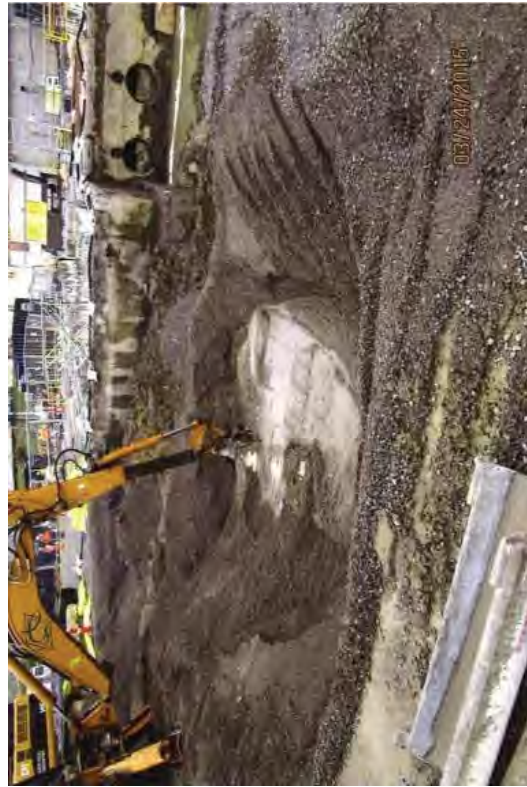
Plugging the Circulating Water Pipe with CLSM allowed backfilling to continue in the HMS Trench.
