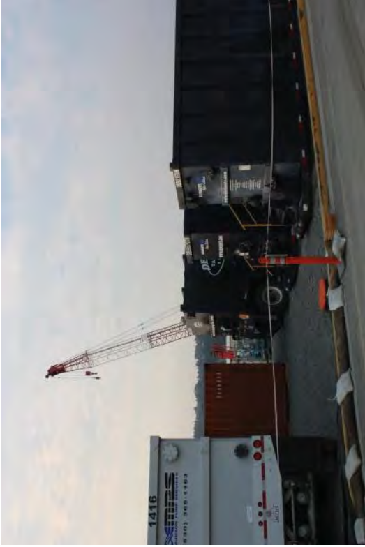
The GWTS 2 control station inside the retention berm area.
