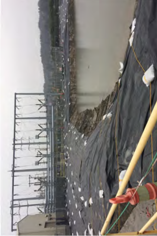
SWPPP Controls for turbidity reduction.
