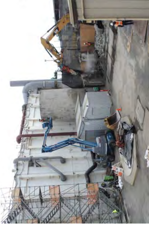
Demolishing the south wall with an excavator and the aid of a spotter who provides dust suppression and constant communication regarding projectiles.
