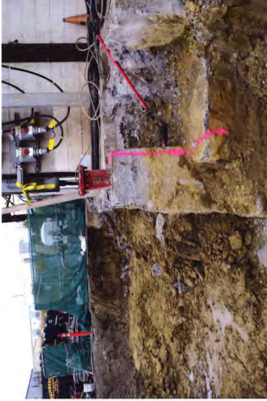
A corner had to be removed from an extension of the RFB, called the PEG room, because it partially encroached on the CSM footprint.
