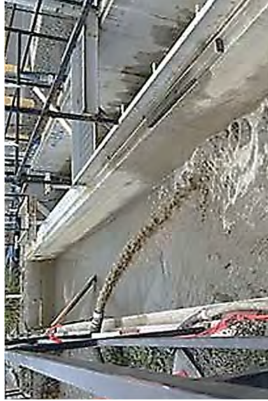
TB excavation water being pumped to the OWS for settling and processing.
