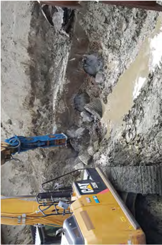
Exposing and removing the first segments of pipe. At this time the bladder bags were still inserted approximately 6 feet into the pipes.
