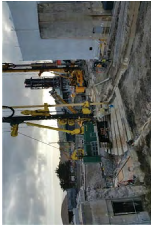
Using the hydromills to install CSM panels while circling the Caisson structure in a clockwise direction.
