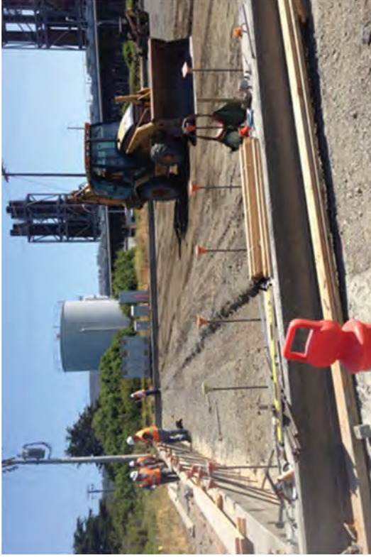
Stripping the forms from the foundation and spreading gravel to install the pad and a drain.
