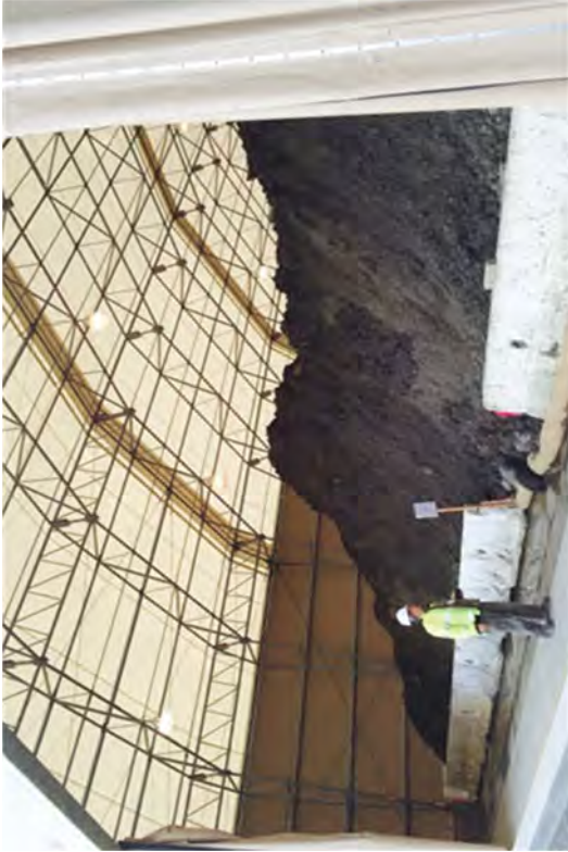
The SMF filled with re-use soils which will be stockpiled in the Discharge Canal.
