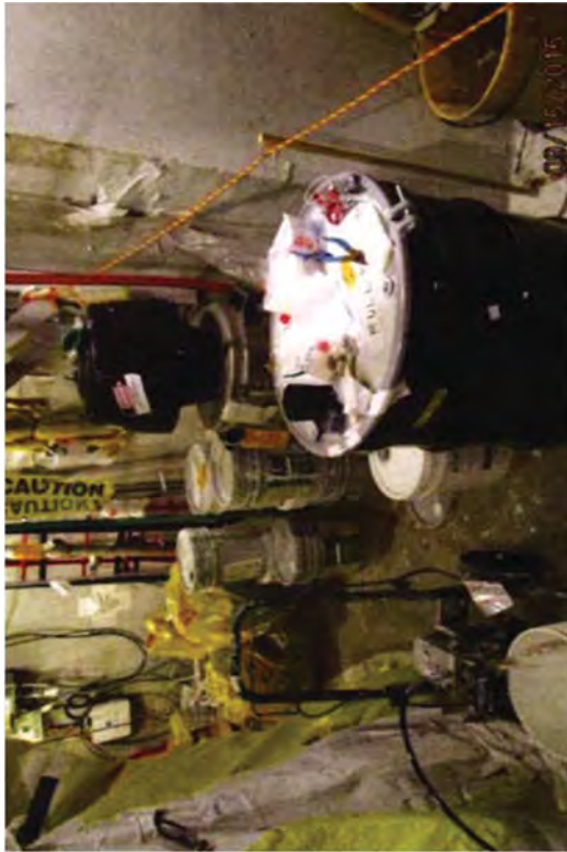
Waste identified for removal at -66' EL.
