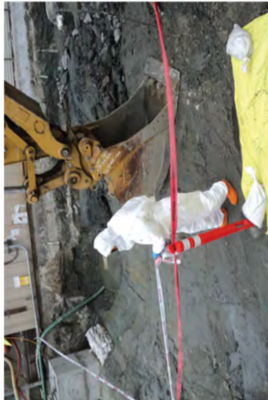
An abatement contractor removes the Asbestos warning tapes surrounding a mitigation area.
