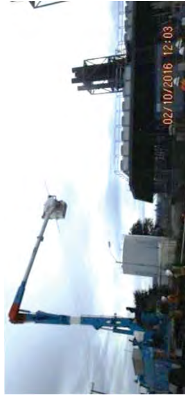
Removing the power line that crossed over the south Discharge Canal work area.
