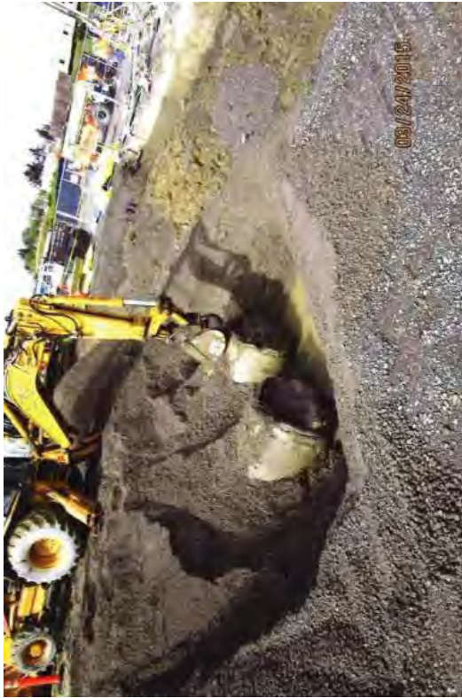
Preparing to cut off the Circulating Water Pipe in the HMS Trench using CLSM.
