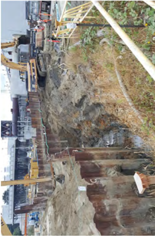
Loading out soils from the excavated west wing area so that sheet pile on the west side of Area D can be removed.
