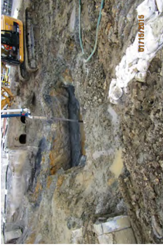
Pumping CLSM into a deep hole left after wooden pilings were extracted.
