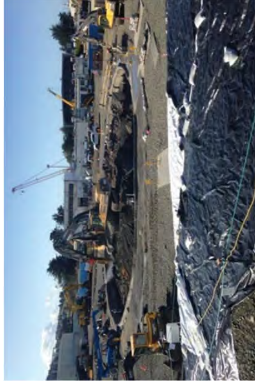
Starting the +12' EL to +8' EL excavation after the slab at +12' EL was fully removed.
