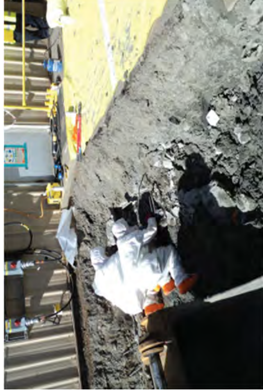
Injecting two-two part epoxy expanding foam into the raceway that remains in the ground.
