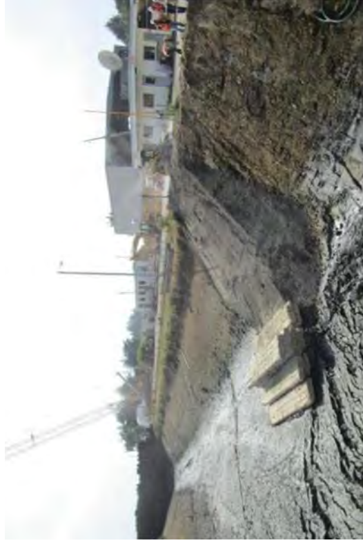
Ramp and crane mats were installed so that an excavator could move into the canal.
