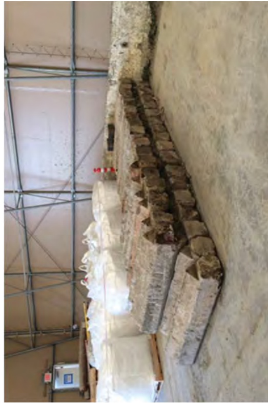
Concrete piles removed from the Discharge Canal outfall structure around the discharge pipes.
