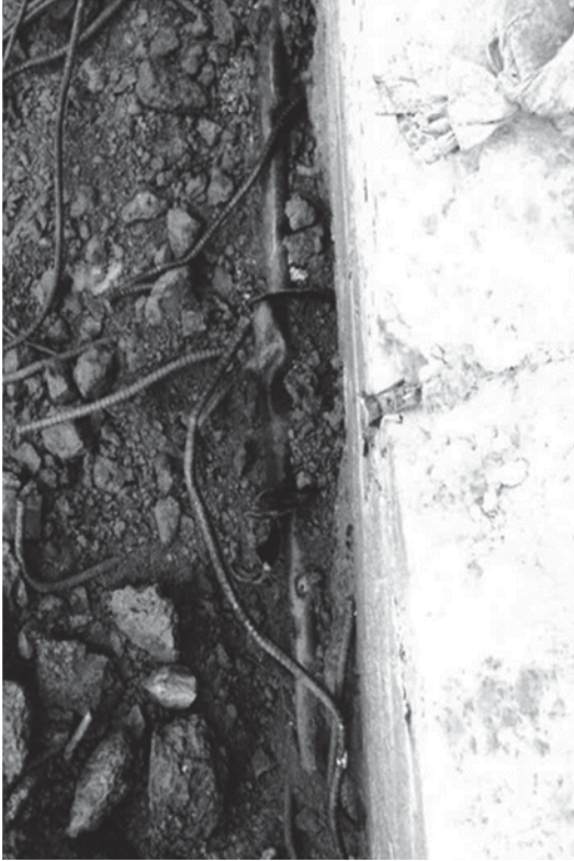
Pipe that RP directs to be placed by machine directly to an intermodal.
