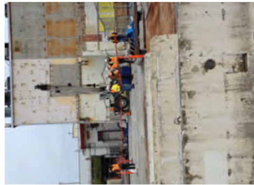
Setting up a boundary, inspecting rigging, and setting up a carry deck crane.
