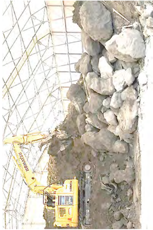
Processing the sacrificial concrete slurry plug from the Discharge Canal and loading it into bags at the SMF
