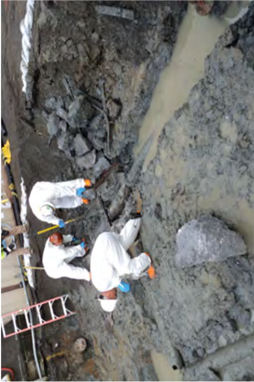
A high concentration of transite pipe in a small area which can only be worked by asbestos trained workers.
