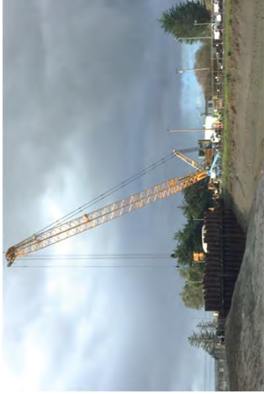
Preparing to pull the first pile from the cutoff wall which will allow the water level to equalize on each side.
