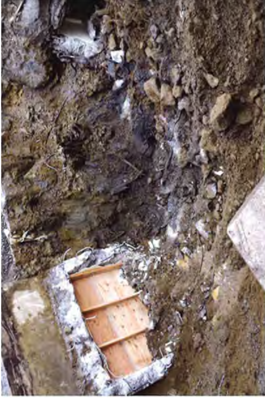
Carefully trimming around the offgas tunnel allowed steel plate to be installed later on.
