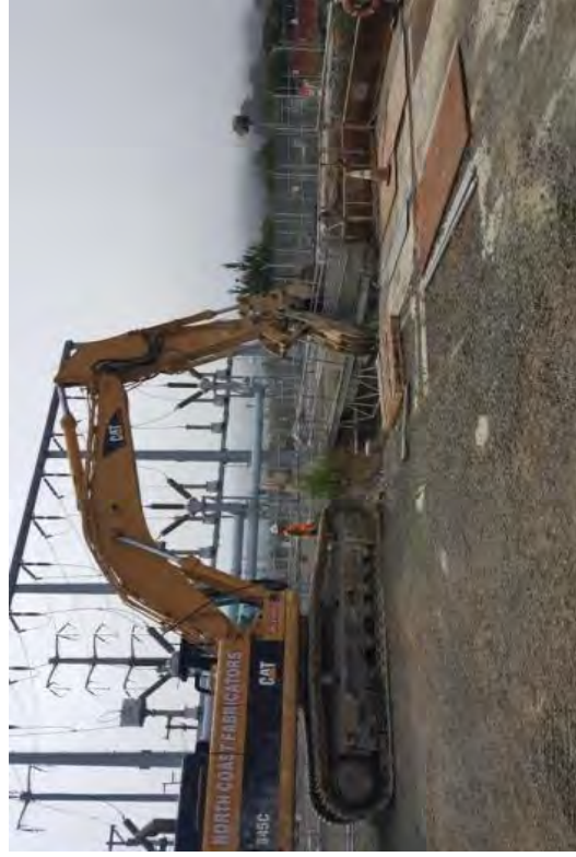
Removing a small pedestrian bridge between the headworks and a storage area for the seaweed net.
