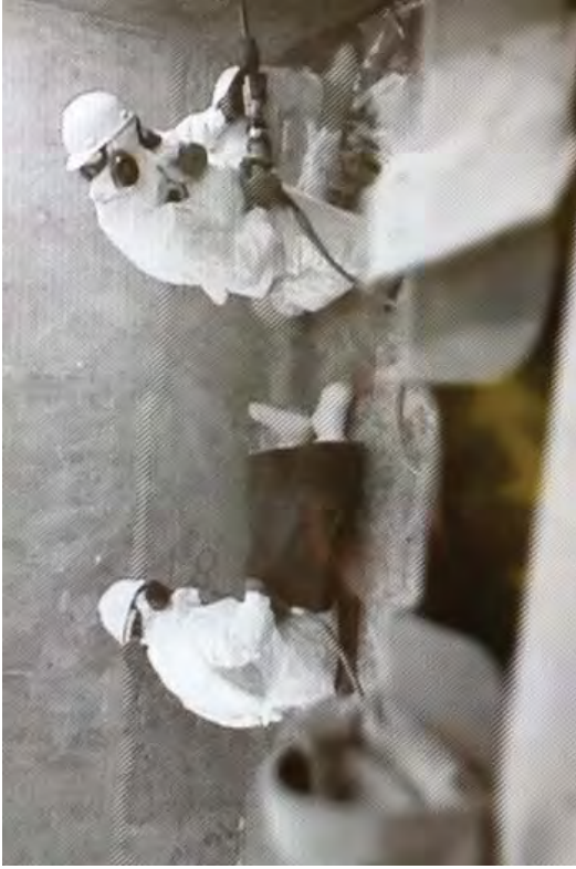
Scabbling the surfaces of the concentrated waste tank room to remove the most contaminated materials.
