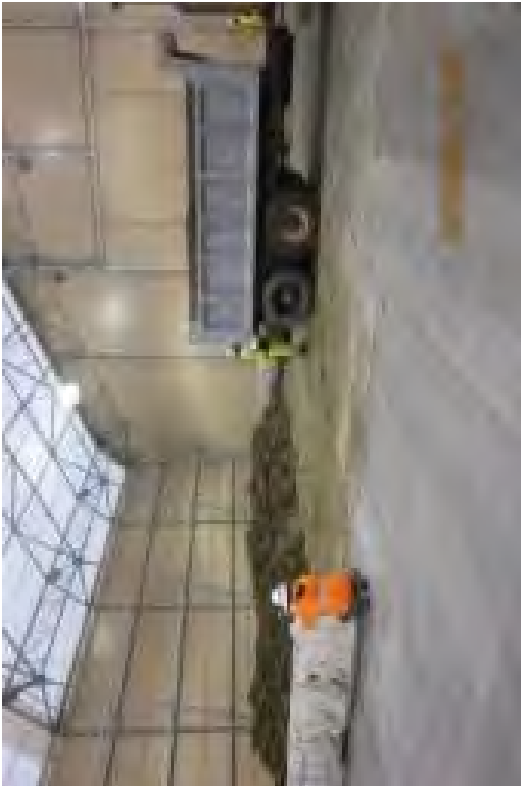
Transferring excavated Unit 2 soil with low or no radioactivity to the SMF for potential re-use.
