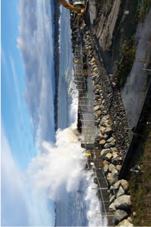
December high tides and storm waves crashing over the sheet pile wall. Note the new riprap structure to keep water out of the canal
