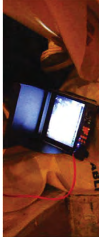
A borescope revealed that the inside of the drain pipe was mildly rusted at its first elbow.
