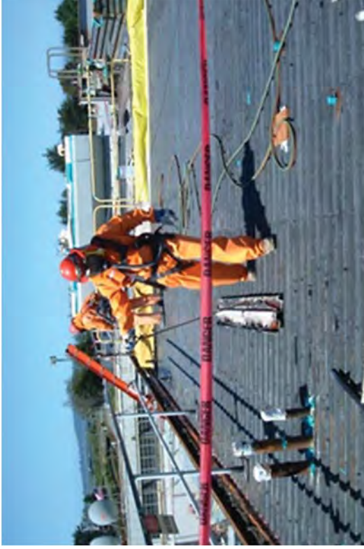
Performing work on a roof required hand rails, a harness with a tie-off, and hazard warning tags.
