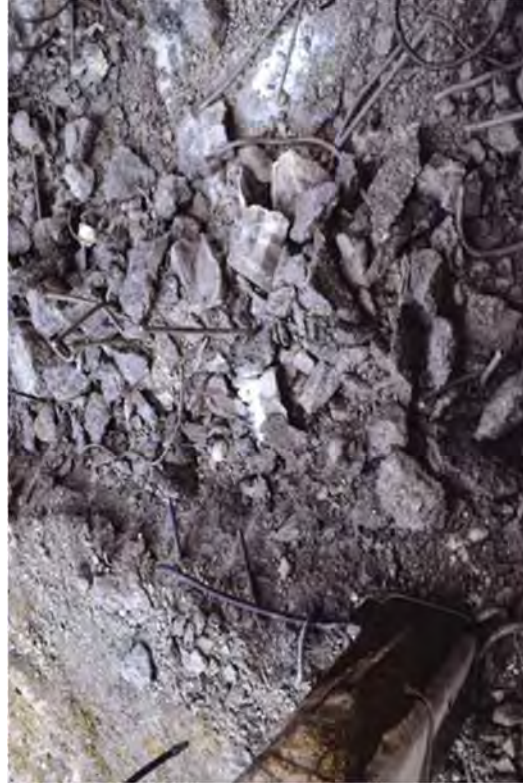
White paint signifies another pipe in the basement to be exposed and placed whole in an intermodal.
