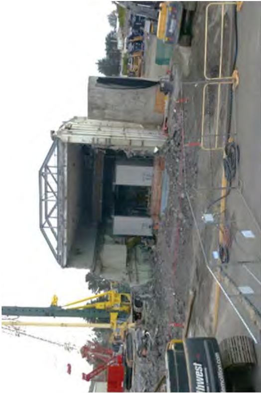
The northern 40 feet of RFB wall removed to make way for the CSM wall.
