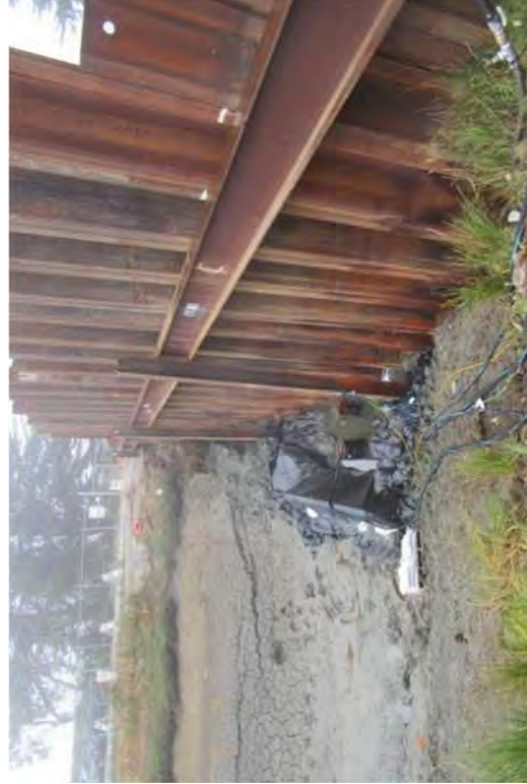
A small containment area built to contain water and aid canal drying.
