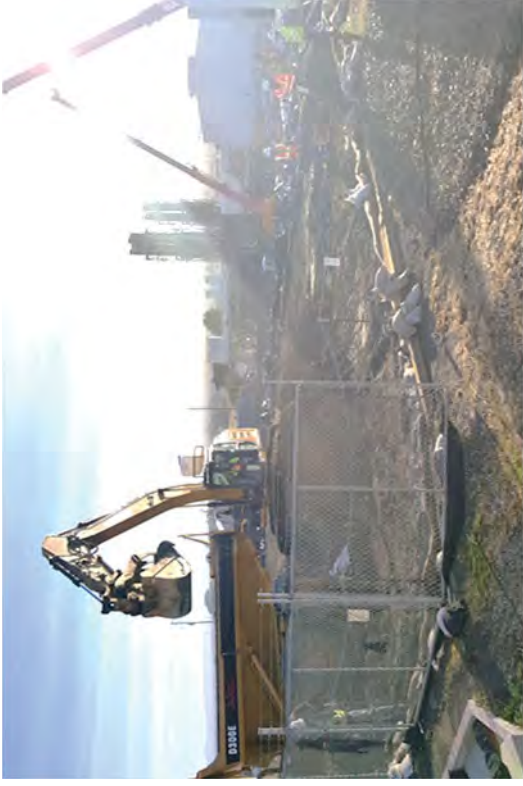
The FSS of upper yard where soils were removed detected some remaining contamination. The RP surveys indicated that an additional 12 inches of material had to be removed.
