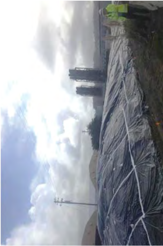
Stockpiled soils were covered to protect them from the seasonal fall rains.
