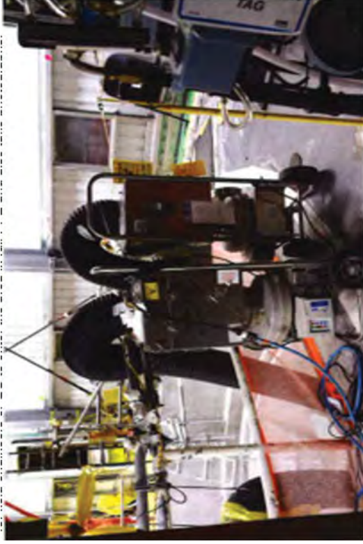
HEPA filtration units and air sample units set up by RP technicians for the drywell pipe cutting and removal process.
