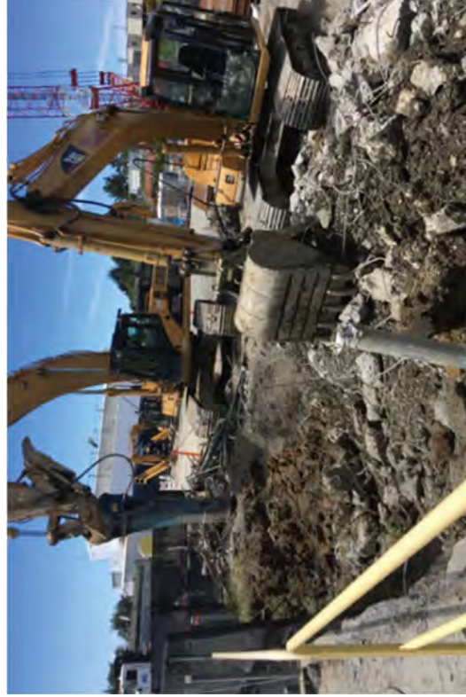
Removing the skimmer oil sump from the south end of the OWS raceway.
