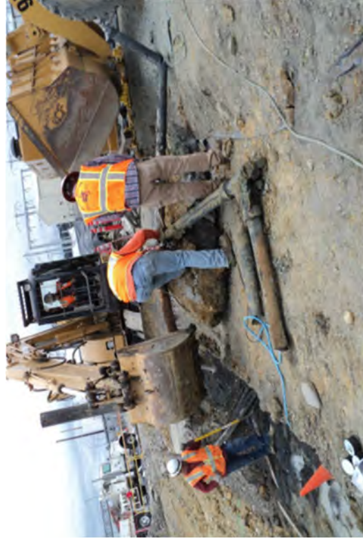
Workers removing and sizing steel pipes. Transite pipe is left in the ground so it can be properly removed.
