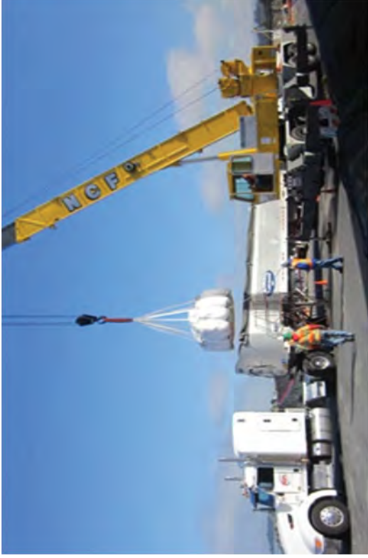
Loading trucks with IP-1 bags for shipment to Redding, CA to be loaded onto Gondola rail car.
