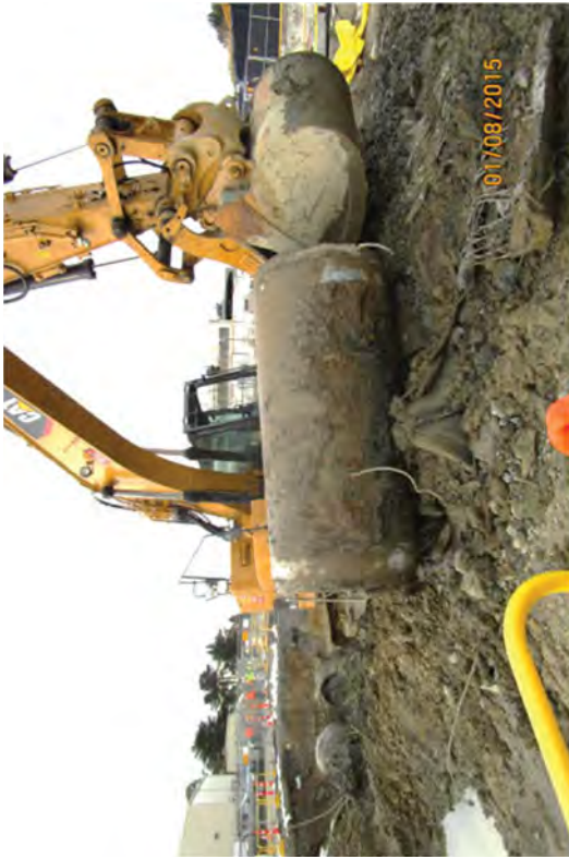
A section of cooling water pipe that has been sized to fit inside an intermodal.
