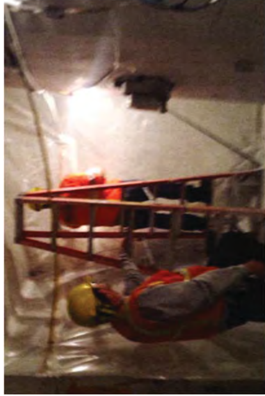
An enclosure was installed around the guard pipe because it was identified as ACM.
