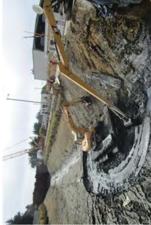
The excavator was set on top of mats to spread the mud and drying canal silt.
