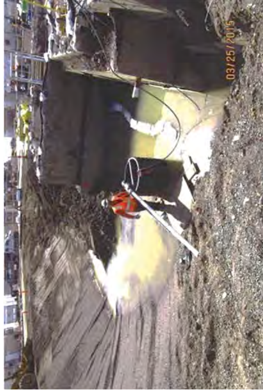
Installing a pump in the drainage sump to ready the area for the TB below grade removal.
