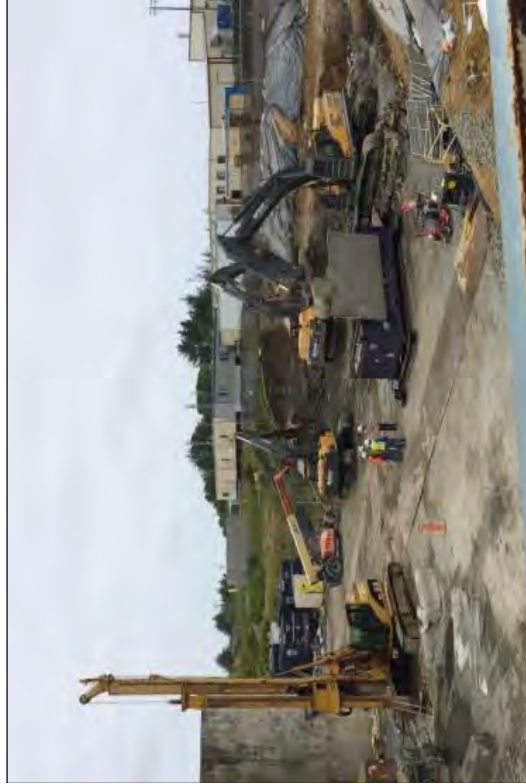
Heavy equipment in the North Yard must be coordinated to safely load IM's, demolish the LRWB concrete, and install the CSM wall.
