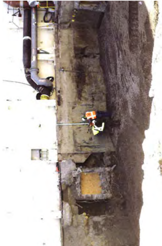
Surveyors painting marks at the necessary intervals for compaction testing to prepare the area for backfilling.
