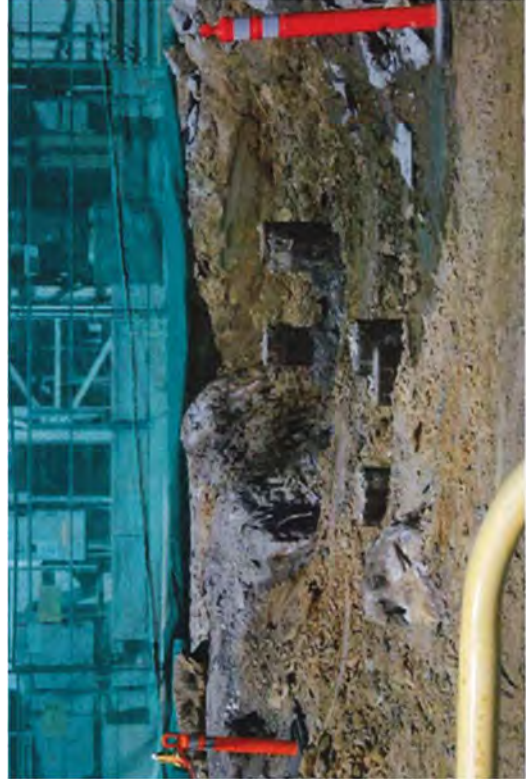
The view facing east of wooden pilings that were exposed while excavating lead-containing soils.
