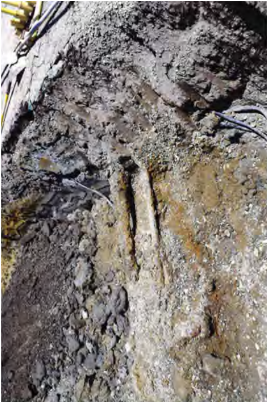
Crewmembers exposing two contaminated lines. A 4-inch drain line from the LRW can be seen along with an abandoned 2-inch radwaste line.
