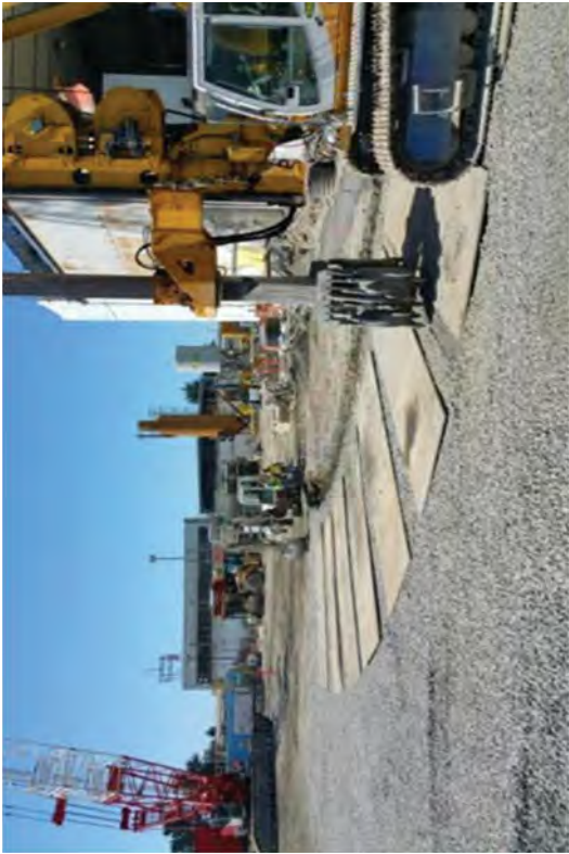
Plates are laid out to support the BG-40 while it installs the final panels.
