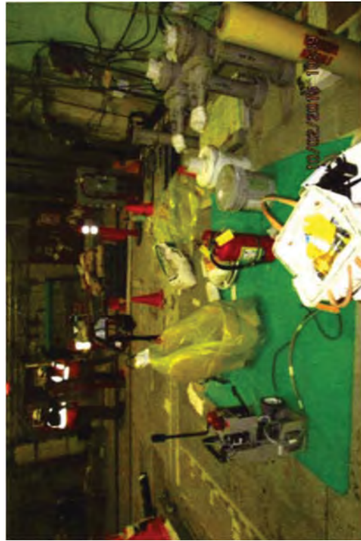
The last miscellaneous items removed from the underground facilities prepped to be removed from the RFB.
