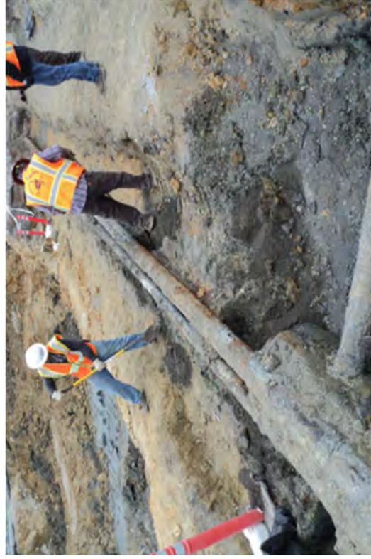
A crew excavating beneath exposed piping so that it can be cut.
