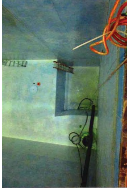
The sump pit in the SFP required additional characterization because it had held highly contaminated waste.
