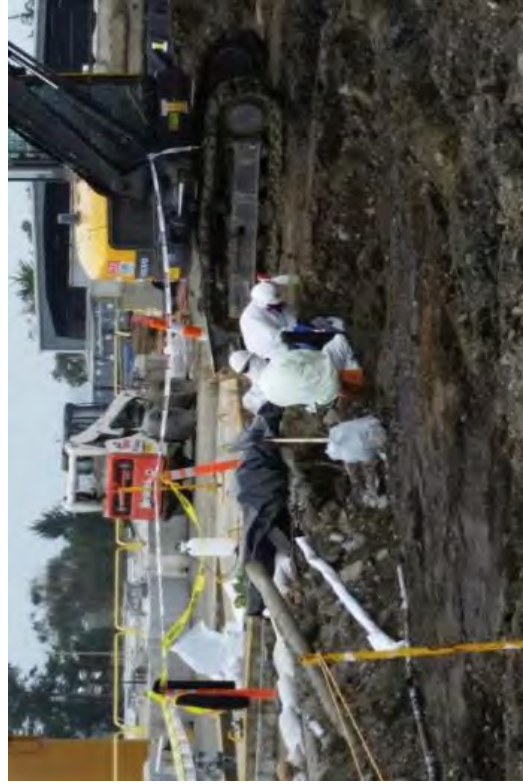
Removing ACM pipe that was the upright section of fire line going to the LLRW Building.
