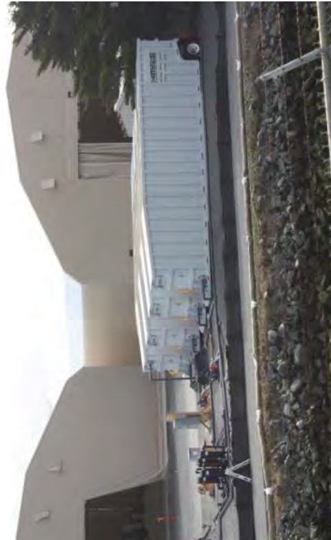
Pretreatment system installation to GWTS.
