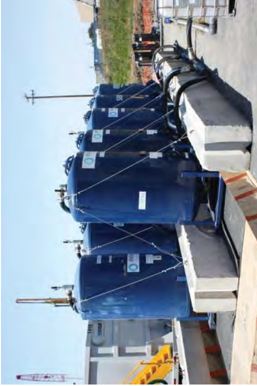
New carbon filters for the GWTS installed in July 2015.
