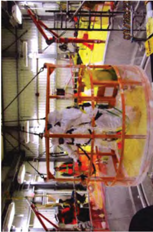
A crew in the man-basket descending into the drywell. The basket and associated rigging was inspected by engineering every workday.
