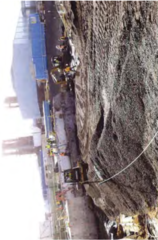
Creating a ramp so that the lower flat areas could be compacted.
