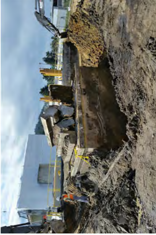
Exposing ACM piping. The HLV is seen with a pile of old rail footings on its lid.
