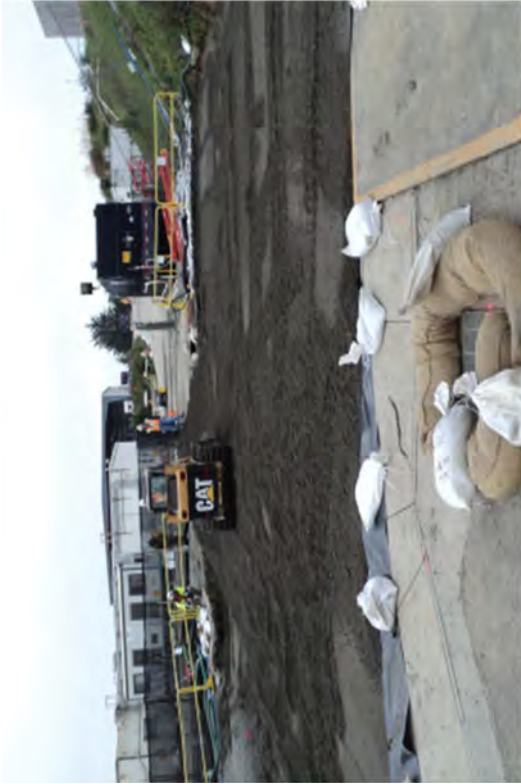
The top 12" inches of backfill placed for this portion of North Yard.
