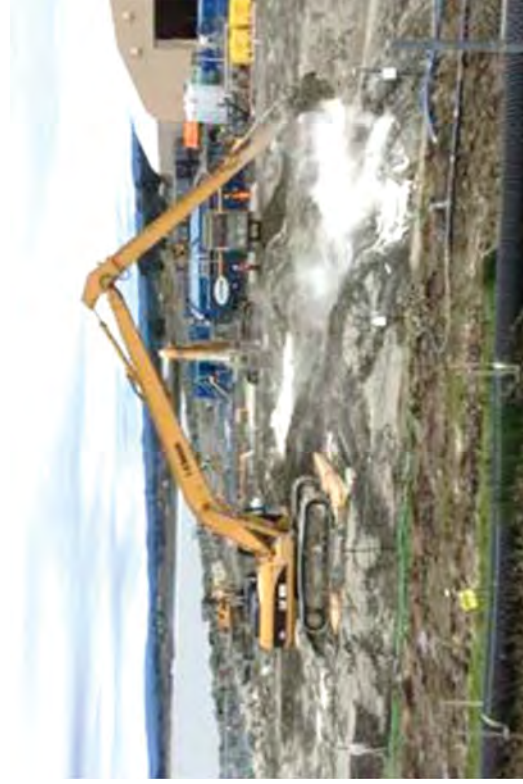
Mixing pelletized lime with CSM wall soils with a long reach excavator in the Discharge Canal.
