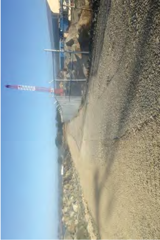
A view of the restored Coastal Trail at north end of canal after all Discharge Canal work was completed.
