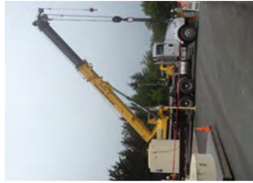
Relocating one SEC shield from the North yard RCA to the count room parking lot.
