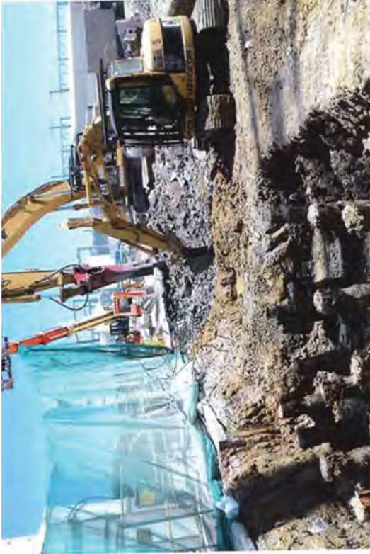
Demolishing and excavating on the eastern edge of the TB foundation footprint.
