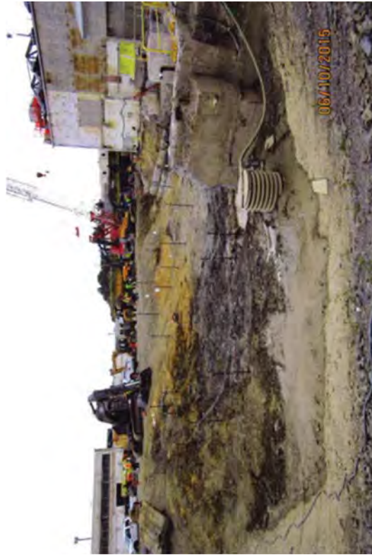
RP techs performing the FSS on the central sections of the TB excavation.
