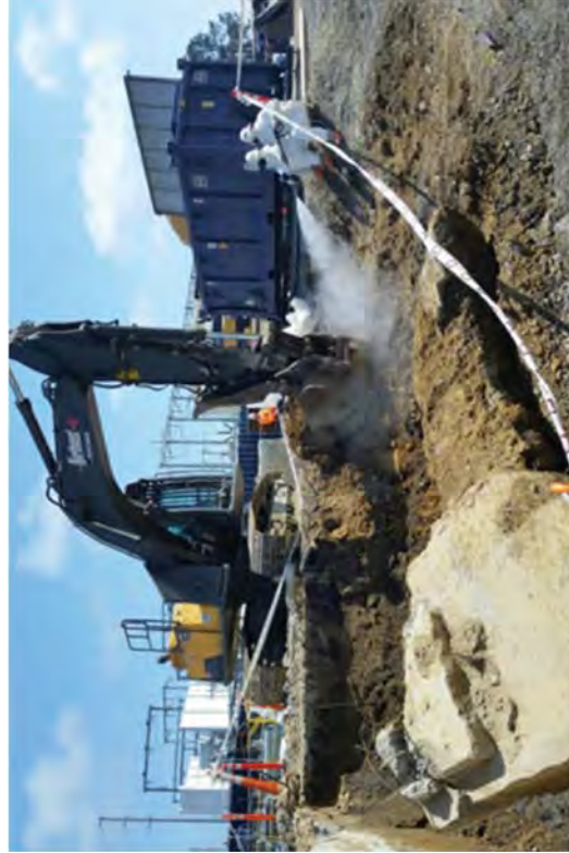
Loading out ACM required stringent controls to ensure the safety of workers.
