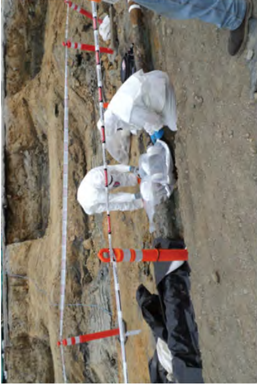
An ACM crew wrapping a glove bag over a 6 inch pipe to remove mastic tape.
