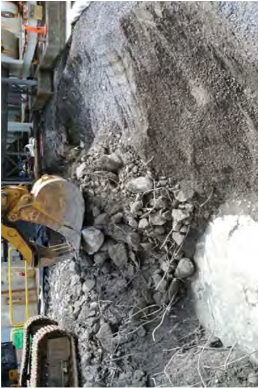
Demolishing and excavating SAS below-grade structures. The excavations were dewatered when it was necessary.
