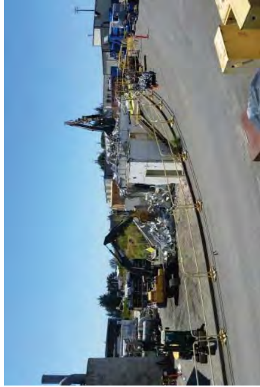
The LRWB steel structure completely down. The excavators are being used to reduce the size of debris so it will fit into intermodal containers.
