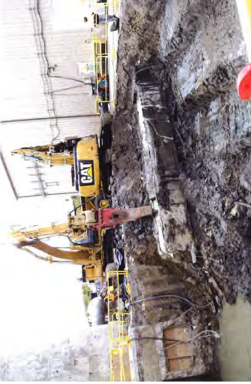
An excavator with a hammer being used to demolish the LRW tunnel floor.
