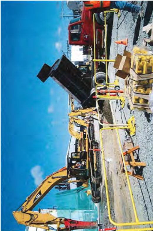
Breaking up a 6 foot thick slab with a hydraulic hammer. Rock has been laid down as a base for crane mats.
