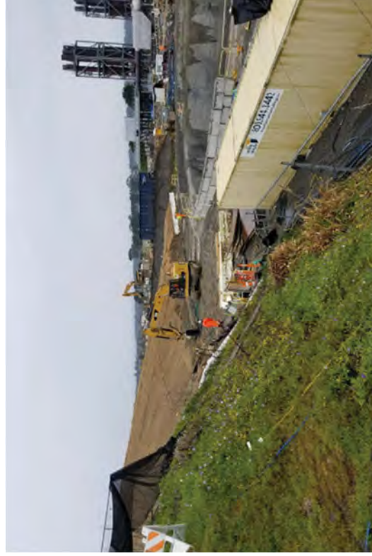
Preparing to transport soils stored in the upper yard for use as backfill material in the Caisson excavation.
