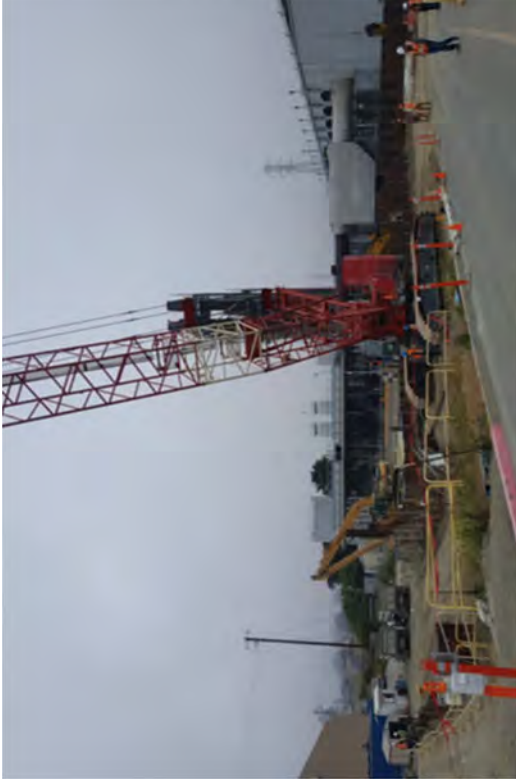
A 275 ton crane that was mobilized to remove sheet pile from Area D.
