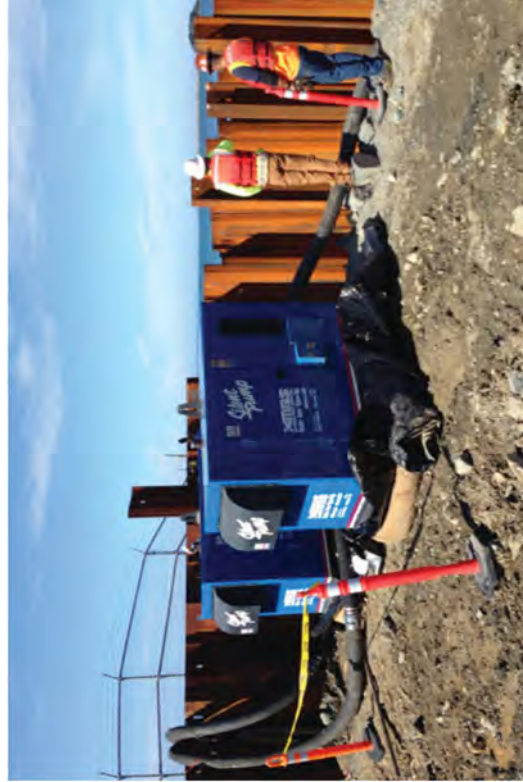
The canal's sheet pile wall suffered a substantial amount of damage during storms in 2014. Strong waves flexed and shifted the piles, which created several large leaks. Two diesel powered pumps operating at roughly 1600 gallons per minute were barely able to keep inflow from accumulating.
