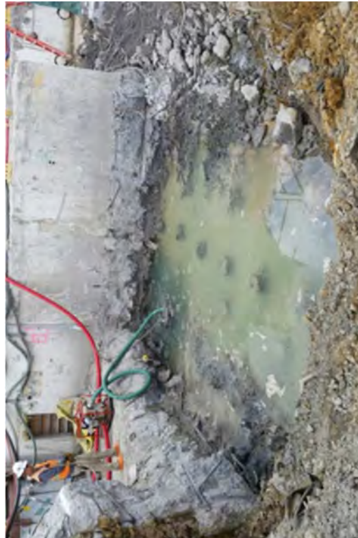
Dewatering the excavation. Wooden pilings can be seen just below the surface of the water.
