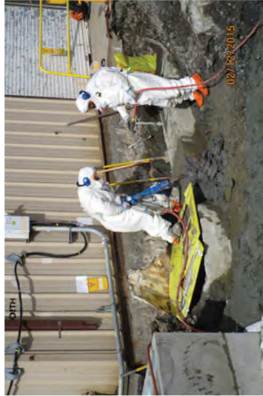
Demolishing the electrical duct run. The crew is dressed out in PPE due to contaminants and transite pipe in the concrete.
