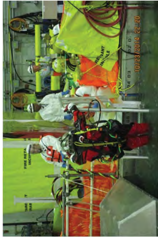
Divers entering the SFP to rig and prepare the liner for removal.
