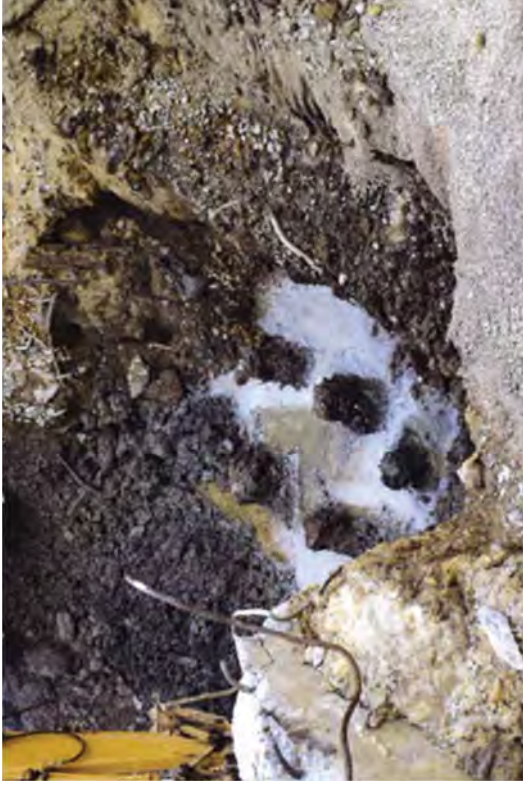
Exposing wooden pilings underneath the TB. A total of twelve wooden pilings were uncovered by the end of this work day.
