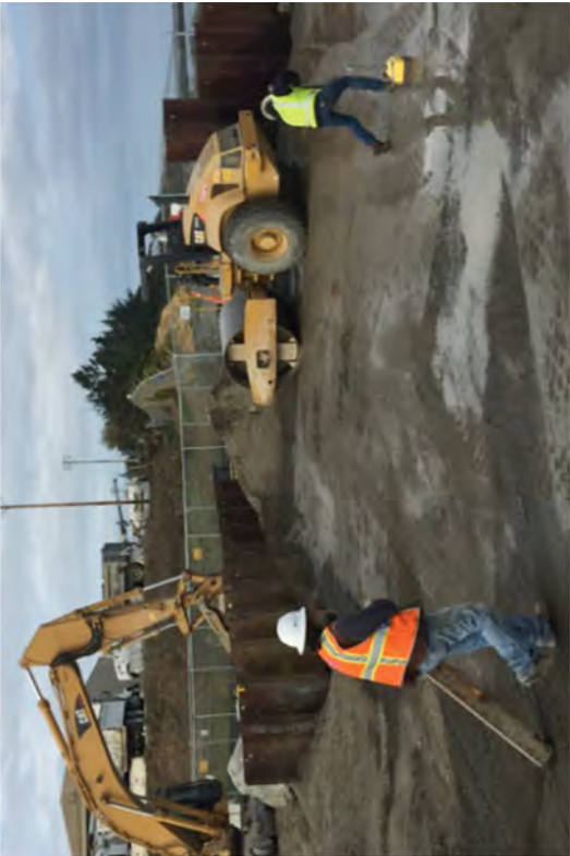
Performing compaction tests before laying down mats for the crane used to remove sheet piles.
