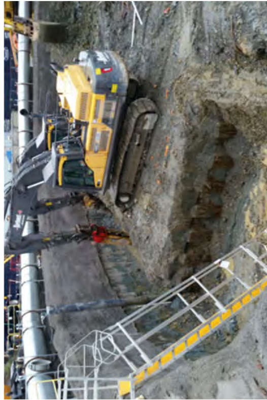
Exposing the east wall and preparing to bore the CSM wall to obtain a core sample.
