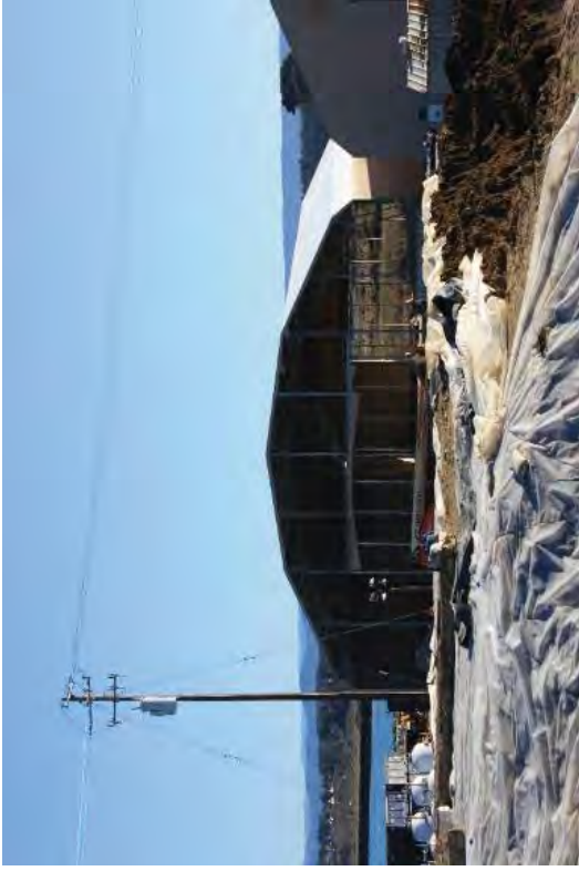
SMF Tent 2 Fabric partially removed.
