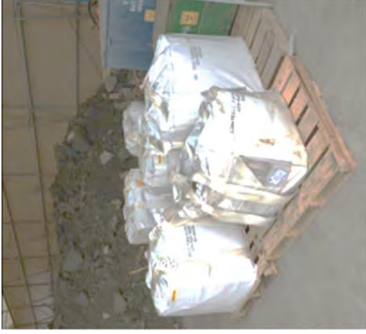
Bags of debris generated from cleaning out the intake structure.
