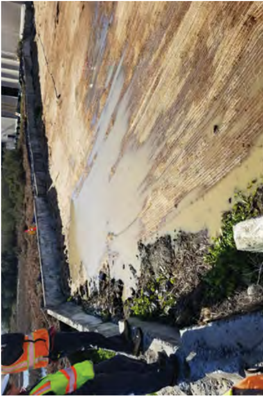
Storm whater that needed to be removed.
