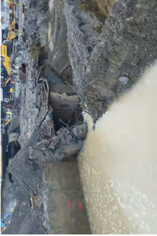
Flooding from storm water in the Caisson.
