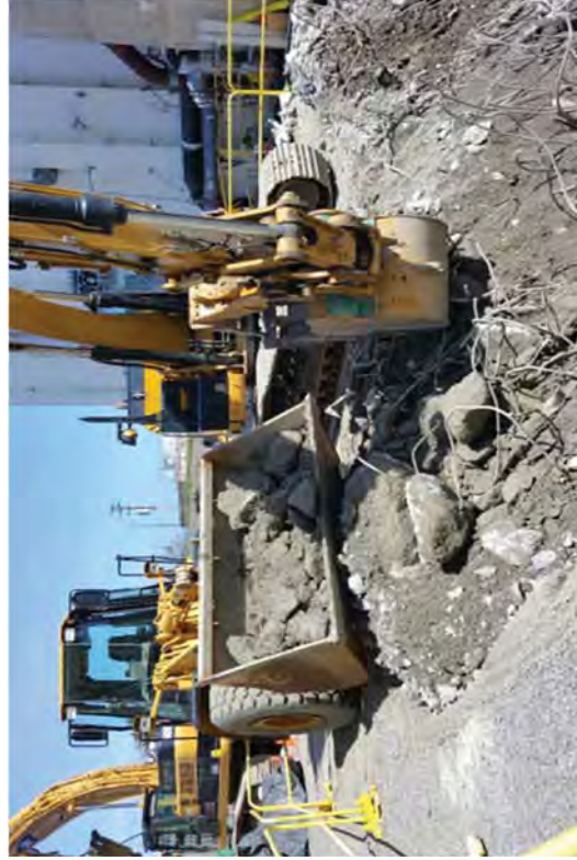
Placing debris directly into a bucket loader which then took the debris to a waste intermodal.
