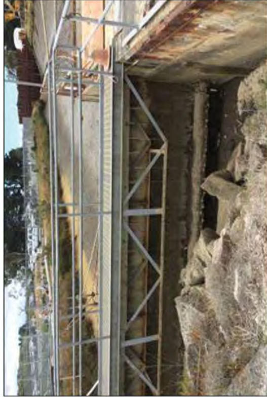
After dewatering the Intake Canal, wooden pilings were unexpectedly found to be incorporated into the Intake Structure. The demolition plans were modified to accommodate the treated wood waste.
