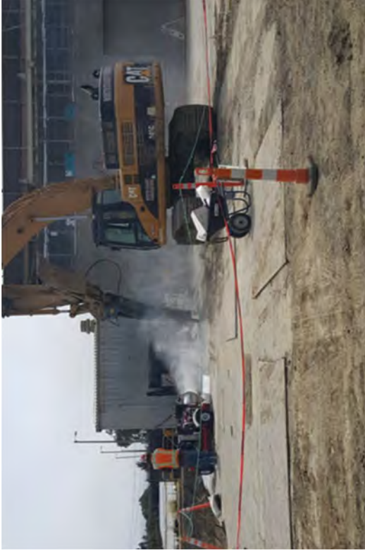
Demolishing the Unit 1 concrete pad to reach underground commodities and Circulating Water Lines.
