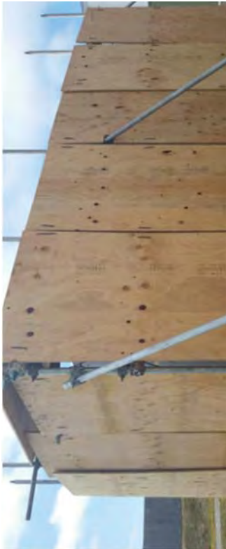
Protection installed around "LC-24", which was an electrical load center. This load center supplied power for demolition activities
