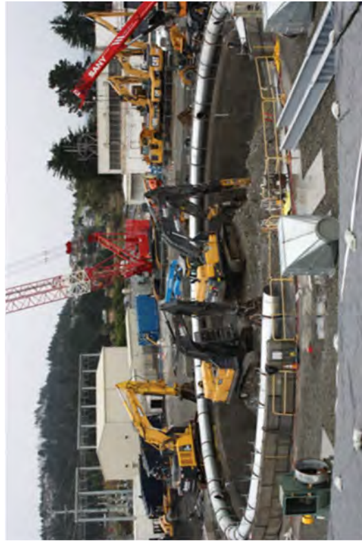
Excavating the center of the Caisson and filling the suppression chamber with excavated soils and debris.
