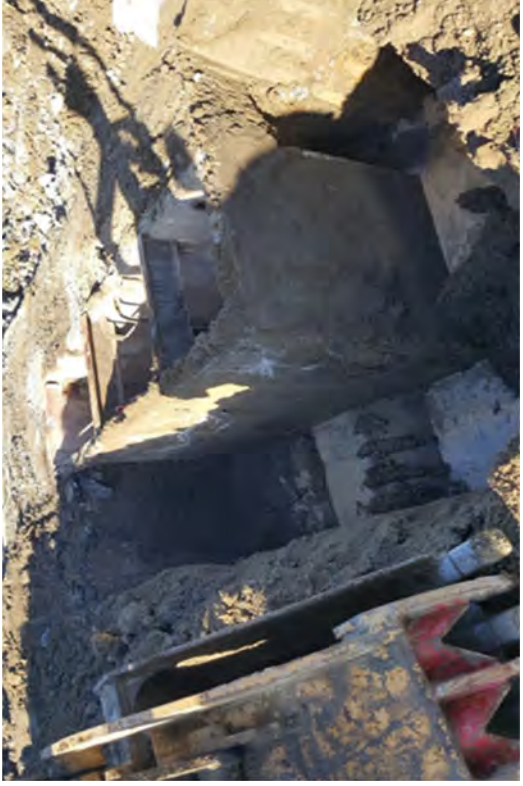
The sampling vault next to Building 5 alongside Circulating Water lines to the Unit 1 inlet and discharge.
