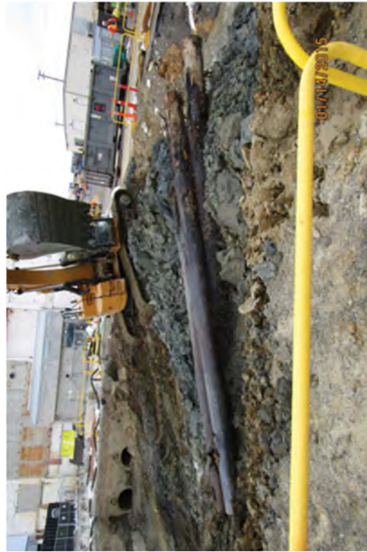
Three wooden pilings after being extracted. They each measured 15 to 20 feet long.
