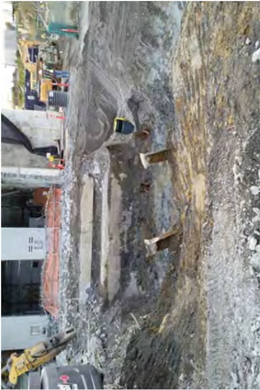
The excavation to remove H-Piles, wooden pilings, and the Off Gas Tunnel.
