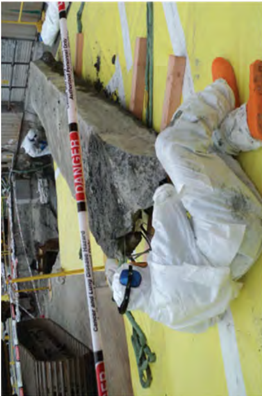
Injecting embedded pipes with two-two part epoxy expanding foam as they rest atop supports. Pipes left in place within the raceway were also injected.
