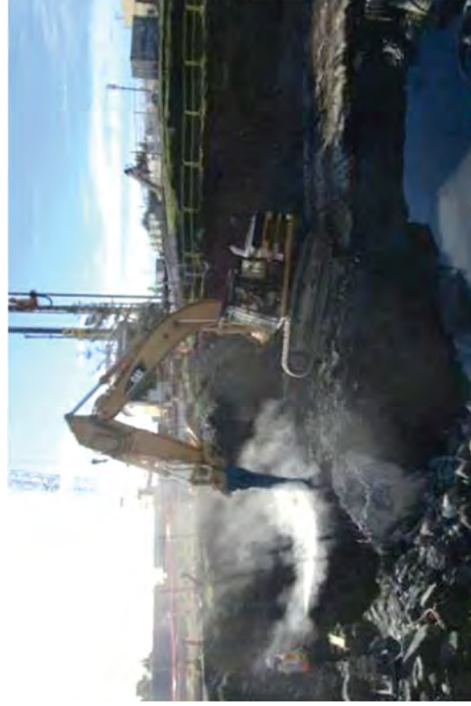
Water misting was used during concrete demolition to control airborne silica dust.
