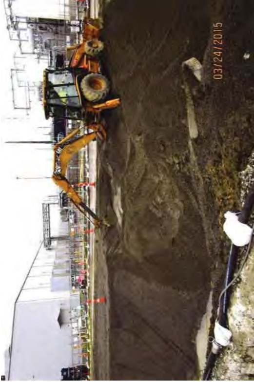
The HMS excavation after the Circulating Water Pipe was cutoff with CLSM.
