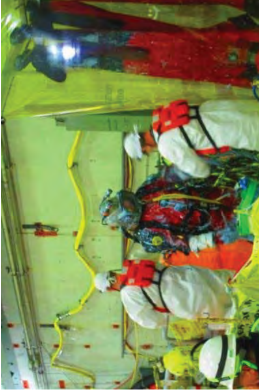
A second diver preparing to enter the SFP and continue cutting the liner. The divers only worked underwater in short shifts to decrease their risk and radiological exposure levels.
