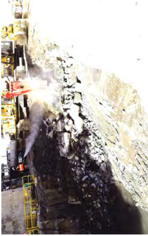
Using an excavator equipped with a hammer along with a second excavator to create and then remove debris.
