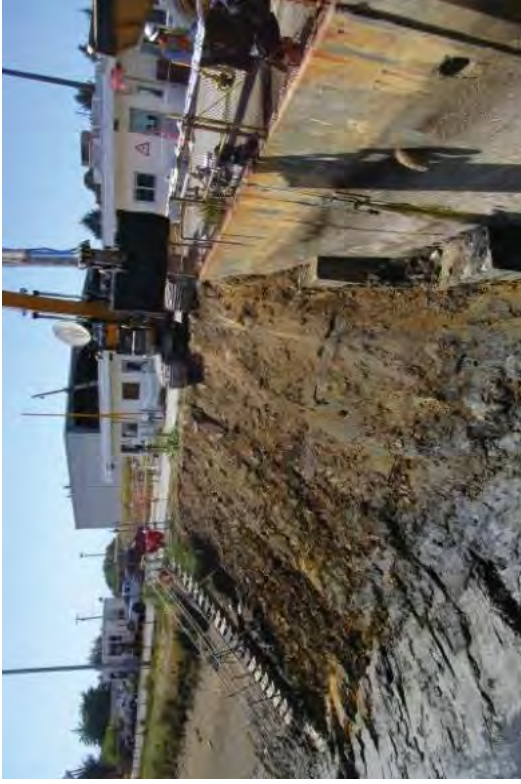
Removing soils from in front of the Intake Structure and spreading mud to dry.
