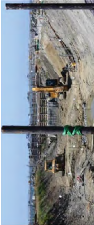
The North Discharge Canal before it was used to stockpile CSM spoils.
