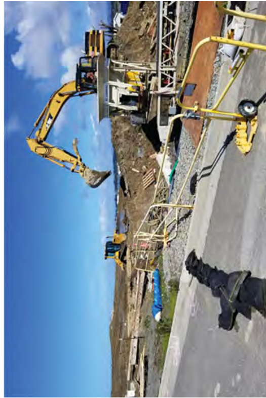
An operator loading reuse soils into the hopper that were transported from storage in the Discharge Canal.
