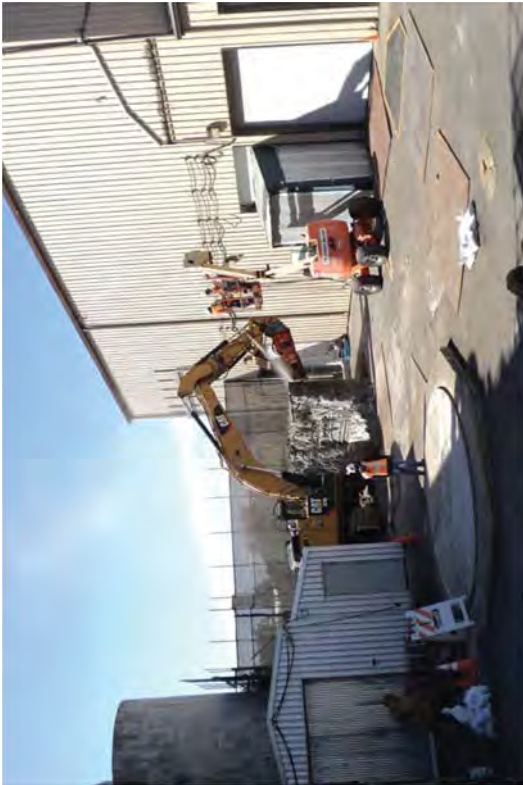
Using an excavator to hammer the north face of the north wall.
