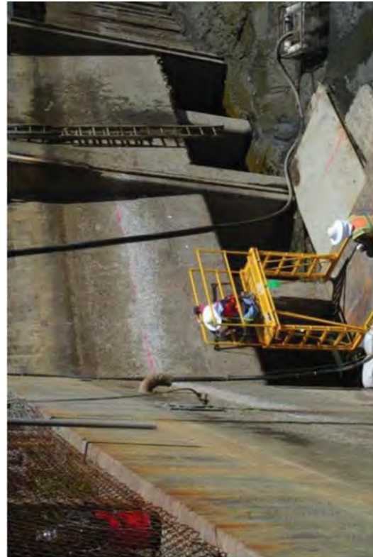
Concrete surfaces had to be smooth before RP and FSS could survey them.
