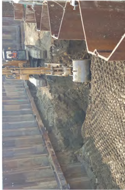
After removing soil and pipe from Area D the sheet piles must be removed and the area finished to grade.
