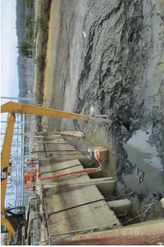
A long reach excavator moving canal silt from in front of the intake.
