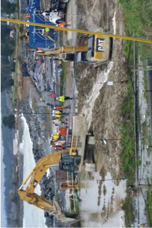
Operators removing excavators from the canal because of the high water levels.
