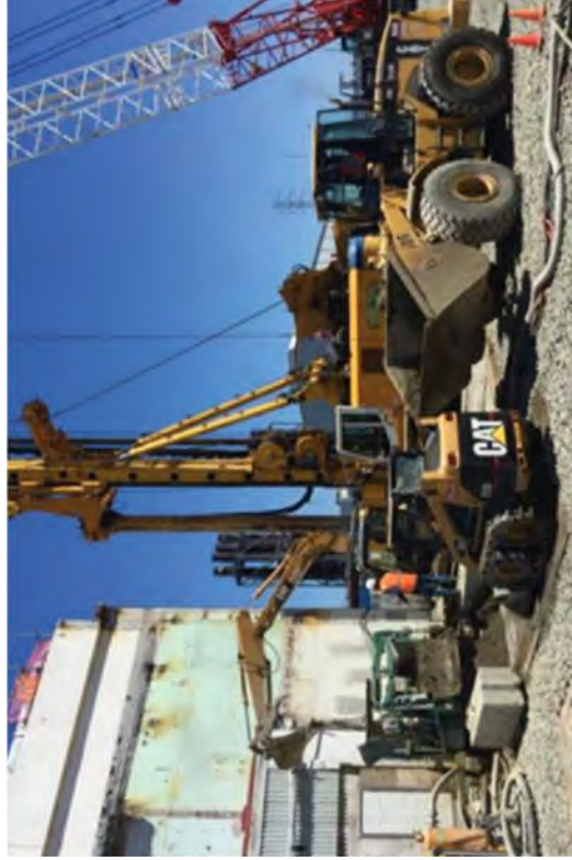
During de-clay operations, a front loader is used loading material into a truck which then transports it to the canal.
