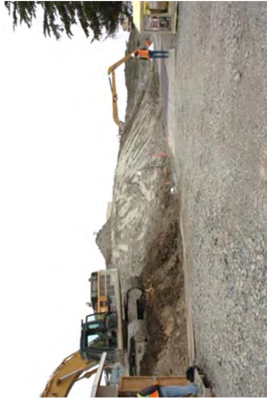
Looking south at excavators being used to manage the stockpile of CSM spoils in the Discharge Canal.
