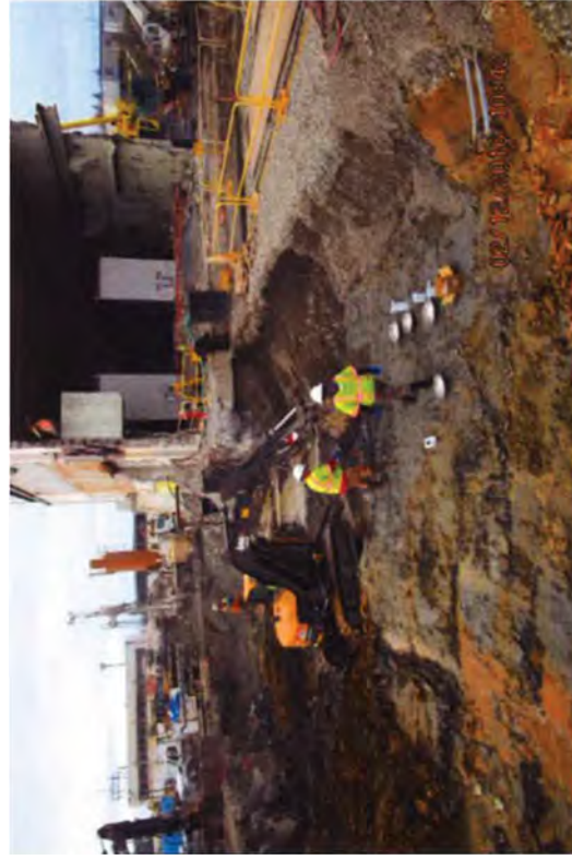
Environmental technicians collecting soil samples while wooden pilings are being removed in the background.
