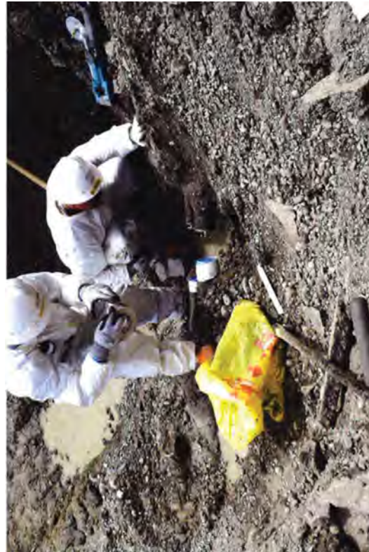
Plugging the ends of the 2-inch and 4-inch pipes that stay in the ground with two-part epoxy expanding foam. The pipes that will be disposed of are taped. The pipes left in the ground is outside the limits of the excavation and will be removed later.
