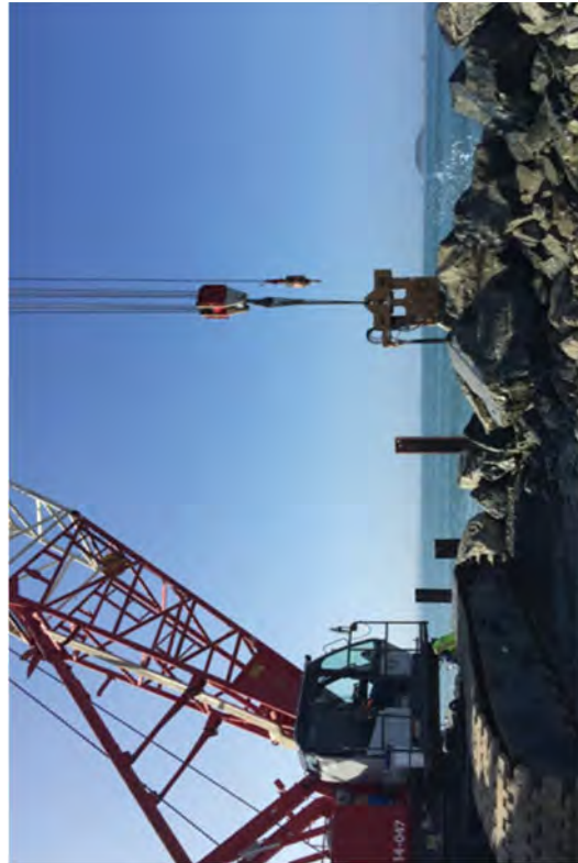
Removing the remaining sheet pile from Humboldt Bay at the Discharge Canal.
