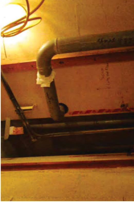
A Pipe in the valve gallery that has been abated of lead.
