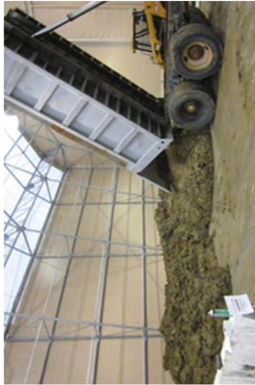
Transferring excavated Unit 2 soil with low or no radioactivity to the SMF for potential re-use.
