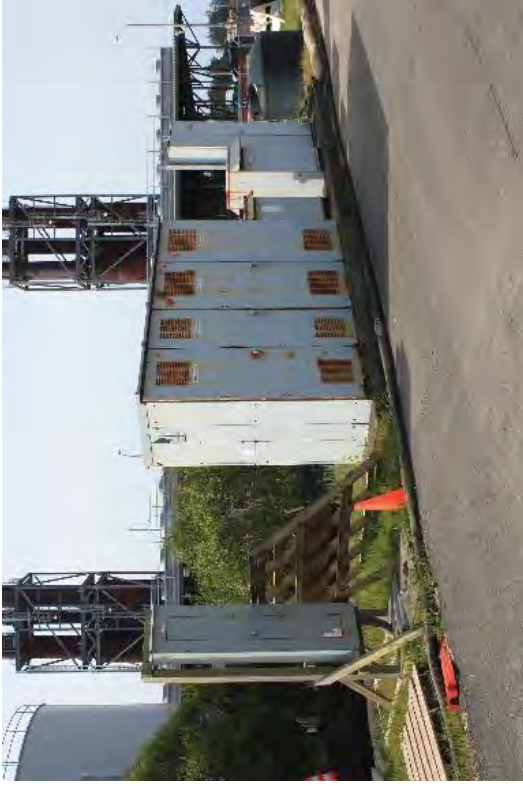
Load Center 5 (LC-50)
