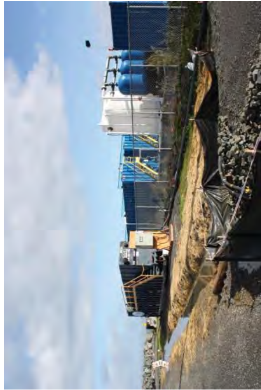
An additional GWTS tank installed for the Discharge Canal.
