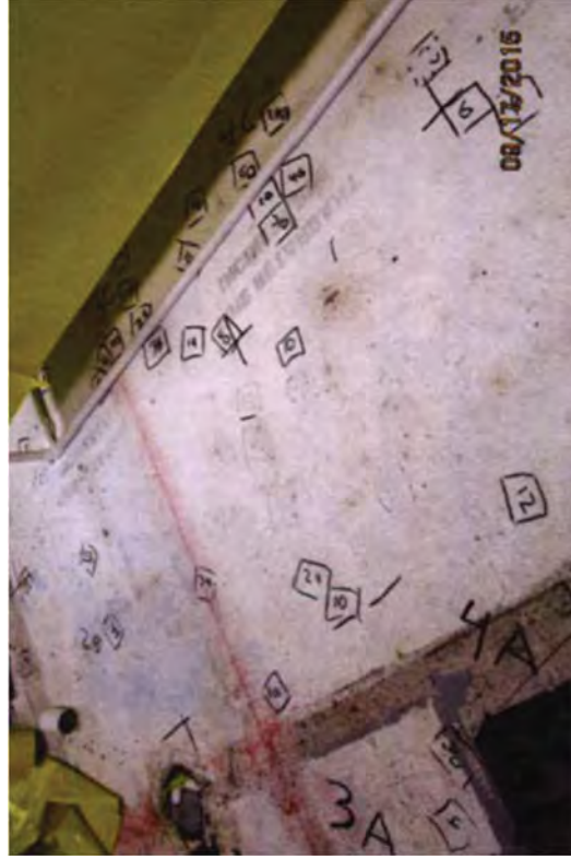
Areas of contamination marked on the RCF flooring.
