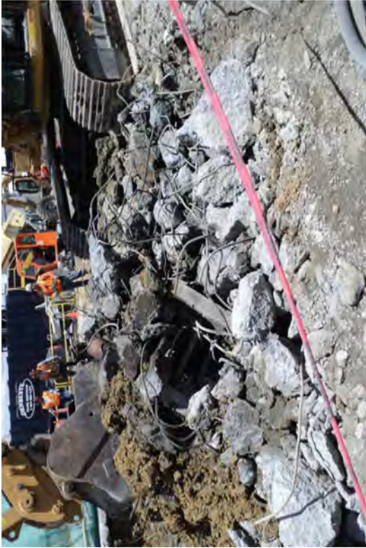
Debris from Unit 2 Boiler Blow-off Drum pit.
