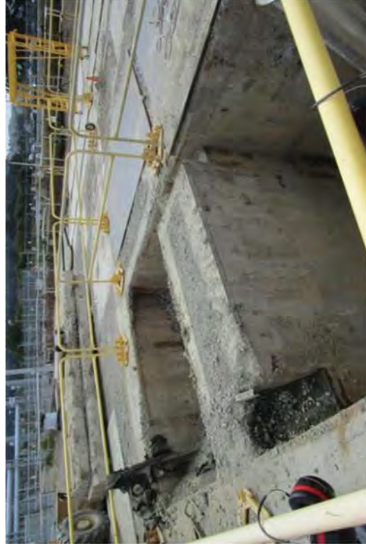
Cells were sectioned off with safety railing after being uncovered.
