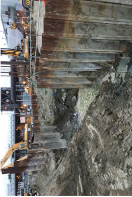
The headwall removed and showing evidence of some water intrusion.
