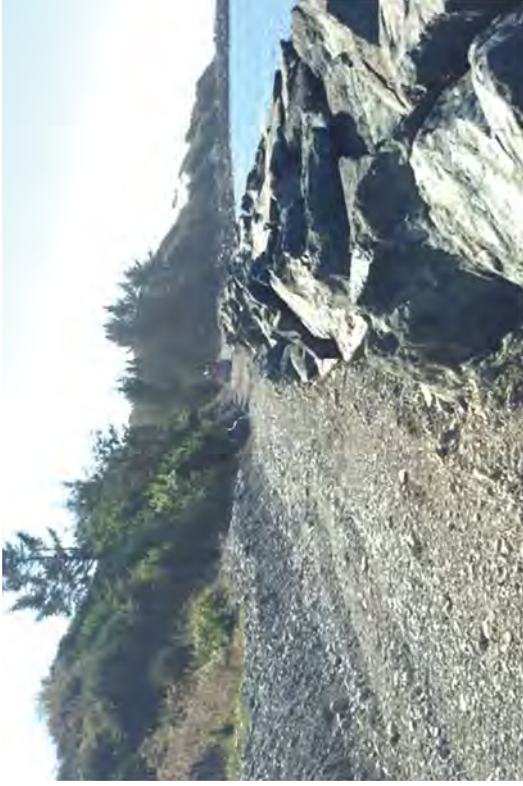
A small front loader spreading and leveling rock for the Coastal Trail.
