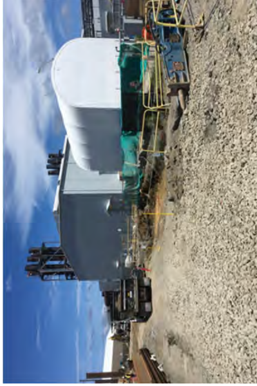
Beginning to backfill after FSS of the OWS raceway excavation was completed.
