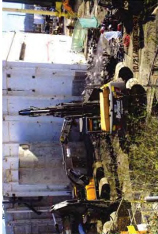
Size-reducing metal scrap debris and Demolishing concrete pads to backfill the area so that the CSM can be installed.
