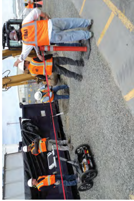
The initial dig into the Unit 2 slab south of the construction fence. Samples were taken at this time for environmental testing.
