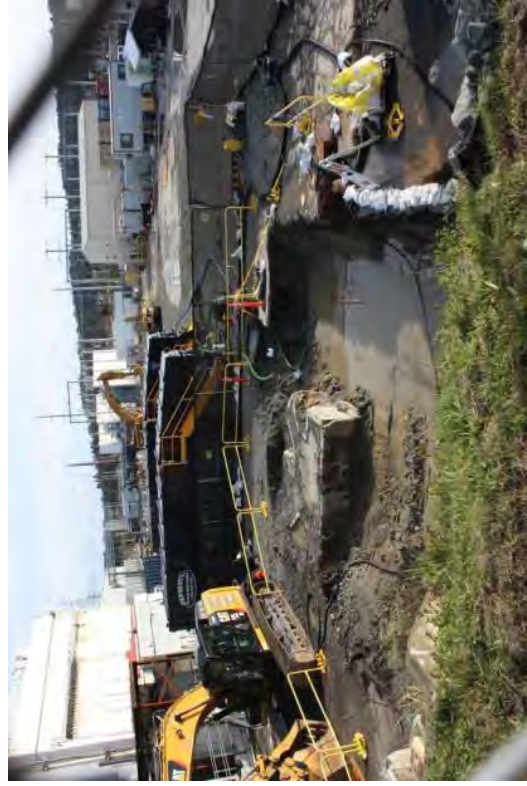
The Unit 1 demolition area with holding tanks for ground and storm water.
