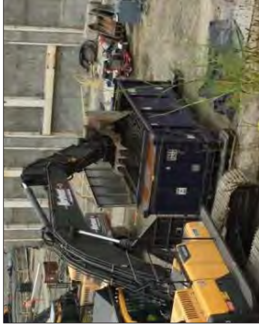
An Excavator moving rebar in an IM closer to its door for easier unloading at the disposal site. Other waste is positioned behind the rebar.
