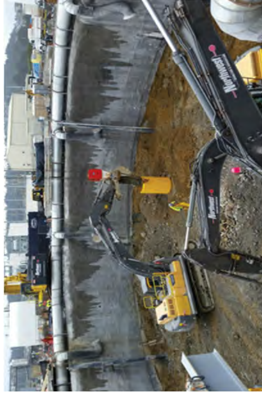
Using an excavator to load out material from the Caisson into a muck bucket.
