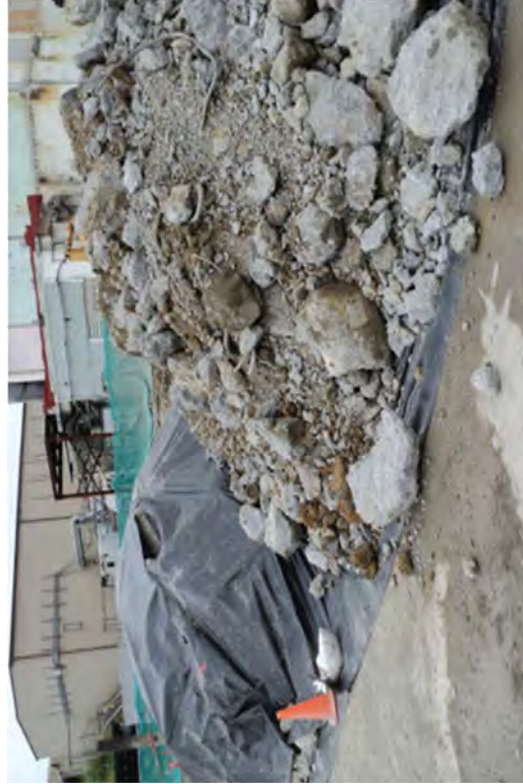
Concrete stockpiles were segregated corresponding to the results of sampling and testing by RP staff.
