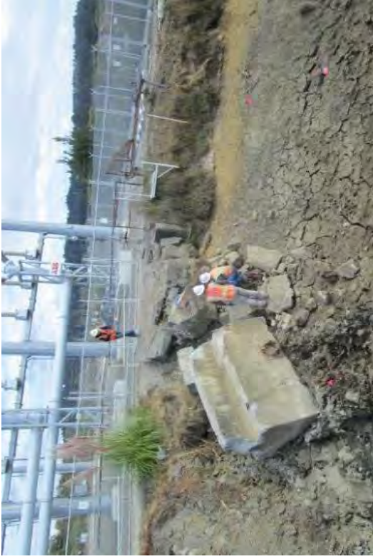
Rubble from earlier days, next to where the small pedestrian walkway bridge was removed.
