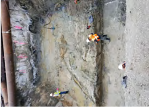
The FSS activities were ongoing. For the instrumentation to work properly, any surface water could be no deeper than 1 inch.
