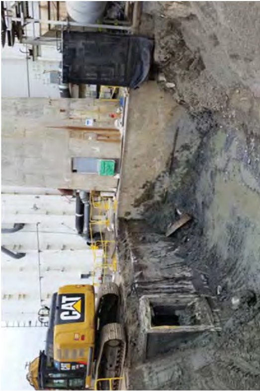
The Off-gas tunnel can be seen on the left of the SAS excavation. The stack is on the immediate edge of the SAS. On the right is the MPEF which is surrounded with protective barriers.
