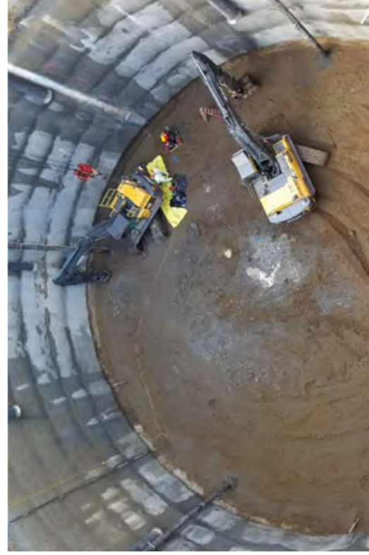
Beginning to decontaminate and remove equipment. At the end of 2017 the Caisson structure was fully removed.
