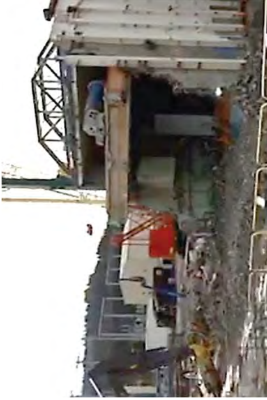
Arranging rigging to make the final pull to remove the crane rails.
