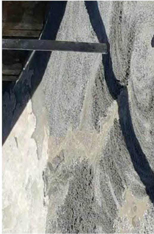
Pouring CLSM to reduce ground water inflow and allow for soil compaction.
