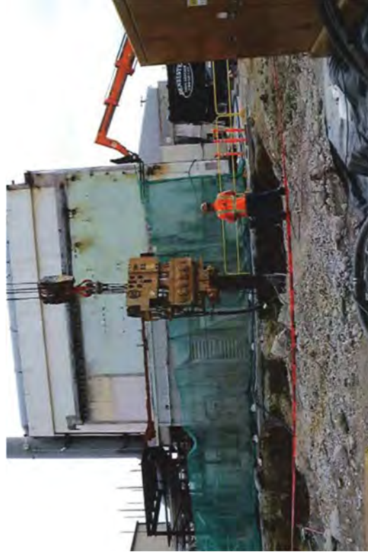
A vibratory hammer forcing a pipe sleeve over a wooden piling to free it by breaking the suction created by the dense clay layer.
