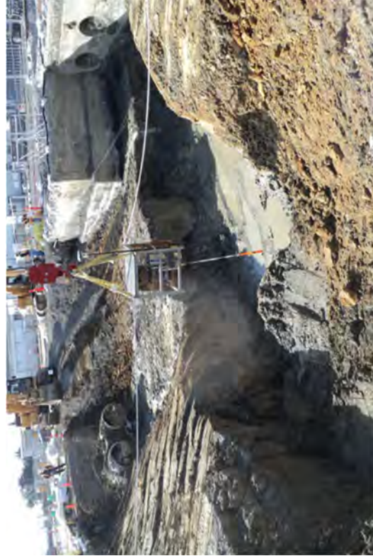
FSS suspends the ISOCSS over an area previously occupied by deep discharge water line.
