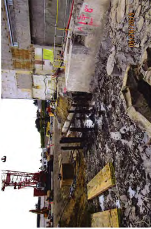
After they are loosened, the piles can be extracted by conventional means.
