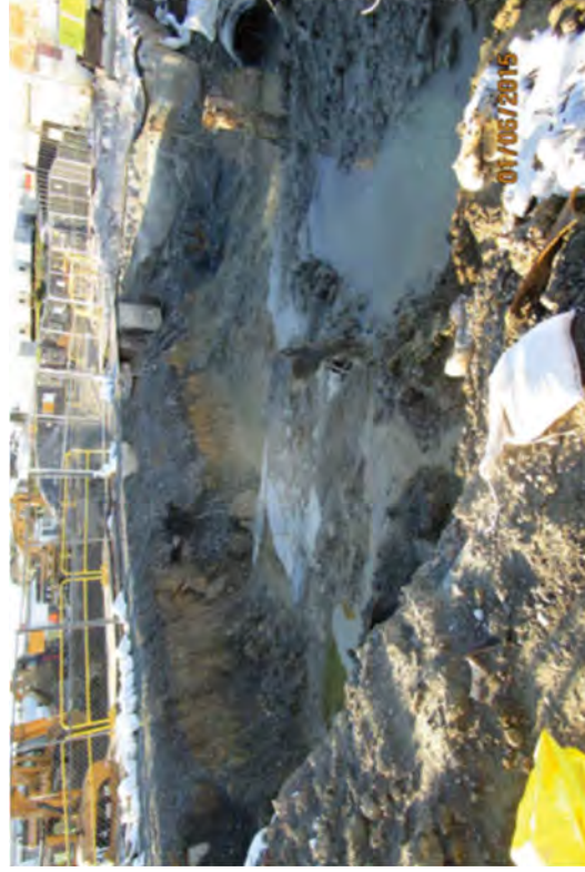
An excavation showing a 39" inch cooling water inlet pipe along its west side.
