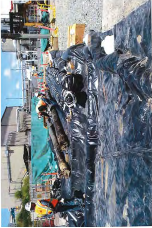
RP technicians reviewing and taking samples in the wooden piling laydown area.
