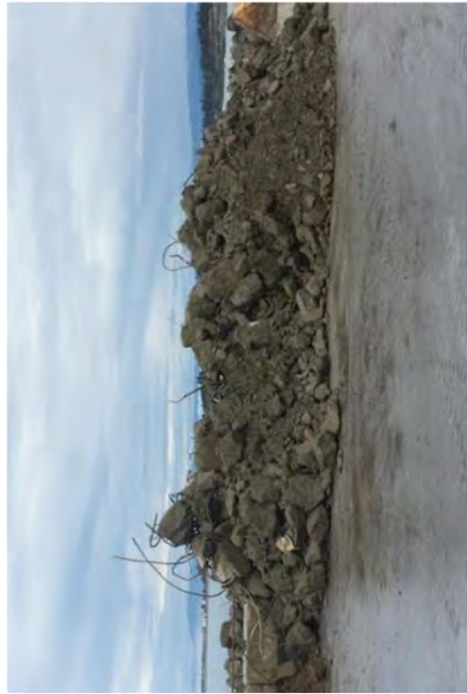
Intake Canal structure rubble.
