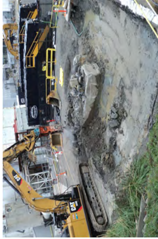
Concrete broken in and around the vault at west North Yard.
