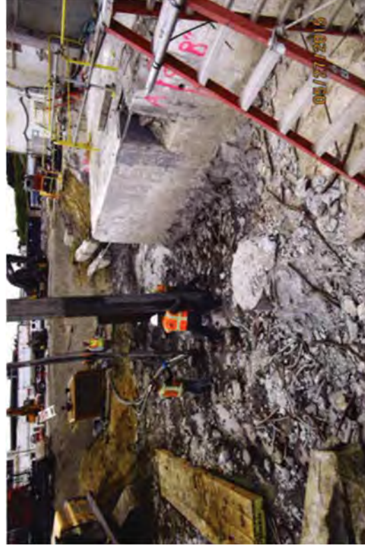
Pumping CLSM into the holes left after the wooden pilings were extracted.
