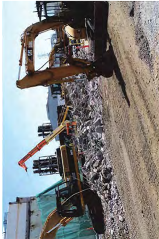
Loading unit 2 slab debris while the ground is prepared for crane mats.
