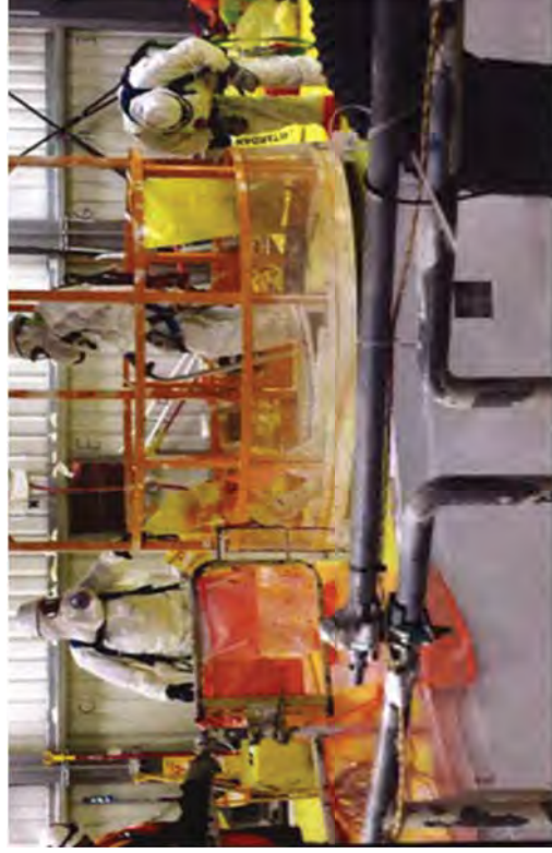
This is the pipe cutting crew starting the removal process. They descended into the drywell in a man-basket, cut small bore pipe, and were then lifted back up to the +12 EL RFB floor with segments of pipe. At the top, they handed the segments of pipe to RP technicians so that they could be surveyed.
