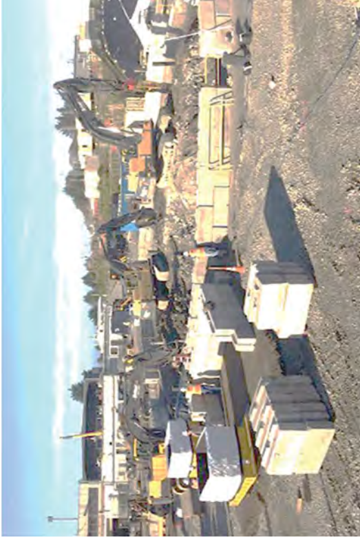
The Caisson excavation was configured so that soft sided IP-1 waste bags could be loaded directly from the work face.
