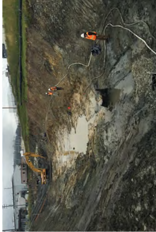
The crew kept the canal dewatered so that FSS could take place.
