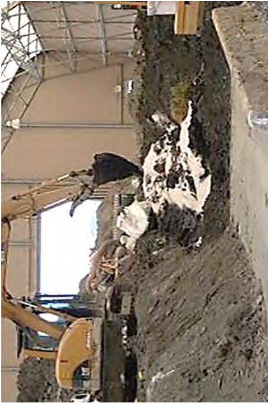
Soil from the Intake Canal. Lime was added to help stabilize the loose, wet material.
