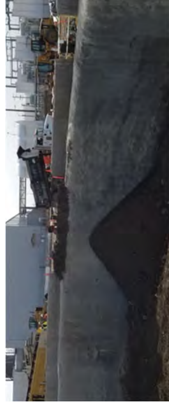
Backfilling the Caisson excavation with processed Concrete material after leveling soils inside.
