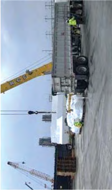
The crew preparing soft sided bags of soil for itemizing and loading to truck.
