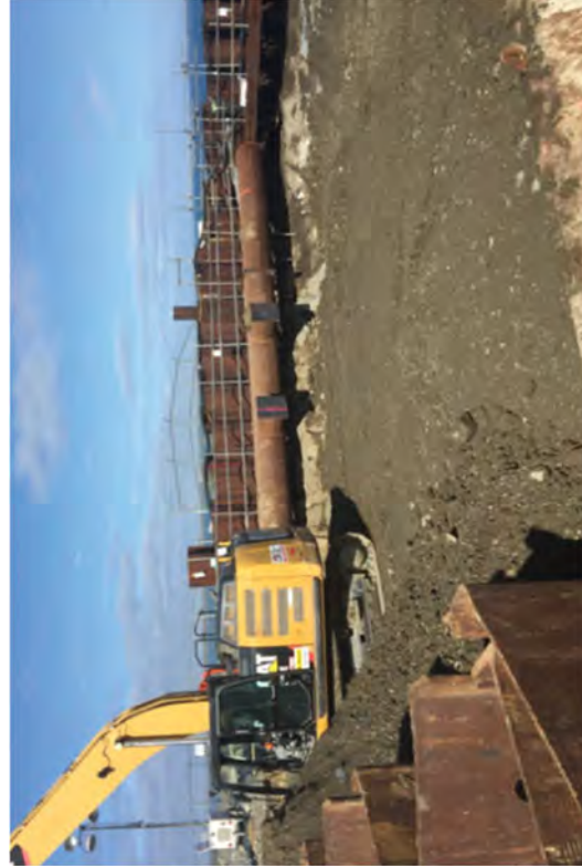
Continuing to backfill the Discharge Canal. The center water supports have been removed.
