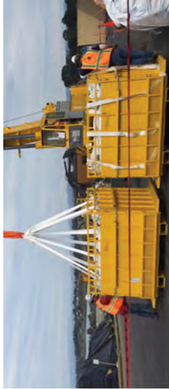
Using a 50 Ton Crane to unload bags of soil waste from metal frames.
