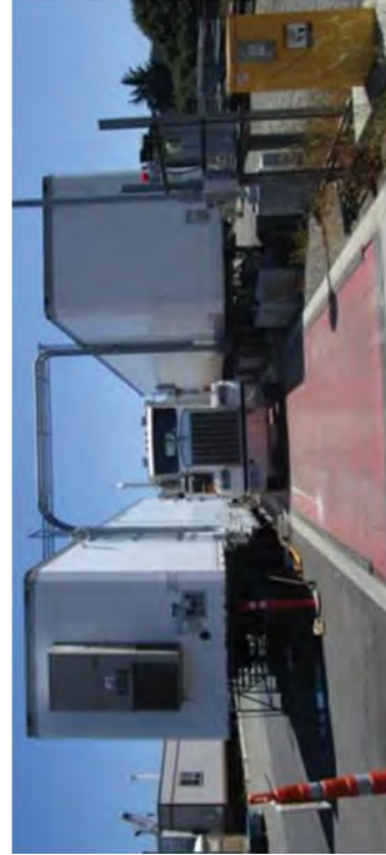
Scanning CSM Spoils with the GARDIAN before stockpiling them in the Canal to be re-used.
