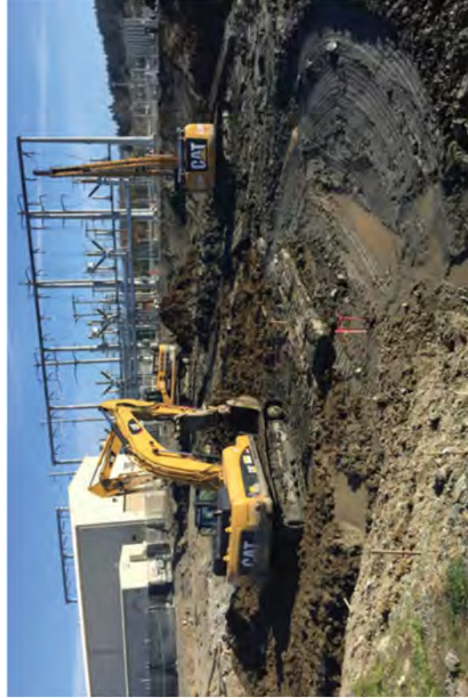
A crew using excavators to place fill at the east and north sides of intake.
