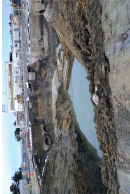
An excavation that needs to be dewatered. This was a typical accumulation for most mornings.
