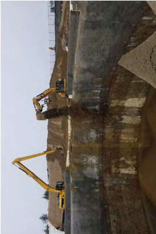
Beginning to backfill the Caisson excavation with reuse soils from the upper yard storage area.
