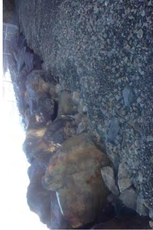
Waves during a storm pulled gravel away from the trail and back into Humboldt Bay. A plan was created to place a boundary of slightly larger rocks between the gravel trail and the larger riprap.
