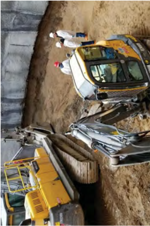
The Project Director and Deputy Director Inspecting the Caisson Tremie at the working surface.
