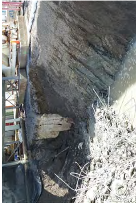
Sacrificial backfill was used to stabilize the West edge of the SAS excavation because hydraulic hammering on the foundation caused soil sloughing adjacent to the sheet piling.
