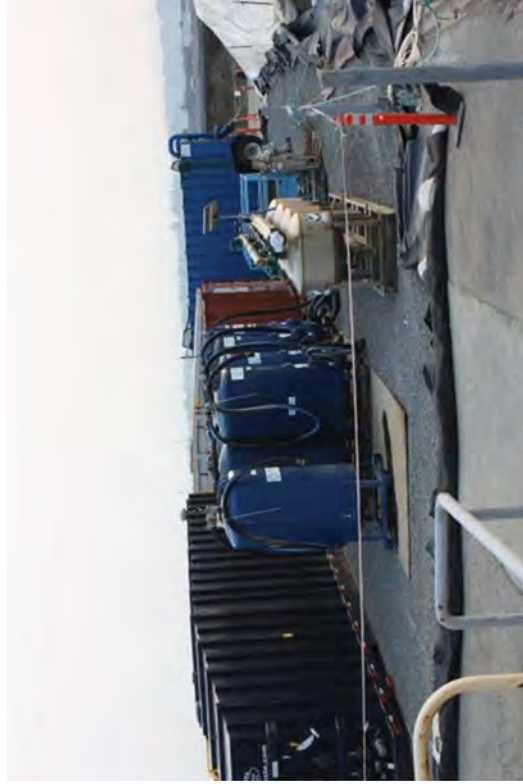
The GWTS 2 components installed inside berm retention area.
