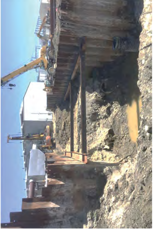
A water installed near the Discharge Canal.
