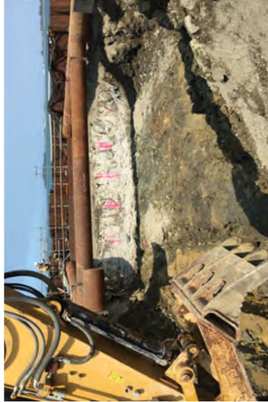
Looking north from sheet piles to where the four discharge pipes originate.
