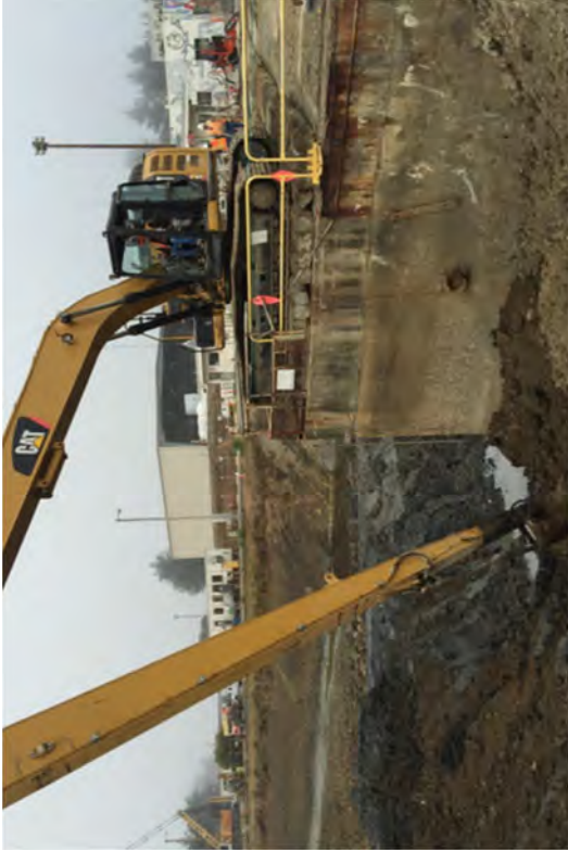
An excavator shaping the area near the Intake Structure before establishing the final grade.
