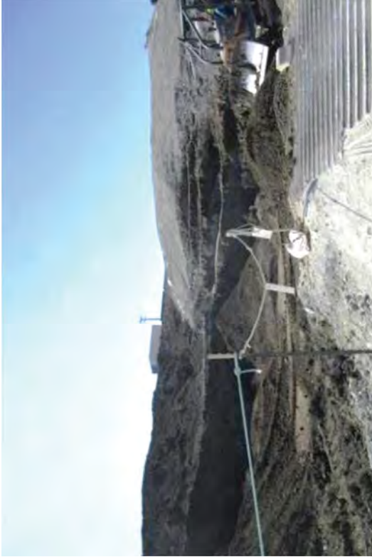
The area beyond the green rope has cleared FSS. Clean soils were loaded into trucks at this ramp.
