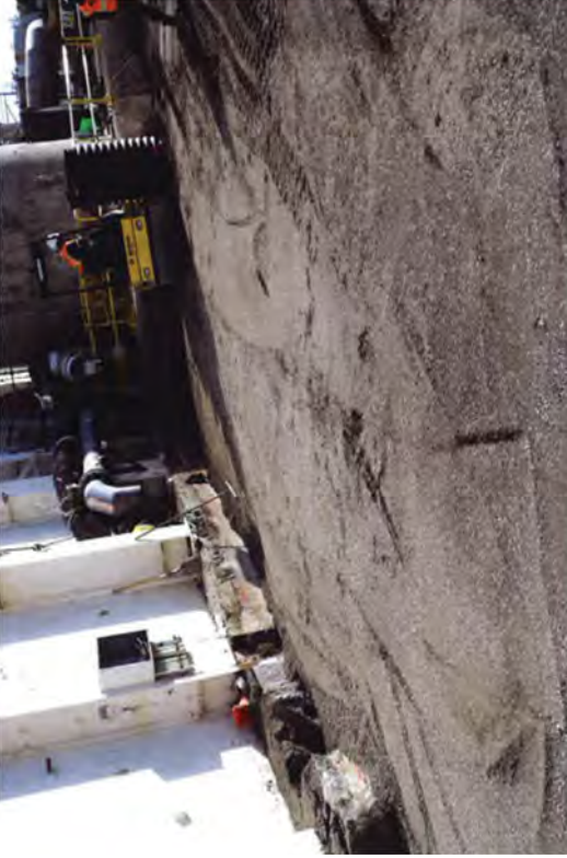
The crew compacts a 20 foot zone so that scaffold builders can wrap the RFB building for asbestos remediation.
