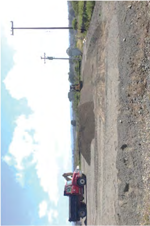
The foundations for the SMF tents were constructed at the former location of Trailer City, which had previously been the location of the Unit 1 and Unit 2 settling ponds.
