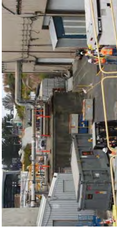
Preparing the SAS Building for demolition, including removal of ventilation and power running across the top of the building.
