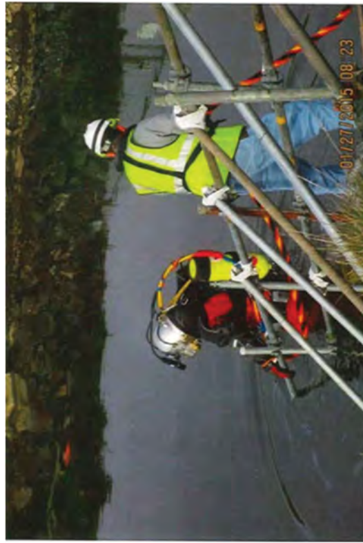
A diver entering the water to install the inflatable bladder inside of the Discharge Canal outlet.
