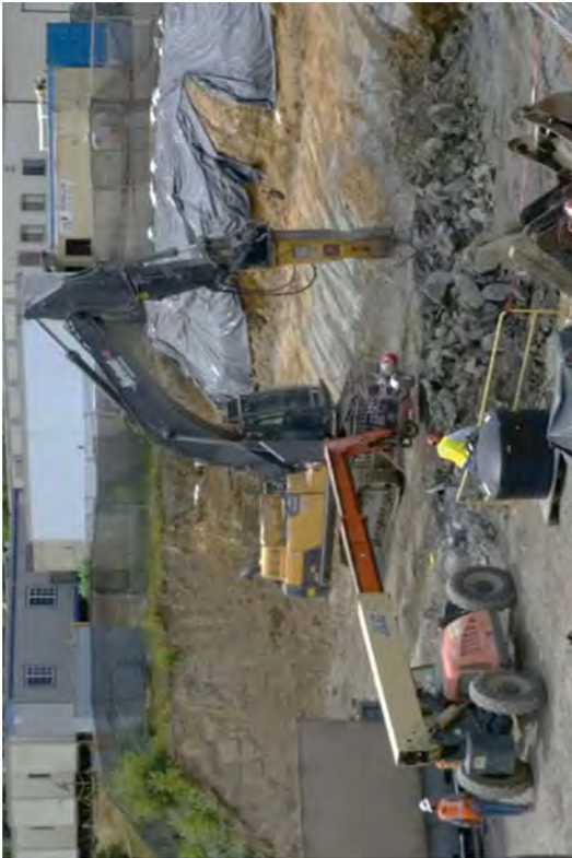
Demolishing and loading out the LRWB slab. The transition slope to the upper yard is covered in plastic sheeting.
