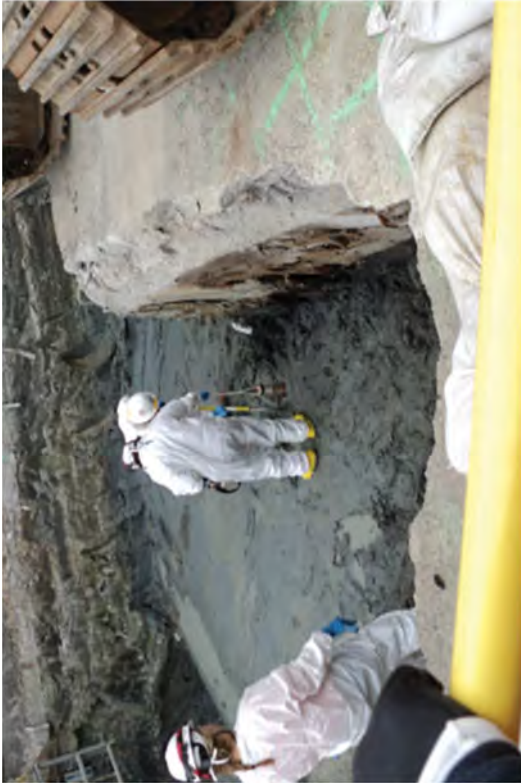
RP technicians scanning the excavation after deeper successive cuts. This area was known to have high radiological and heavy metal contamination.
