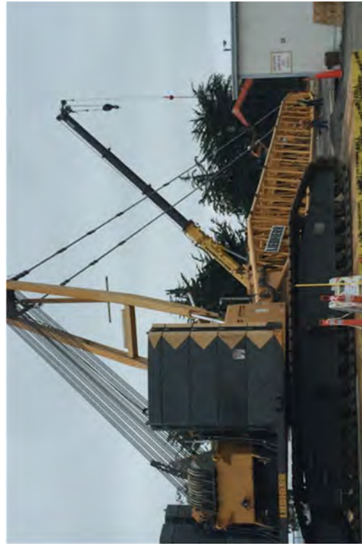
Assembling a 330-ton crane. Twenty trucks were needed to deliver its components.
