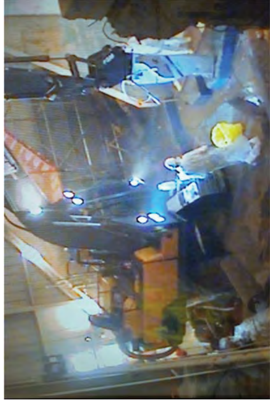
Decontaminating an excavator so that it could be removed from the building.
