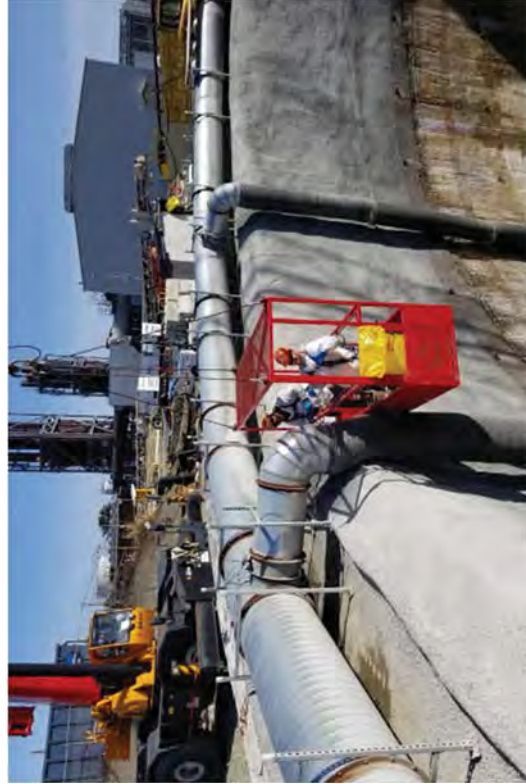
Man basket in use for Caisson work. Man baskets were only allowed and used with strict procedures and inspections.
