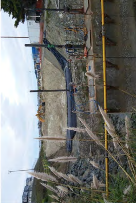
A bladder dam was installed on the South end of Discharge Canal to control water intrusion from the bay. Soil is stockpiled from the CSM installation behind the bladder dam.
