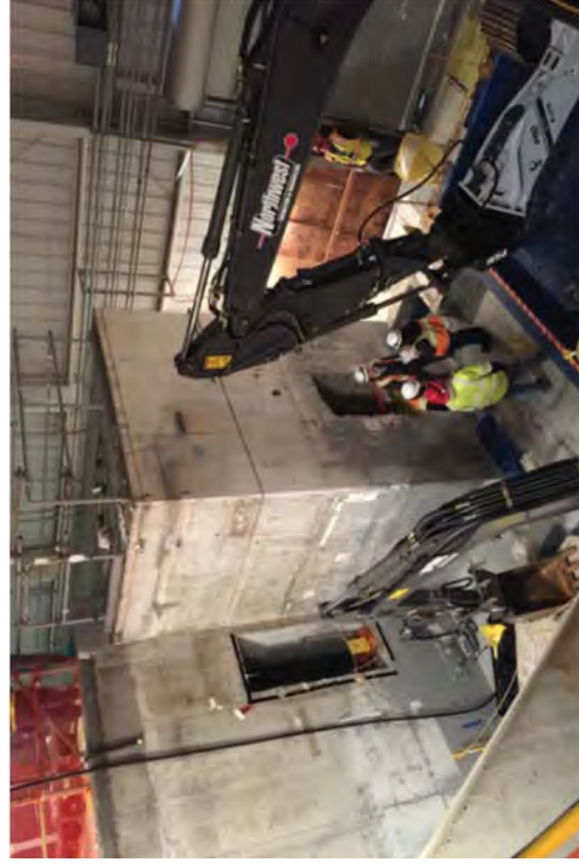
Personnel performing a PPE dry run in the LRWB before starting demolition work.
