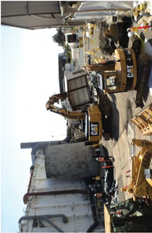
Preparing the metal building for demolition, size reduction, and loading into an intermodal.
