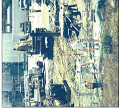
Asbestos Abatement workers were supported by Waste Management while removing transite pipe.
