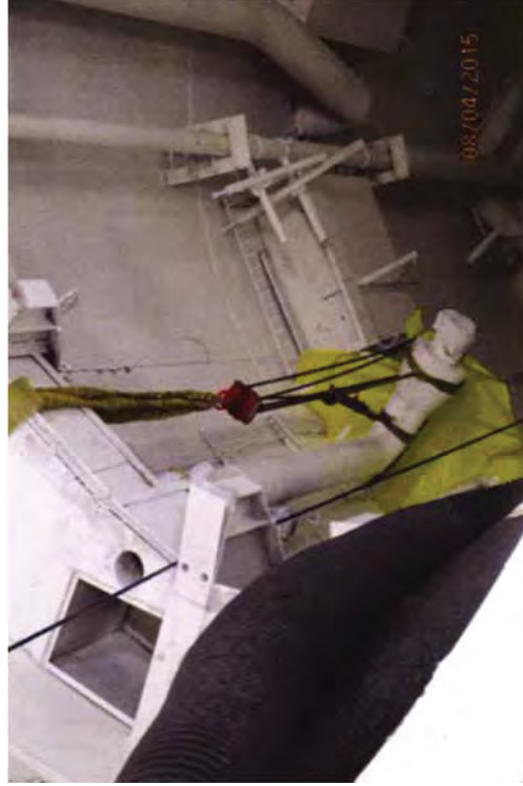
Removing a section of 8-inch feedwater pipe after various lift plans were evaluated.
