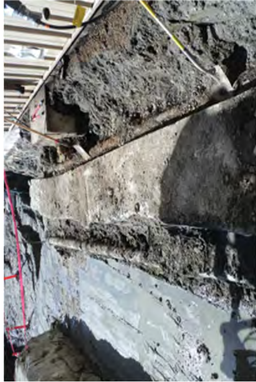
The transite fire line, electrical raceway, and iron 4-inch LRW drain line exposed.
