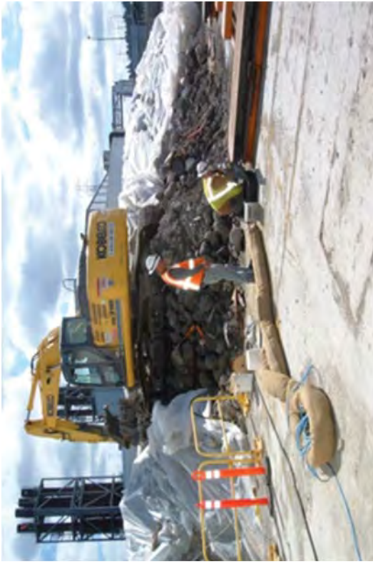
The spotter for an excavator ensures that a worker does not enter into its swing radius.
