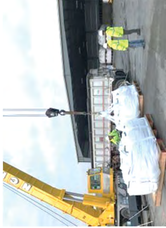
A crew preparing soft sided bags to itemize and load soil onto trucks.
