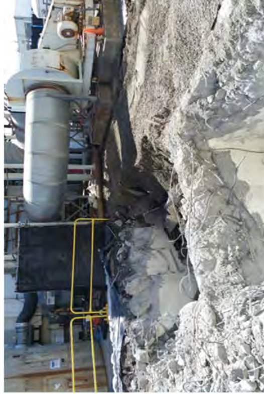
West edge of the SAS below grade looking SW to the MPEF foundation slab. The foundation had to be protected and the MPEF had to be kept in operation because it was a critical component in future demolition activities.
