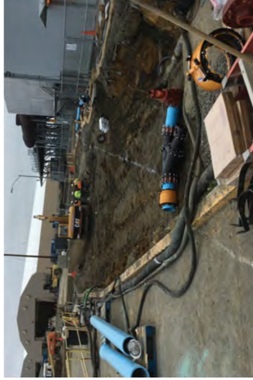
Piping material that was prefabricated for the fire line. A white CW line is marked out. The crew in ditch is obtaining samples for FSS and GPS location.
