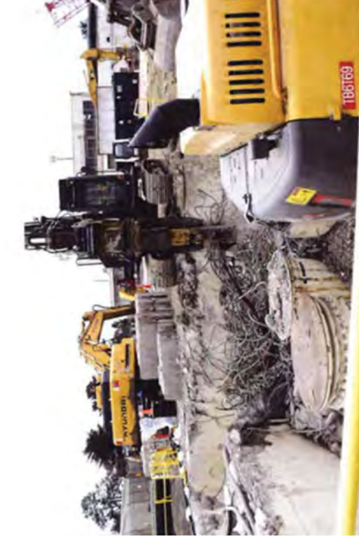
Shearing rebar with hydraulic jaws so that it will fit into intermodals.
