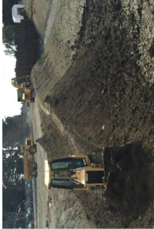
Grading an access path from the old Parking Lot A to the canal. This area will eventually be one contiguous wetland.
