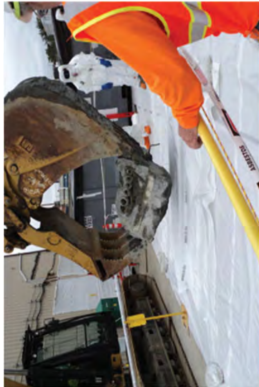
This is a collar section containing visible transite pipe that broke off the raceway base connecting to the east-west electrical run.
