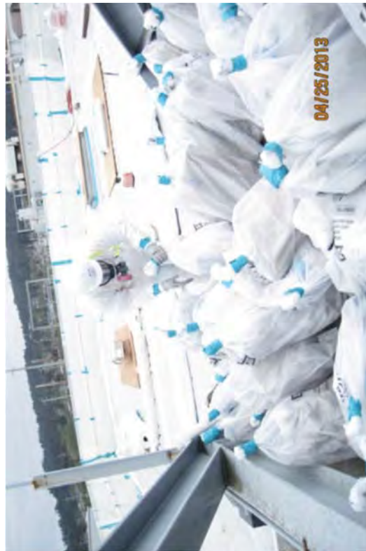
Stockpiled ACM waste on the roof of the RFB.
