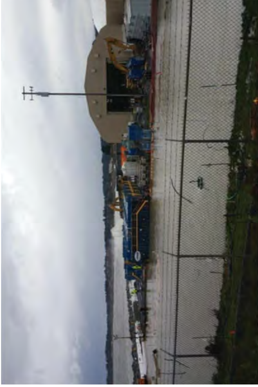
A view of the flooded Discharge Canal after the storm in late 2015.
