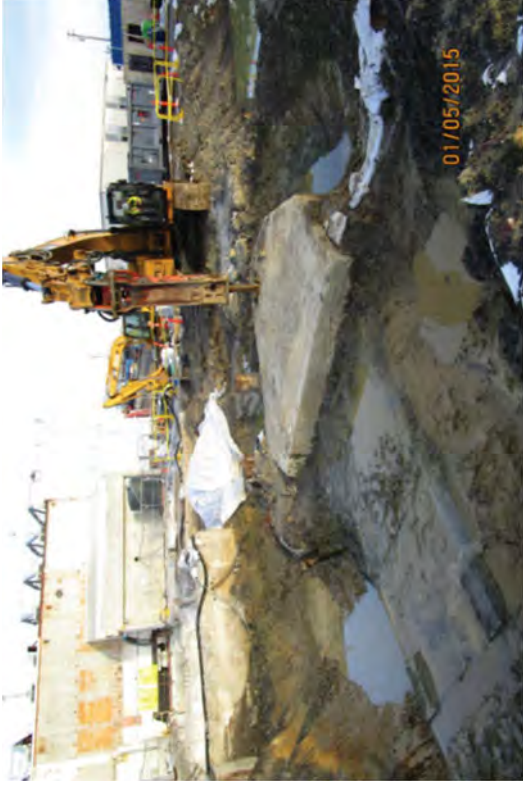
Demolishing thrust block "W". The chase in the foreground contains a section of 39" inch cooling water pipe.
