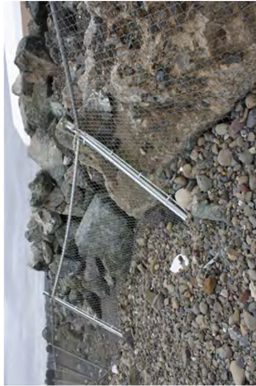
Fence damage from a storm.
