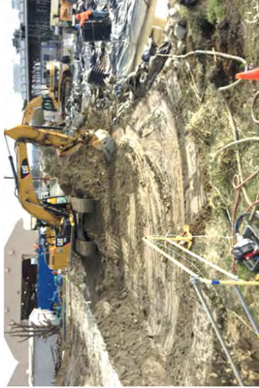
The South Discharge Canal area was prepared and surveyed. Impacted utilities were located in preparation for installing sheet piles.
