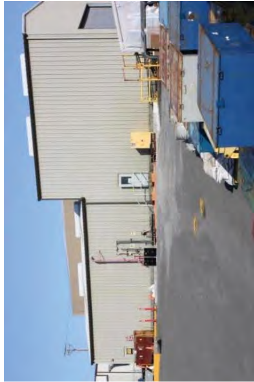
A view of the area after the LLRW Building slab, SRW Building, and underground utilities were removed.
