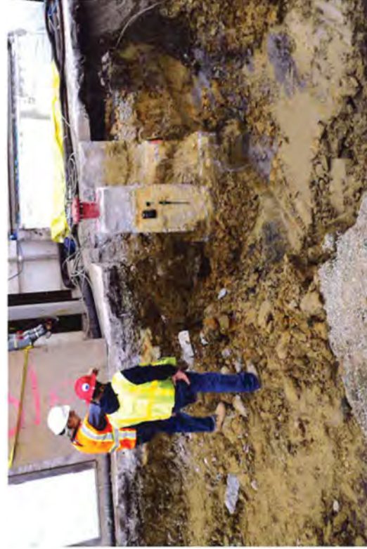
Engineering staff gave directions that a steel pipe had to be cut and the concrete thrust block and corner of the PEG room footing had to be removed.
