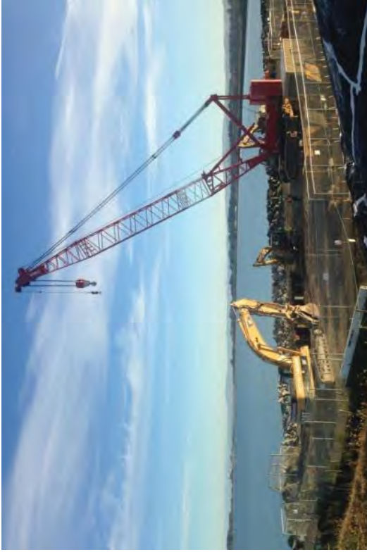
Sheet pile removed from the Humboldt Bay side of the re-established sea wall.
