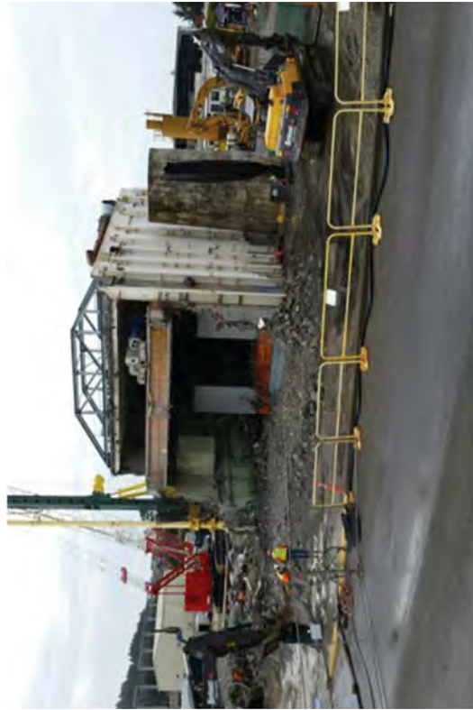
The 75-Ton trolley crane was pulled off of its rails and to the ground before CSM wall pre-trench work began and water management controls were put in place. The 75-ton crane was then segmented and removed.
