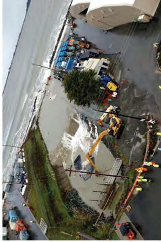
The secondary dam was breached during the storm in late 2015. Crews recovering the bladder from the south end of the canal.
