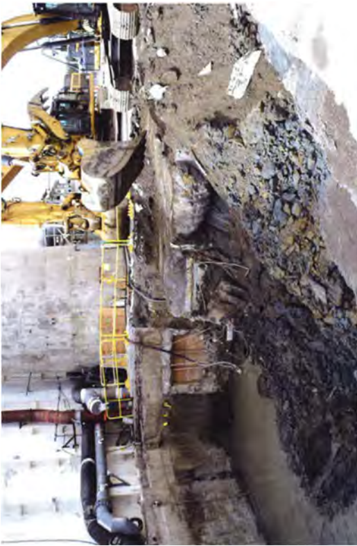
Using an excavator to remove soil from around wooden pilings and beginning to expose the LRW tunnel.
