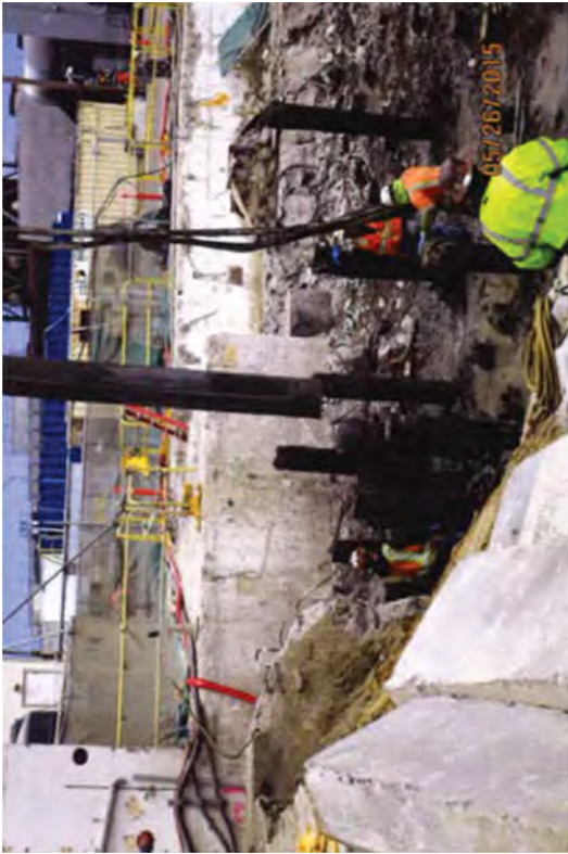
Using a crane with a pipe drilling attachment to vibrate wooden pilings loose.
