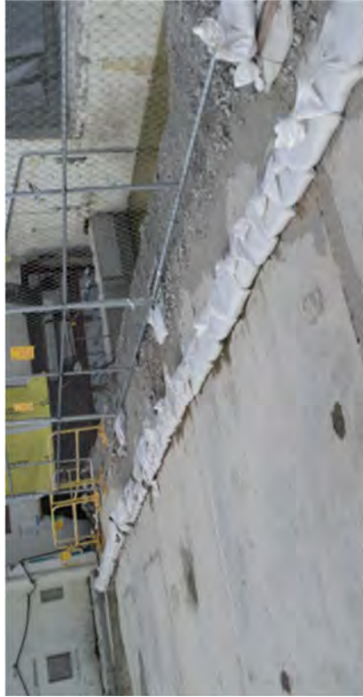
BMP's installed along the TB foundation's border with Unit 2 in preparation for excavation.
