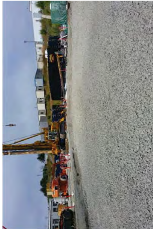
The work surface for the hydromills ready to be used after it met the required standards.
