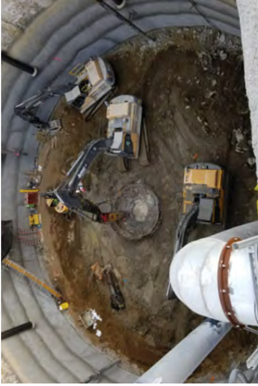
Using an excavator with a hammer to break apart concrete on the interior of the Drywell.
