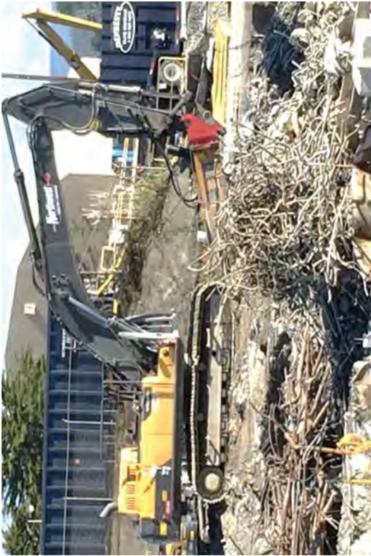
Rebar and metal removed from the Caisson excavation which will be loaded into IM's.
