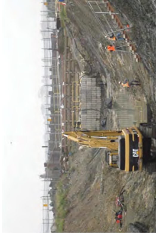
Discharge Canal remediation progresses towards FSS so that soils can be stored in the empty canal and re-used to backfill the Caisson excavation at a later date.
