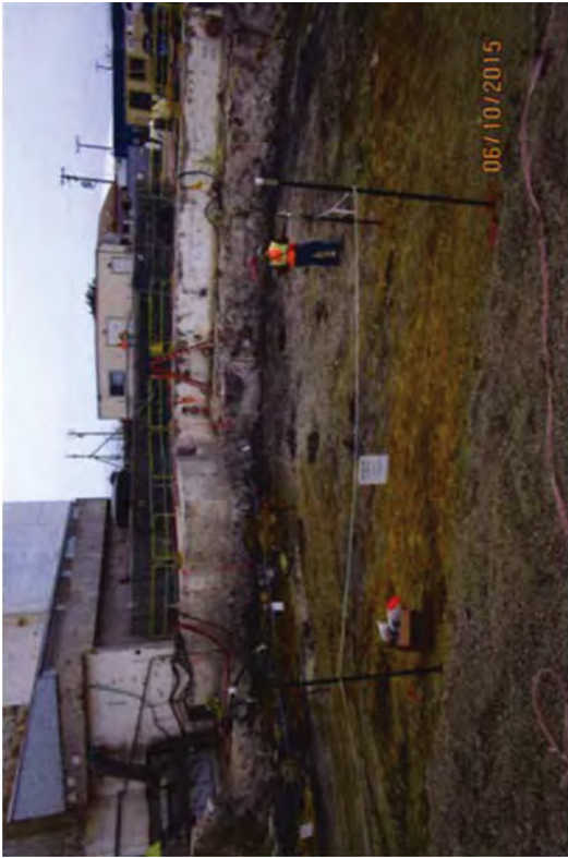
RP techs performing the FSS on the west end of the TB excavation.
