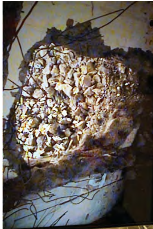
The concentrated waste tank pad was demolished by remotely operated equipment to prevent workers from being exposed to contamination.
