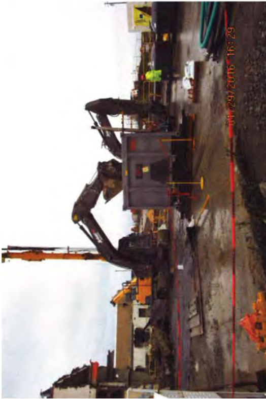
Loading out waste into an intermodal that is sitting on a portable scale.
