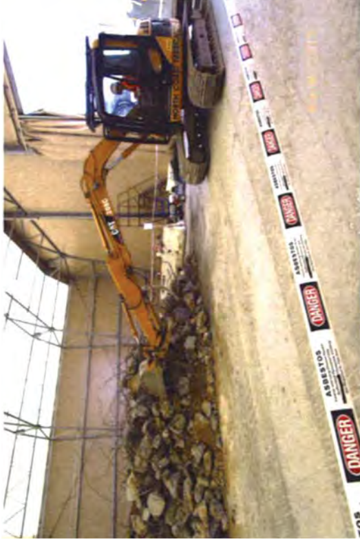
Using a small excavator to sort and load TB debris into intermodals.
