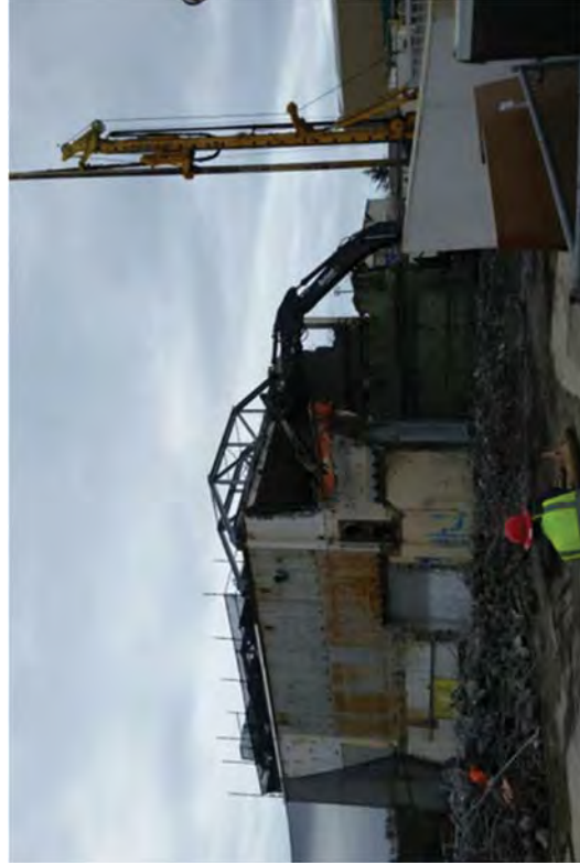
Demolishing the RFB while a crane works nearby to install the CSM wall.
