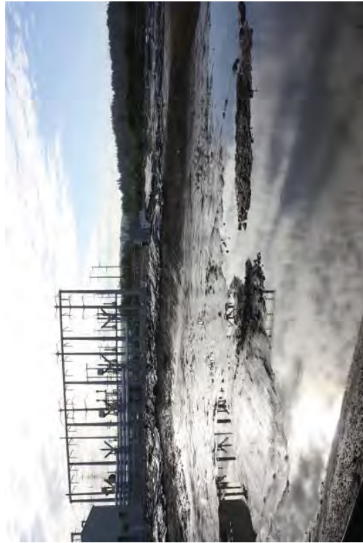
Intake Canal before restoration work.
