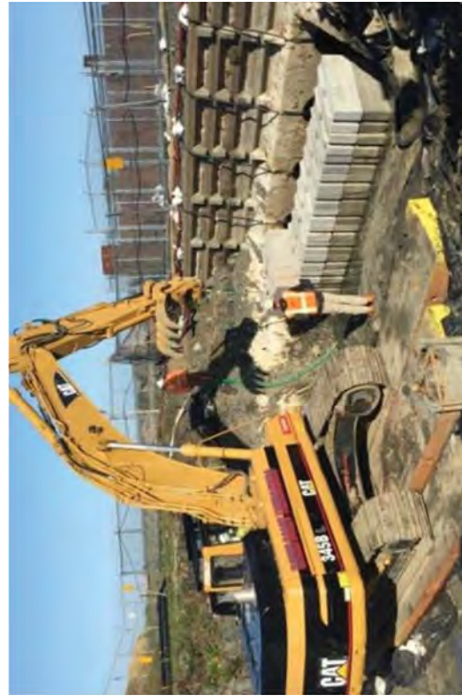
A civil engineer checking to see that the eco blocks are installed properly.
