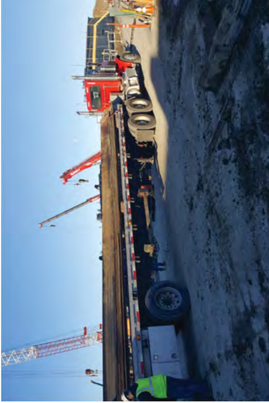
Moving the sheet pile out of the area for so it can be surveyed and released from the site.
