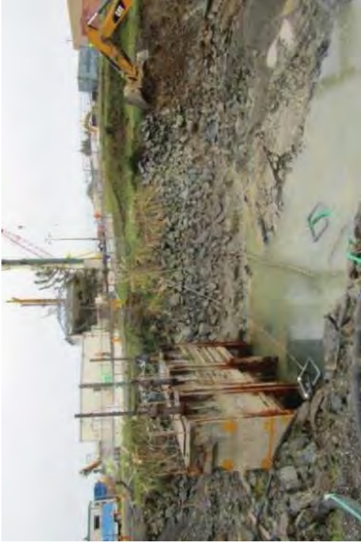
Removing the remaining riprap. Pump boxes with mesh sides are in the water.
