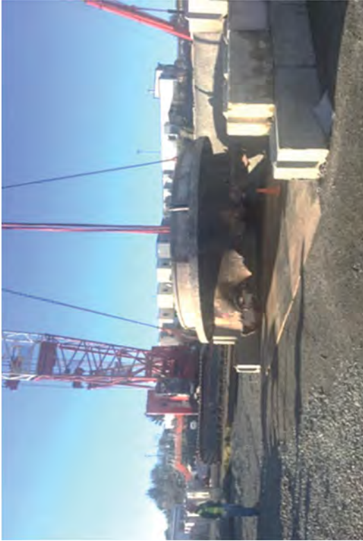
Upper ring of the drywell located in the bull pen for size reduction and loading into IM's.
