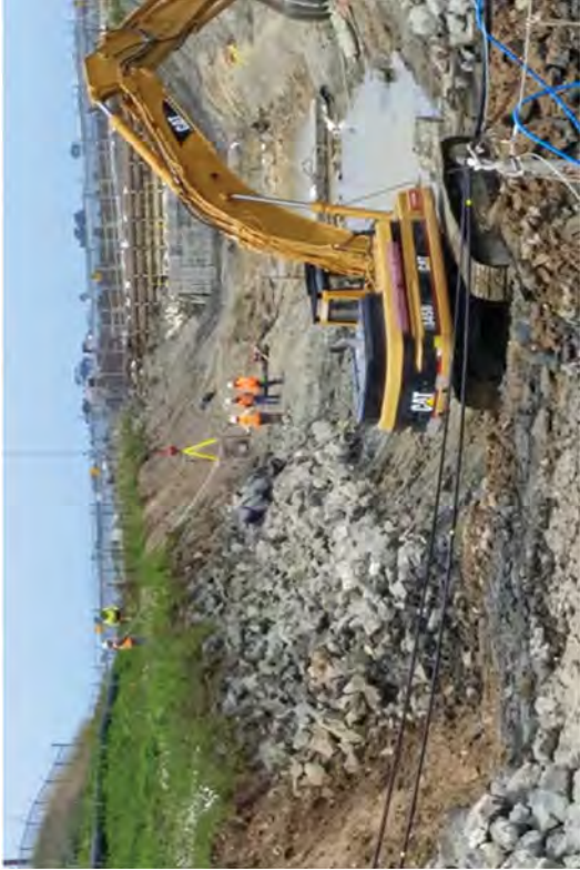
Removing riprap from the south bed of drained canal. FSS is being performed on the North end.
