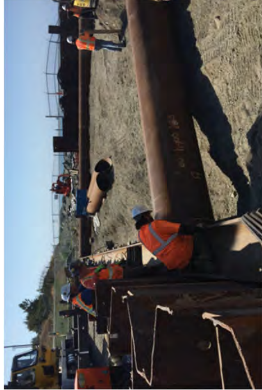
The south end of the water supports which brace the sheet piles against the force of the waves.
