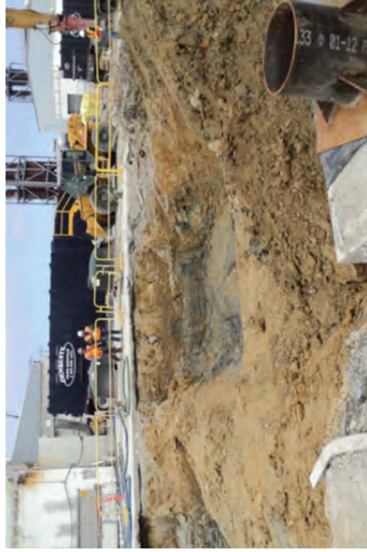
The Unit 2 footprint excavation at a depth of approximately 10 feet below grade where deep feature removed.
