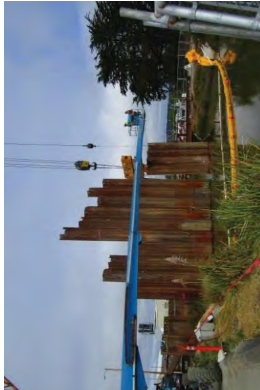
The crew in the lift attaching the driver to the sheet pile. The yellow boom in the water is a silt curtain.
