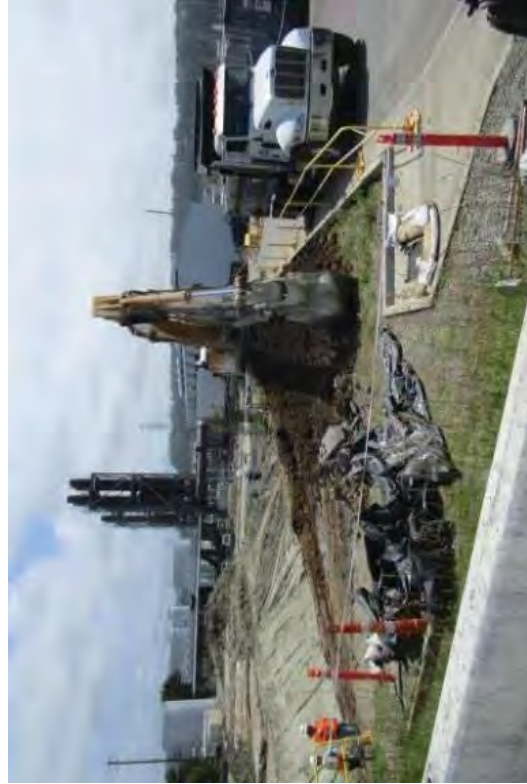
Beginning the excavation of the NE Laydown Area which will eventually blend into the canal
