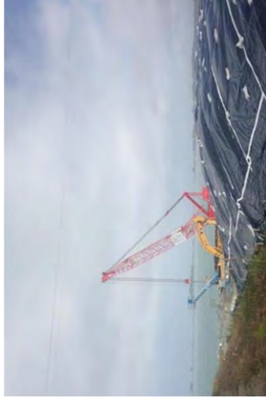
Removing sheet piles from Bay with covered CSM soils in the foreground.
