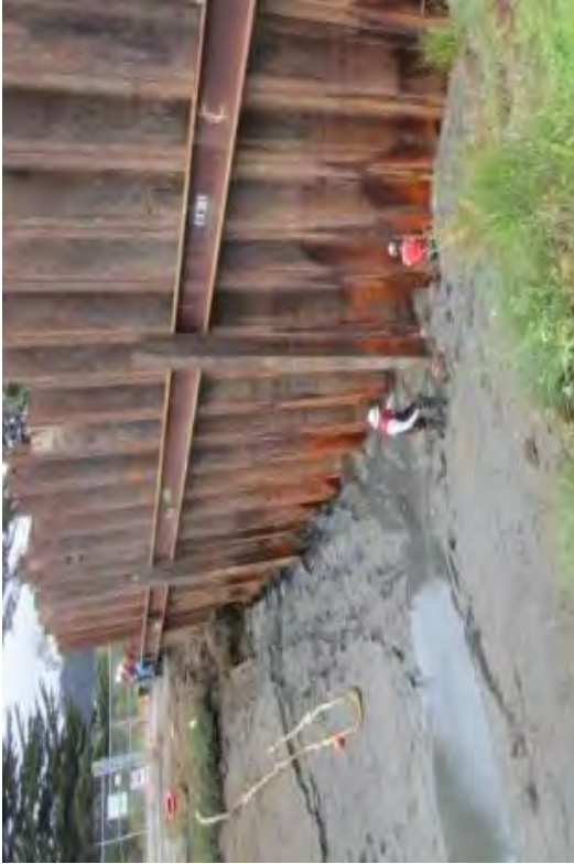
A pump was placed at the low point as planned because in-leakage was always expected.
