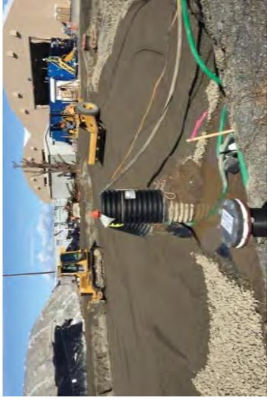
The crews laid geotextile fabric, rock, and a base layer before compacting the area to prepare it for sheet piles.
