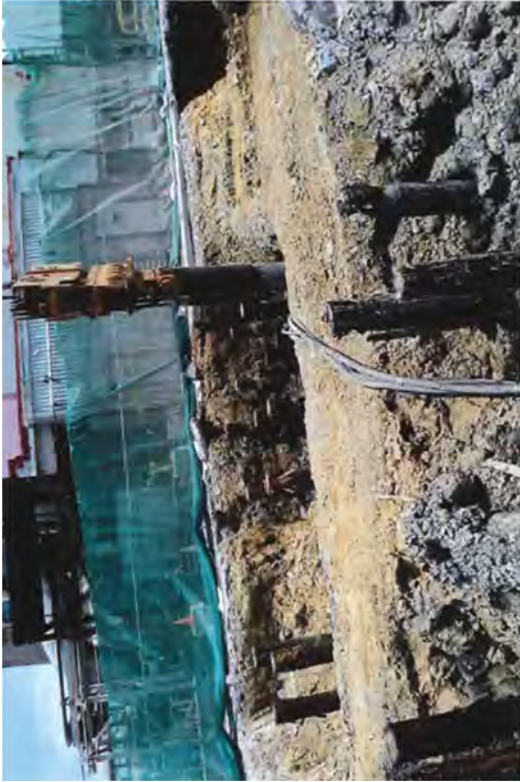
A vibratory hammer forcing a pipe sleeve over a wooden piling to free it by breaking the suction created by the dense clay layer.
