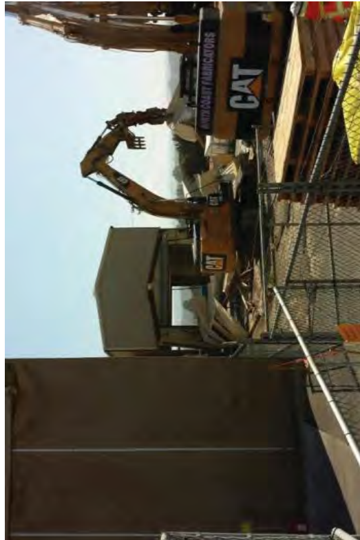
Workers evacuated the RUBB tent while demolishing the steel and metal structure of the SRWB because the two structures were so close.
