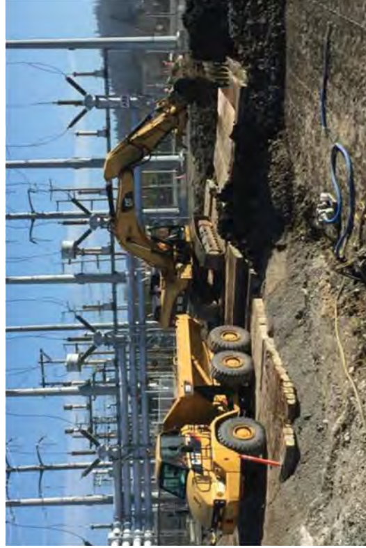
An excavator moving and placing soil at the south end of the canal.
