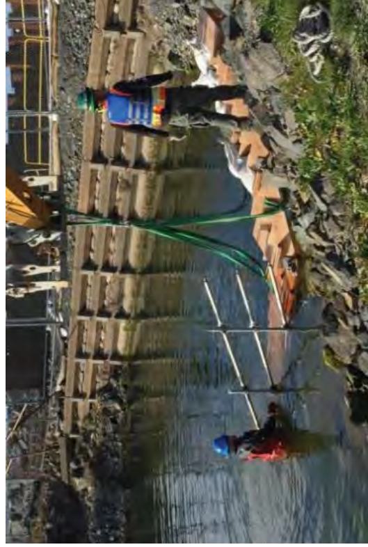
Divers installed inflatable bladders to plug the four uncovered concrete outlet pipes and completely close the canal off from the bay. The rubber bladders were 10 feet long and filled with nitrogen.
