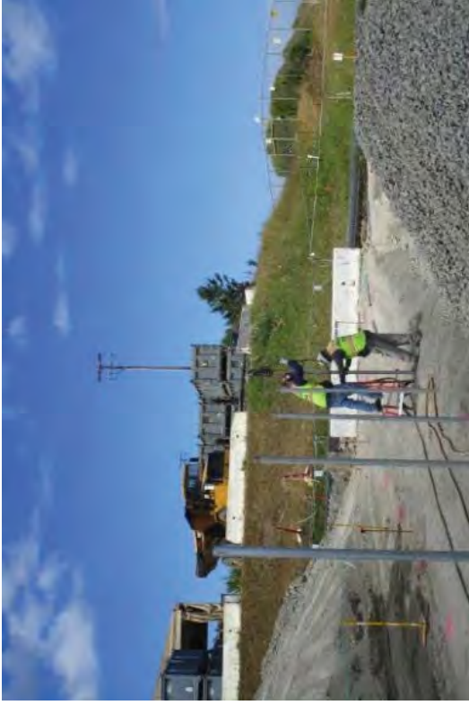
Installing fencing for a bypass trail while the Discharge Canal outlet pipes were being removed.
