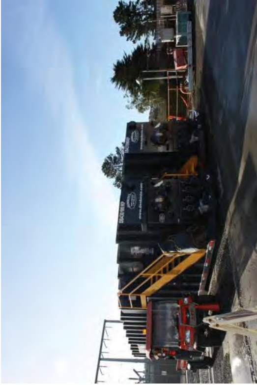
GWTS storage tanks throughout site.
