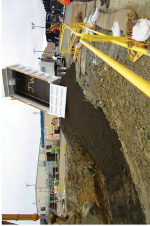
Beginning to backfilling over the CLSM and a layer of geotextile fabric.
