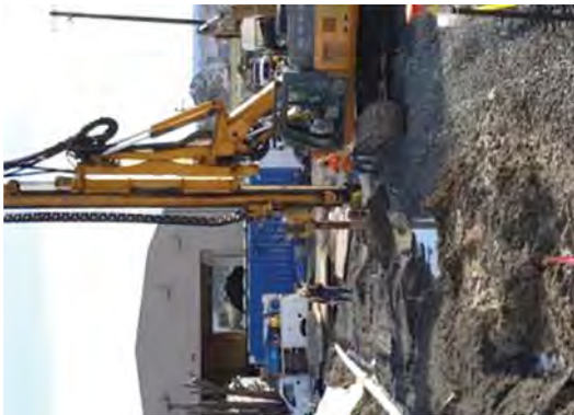
Crews pre-drilling for a third sheet pile near the south end of the discharge canal.
