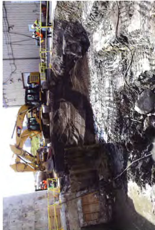
Backfill material was delivered to create a ramp to access and remove sheet piles and wooden pilings.
