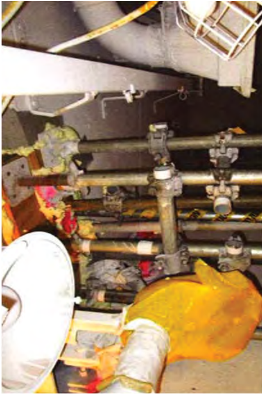
RP directed that some pipe ends were to be filled with a two-part expanding epoxy foam. The scaffold in this photo is supporting the bulkhead.
