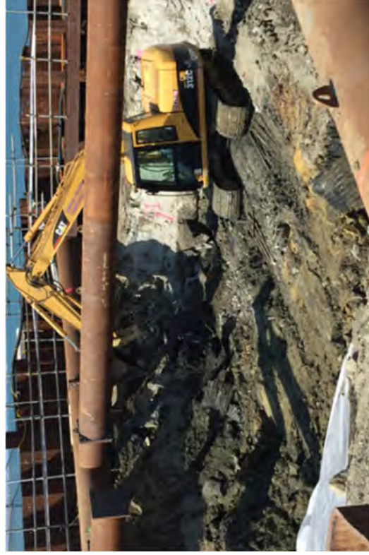
Continuing the excavation to expose piping. The pipe came out in scraps, not large sections.
