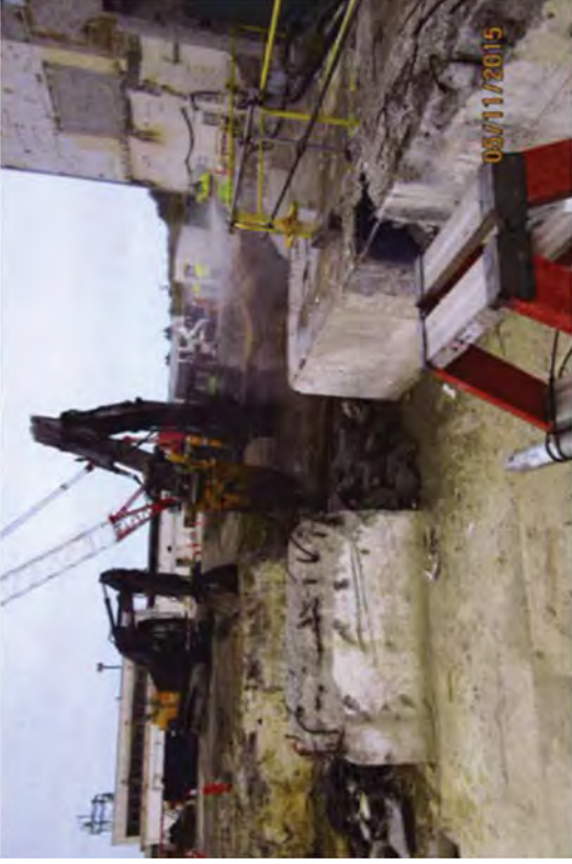
Demolishing the TB foundation. Parts of the concrete slab and pedestals were 6 feet thick.
