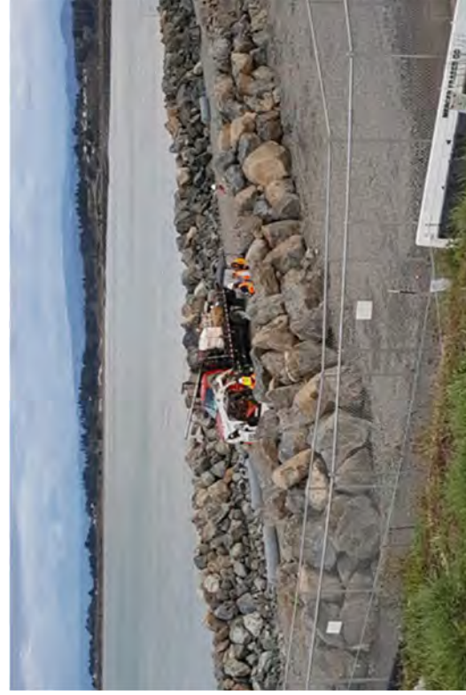
A crew began digging post holes to reestablish the perimeter fence. The temporary pedestrian trail fence is in the foreground.
