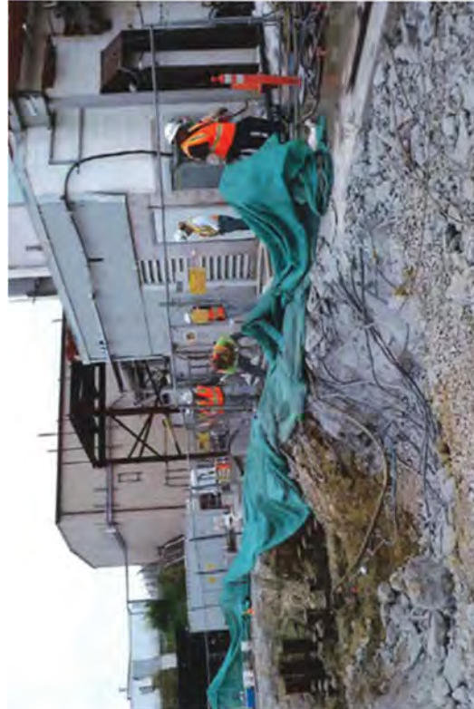
The RCA fence was moved east under the guidance of FSS so that demolition of the TB Foundation could continue.
