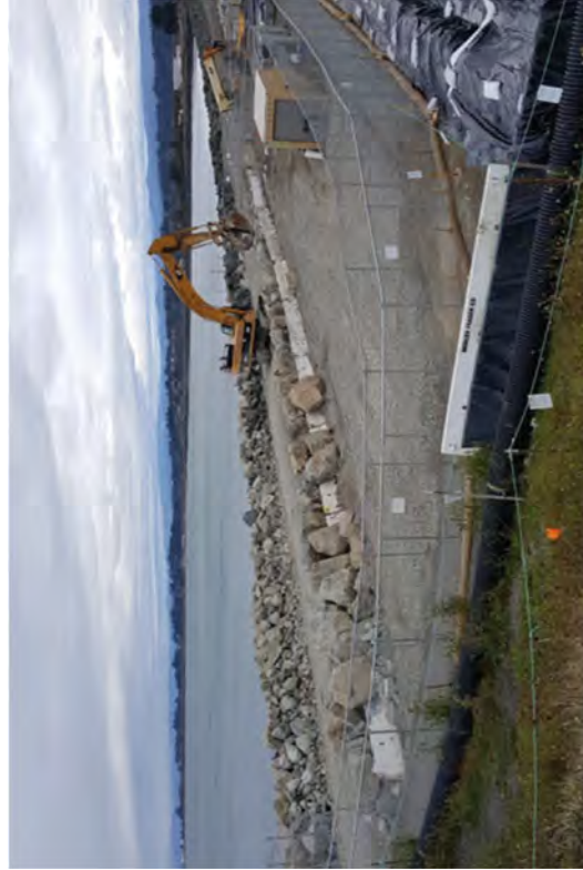
An excavator building a riprap pile around the K-rail as a secondary wave protection measure.
