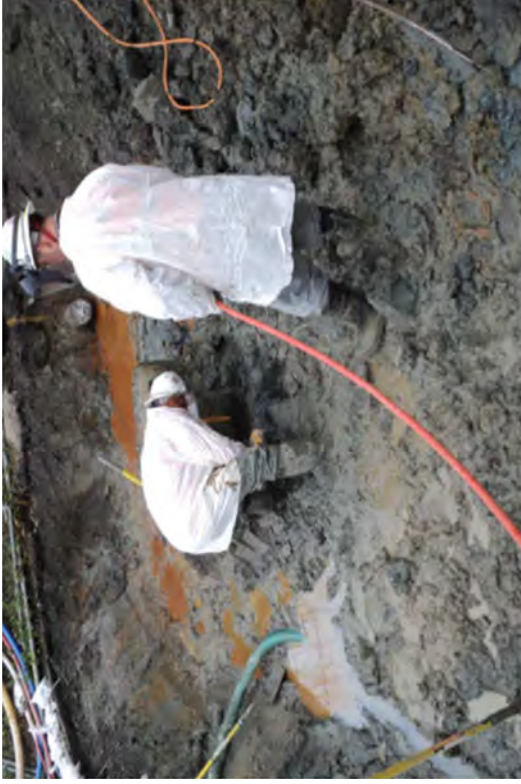
Crewmembers cutting bolts from a metal flange which connects transite pipe to a thrust block.
