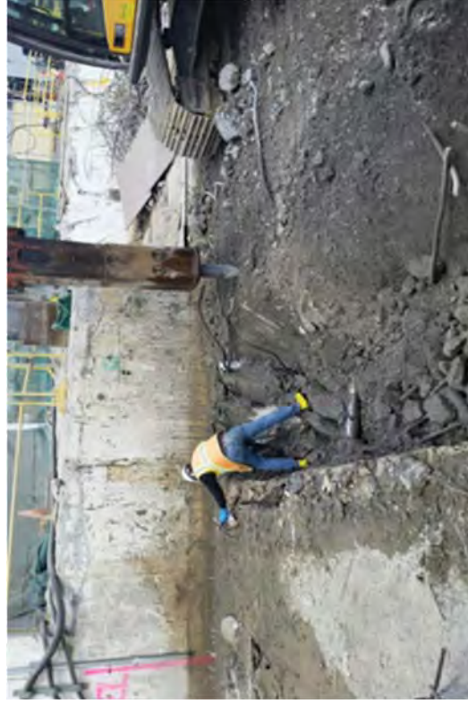
RP technicians surveying embedded drain lines while removing the TB floor slab.
