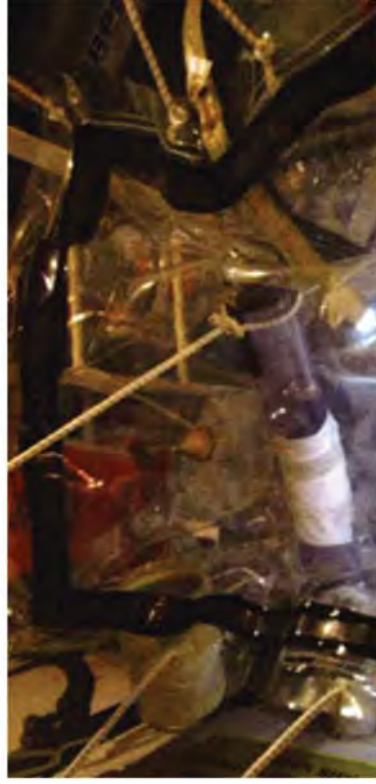
A spent fuel drain pipe was inspected with a borescope camera after being wrapped with a glove bag.
