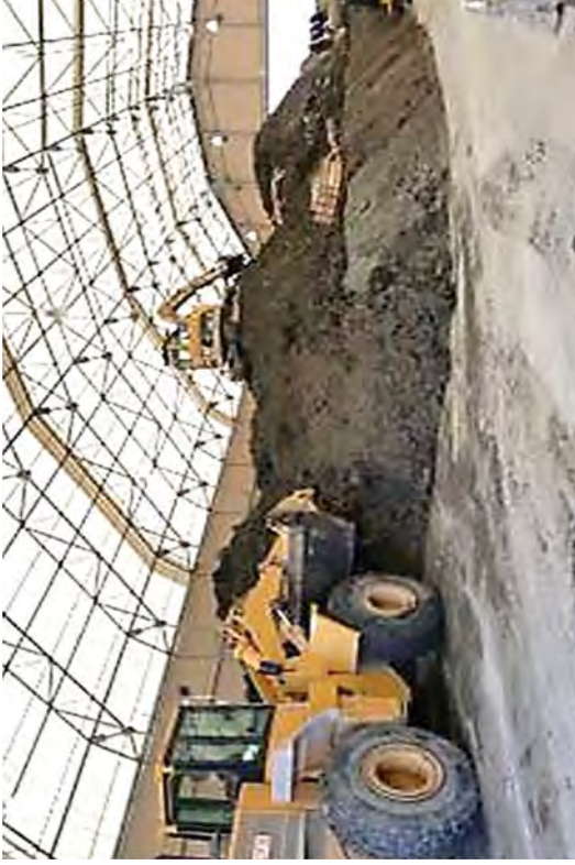
Soil mounds in SMF grow as Rip-Rap and mud from the Intake Canal are added.
