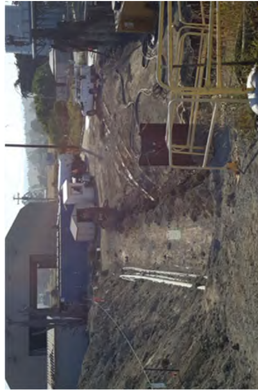
Removing Circulating Water Lines and sheet pile from the North end of Area D.
