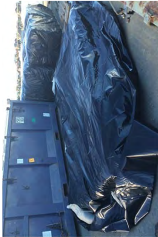
A contaminated 17,000 pound, 10-foot wide, 3-inch thick steel seismic impact plate that was removed from the Caisson excavation wrapped in plastic and being prepared for disposal.
