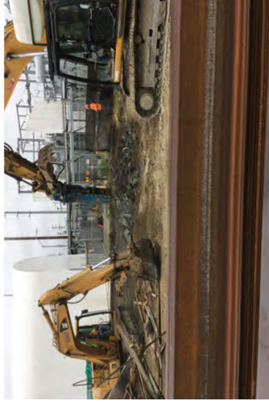
Removal of the concrete wash pad along with its wooden fencing, area was then sampled by Environmental and surveyed by FSS.
