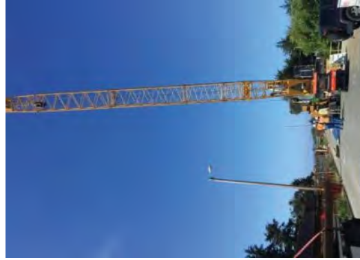
Crew driving sheet piles into the Intake Canal using the 330-ton crane.
