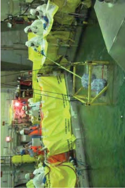
Removing debris from the SFP that accumulated as a result of the divers' underwater work.
