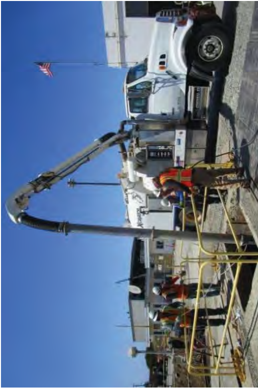
Cells in the Intake Structure were filled with gravel after any pumps, equipment, grating, and piping was removed.
