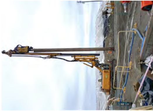
Crews installing a third sheet pile near the south end of the discharge canal.
