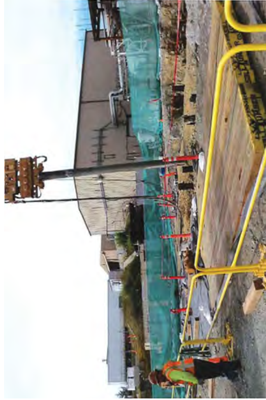
Loosening wooden pilings.
