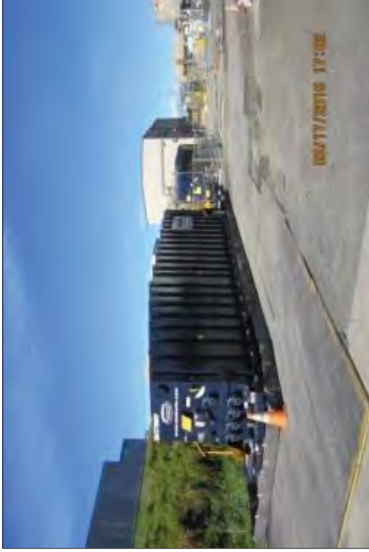
A FRAC Tank in position to drain and dispose SPF water
