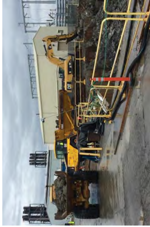
Loading Intake Structure rubble.
