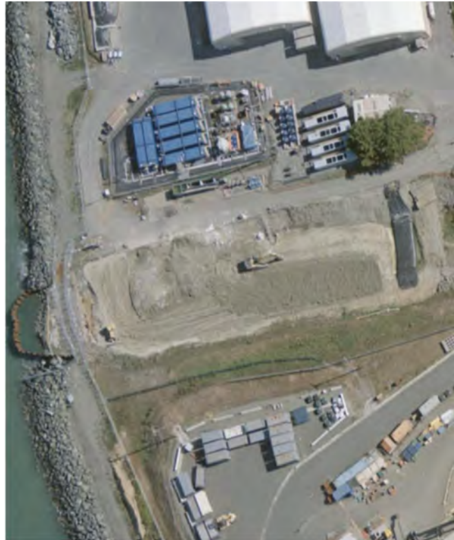
An aerial view of Discharge Canal and GWTS before winter storms in late 2015.
