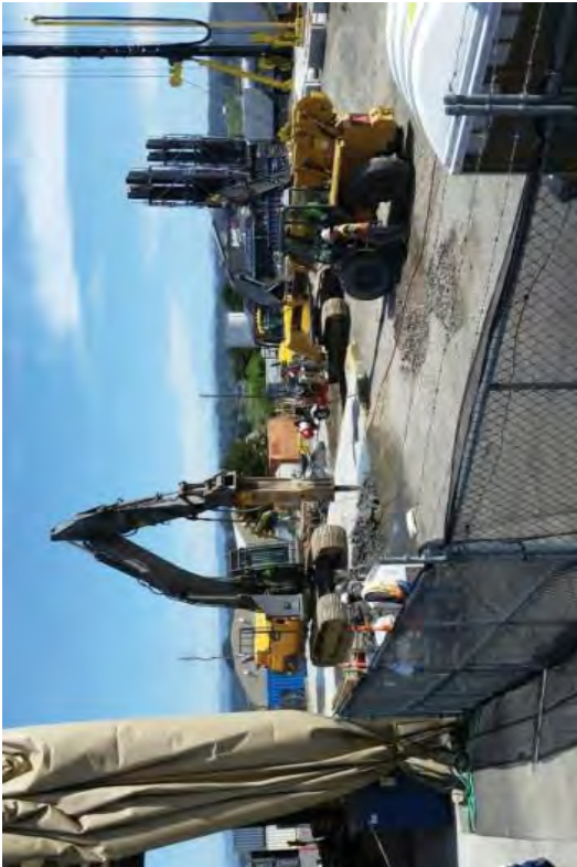
Using an excavator equipped with a hydraulic hammer to break apart the SRWB slab.
