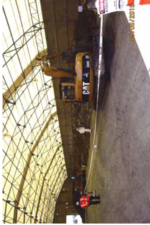
ACM is segregated from other materials and monitored by an abatement supervisor.
