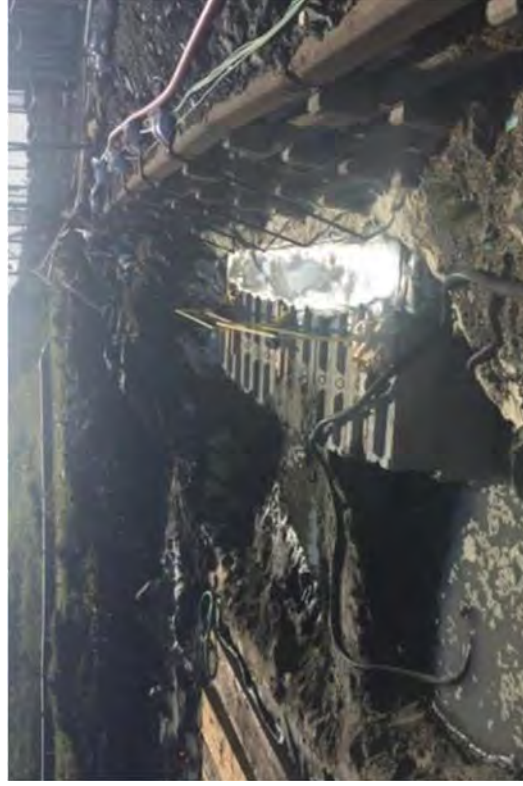
The finished temporary cut-off wall with the sump pump hose in foreground.
