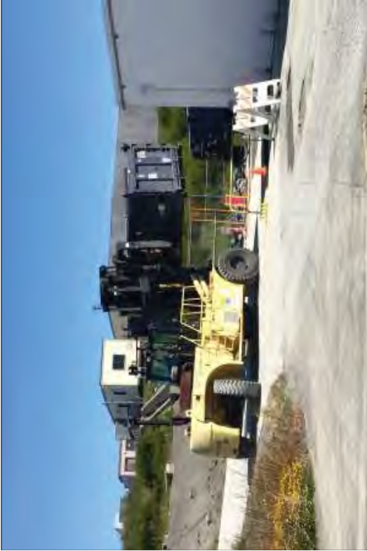
Maneuvering an empty IM into the Unit 1 and Unit 2 pad area so that it can be set up in the North Yard to load out concrete rubble from the LRWB walls.
