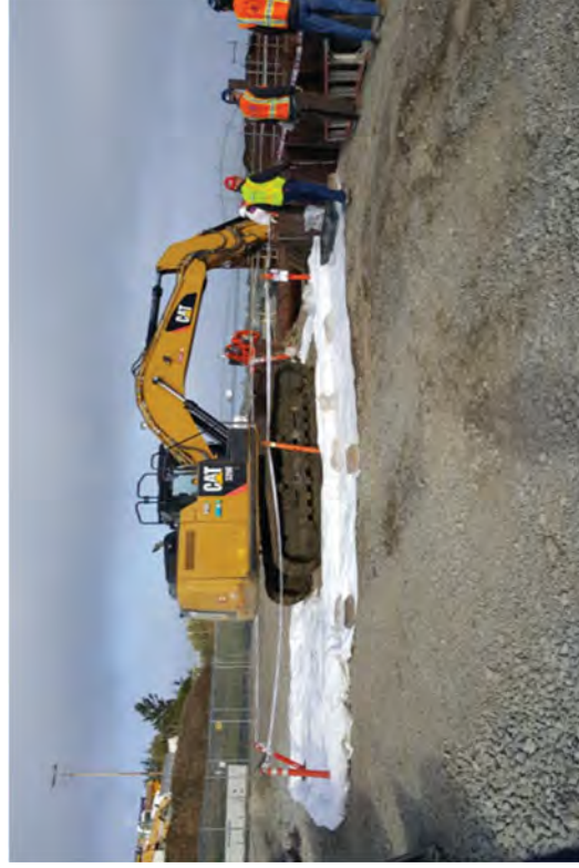
Preparing the working surface in front of the 48-inch discharge outlet pipes.
