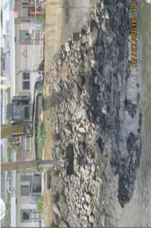
Removing riprap from the Intake Canal and transferring it to the SMF.
