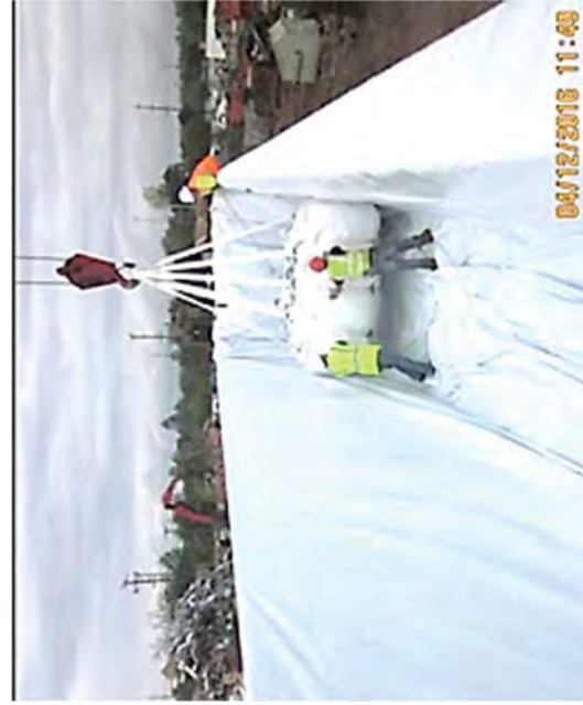
Loading IP-1 bags into a railroad gondola at the railway transfer station.
