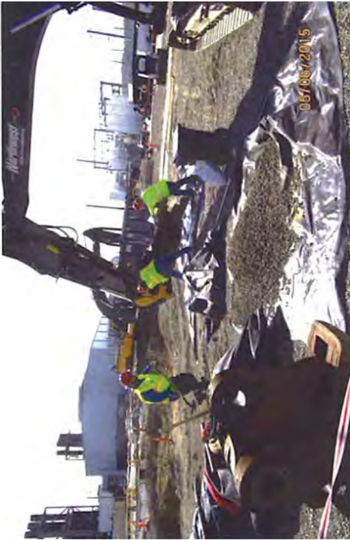
Any hydraulic leaks are contained and cleaned according to a set process. They were inevitable and caused by constant contact with rebar fragments and other rough surfaces.
