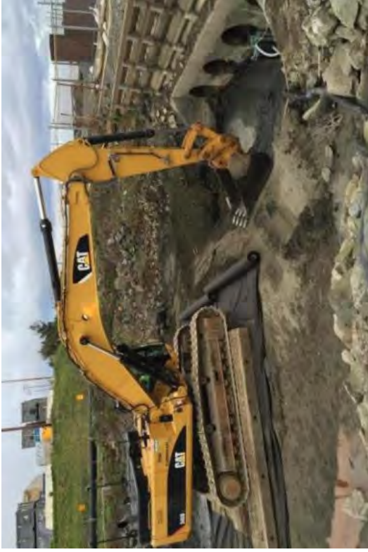
The first excavation in the canal was to uncover four pipes which provided access to install pumps.
