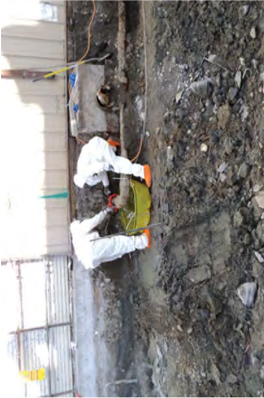
Crewmembers carefully cutting pipe at the LRWB foundation on the northern edge of the North Yard pre-trench area.
