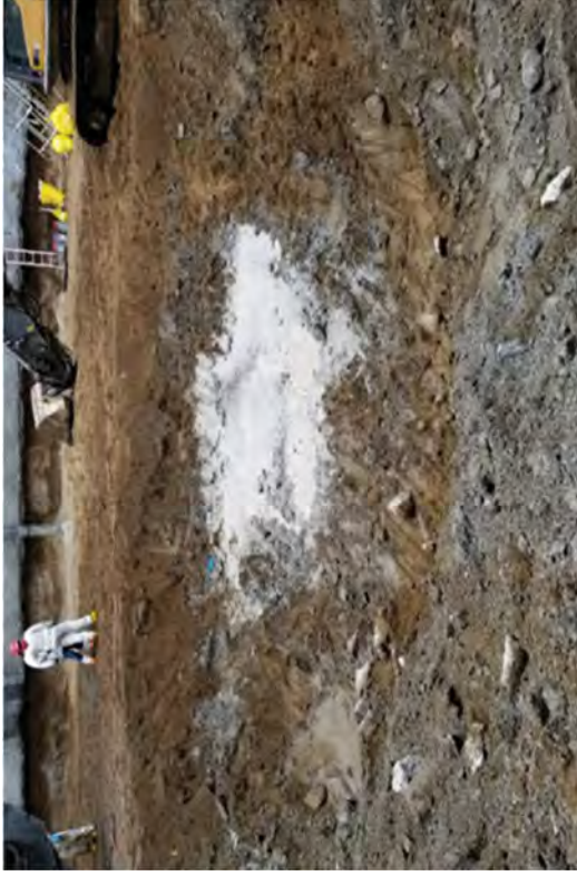
The area was excavated deeper than -76' EL after the concrete Tremie was removed with the purpose of being the final cleanup and to prepare for survey.
