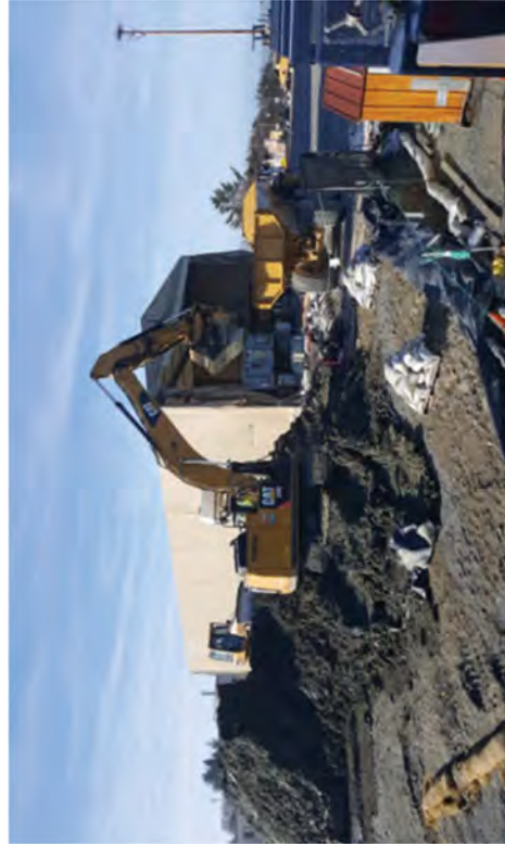
Moving Caisson excavation soils stored in North Yard to the SMF due to contamination.
