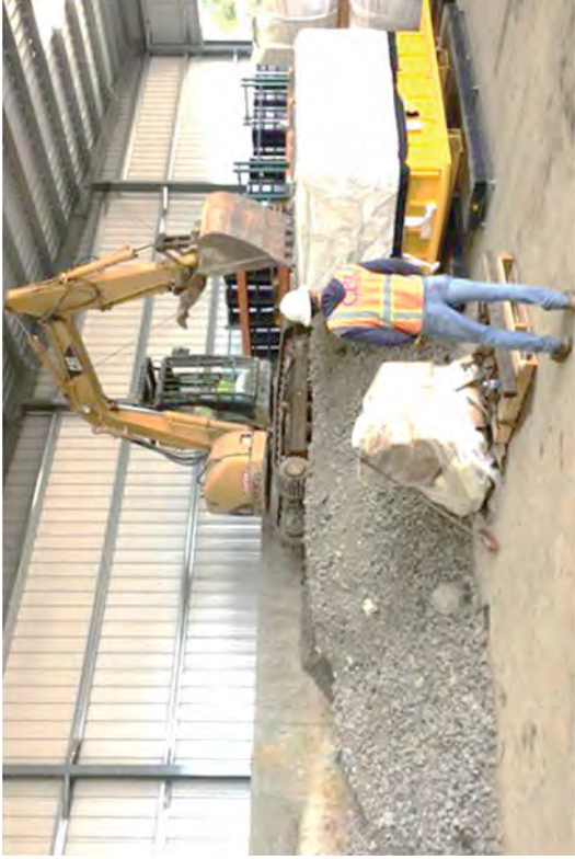
Size reduced concrete from the bucket crusher being loaded into waste bags.
