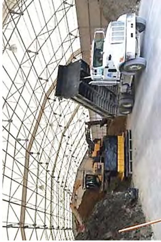
Safely and efficiently coordinating an excavator loading waste bags, dump truck unloading waste from the Upper Yard, and a second excavator conditioning waste for shipment inside the SMF Tent.
