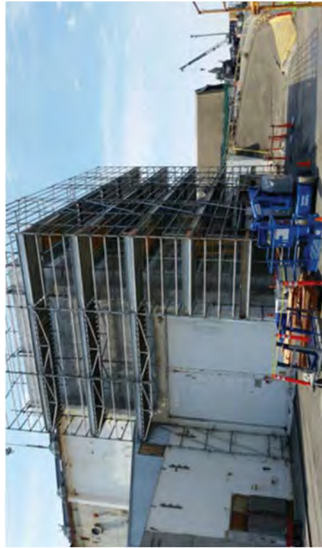
The RFB after completing asbestos abatement and removing the shrink wrap that encased the scaffolding.
