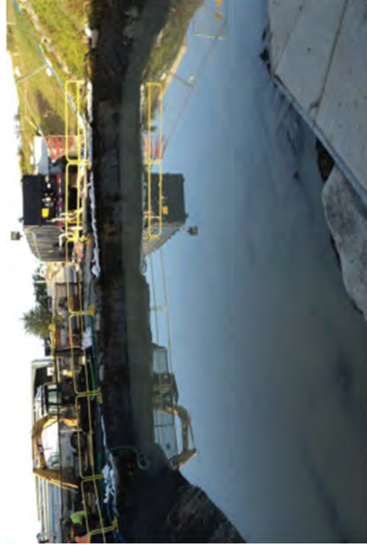
A typical accumulation of water in an excavation after substantial rains.
