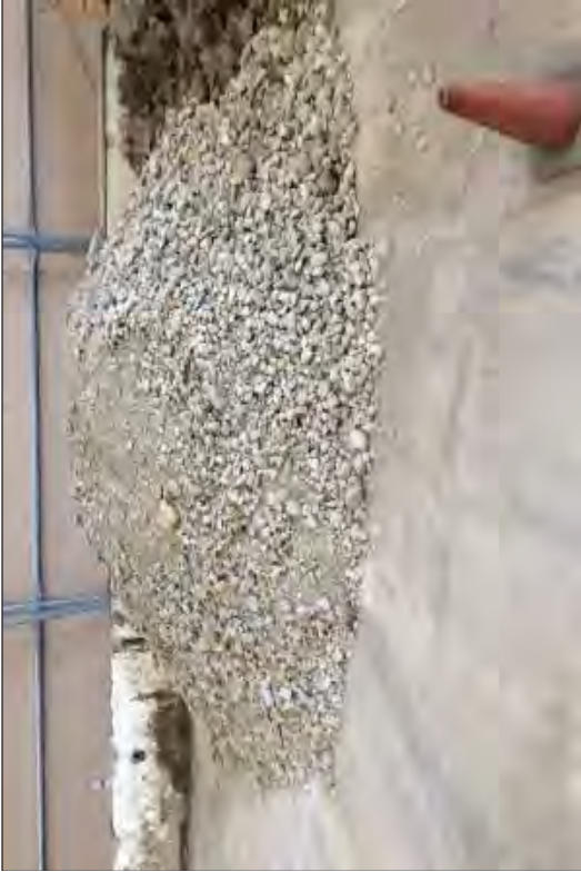
This 3 inch and smaller Backfill material from the North Yard was stored in the SMF because it failed screening through the GARDIAN due to contamination.
