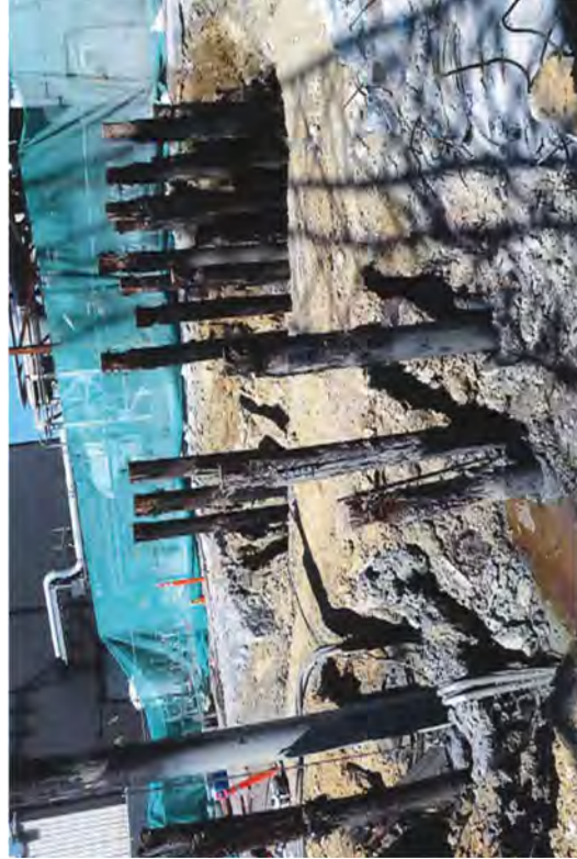
After the pilings are loosened with the hammer and pipe they can be removed from the ground with lower cost equipment than the large crane.
