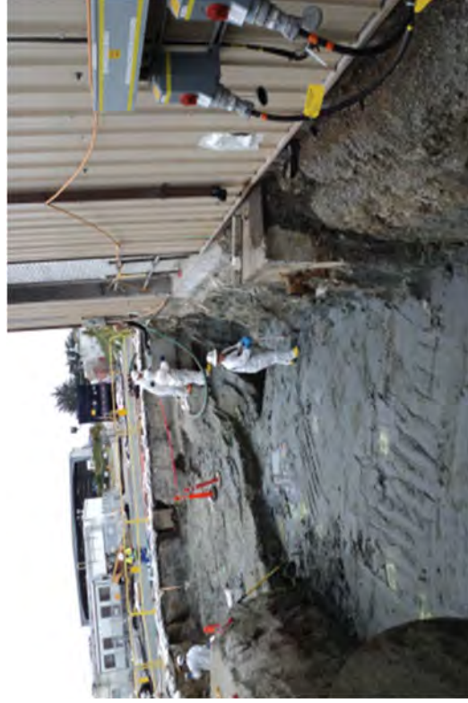
Continuing RP remediation activities after several rounds of digging and removing soil.
