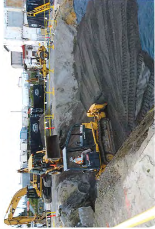
Operators using a backhoe to deliver fill material into the excavation where a dozer then spreads it.
