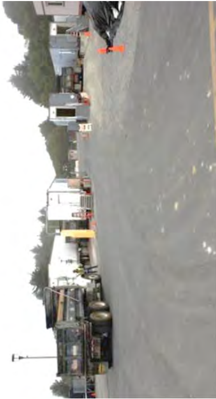
The center drive-thru area was one of two ways access HBPP. This access point is on the east side of the site.
