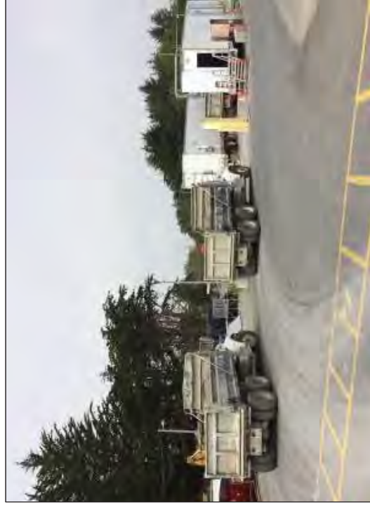
Three dump trucks full of backfill from the North and East Yard staged to be screened through the GARDIAN.
