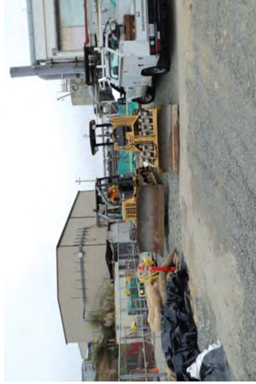
Backfill equipment arriving at the site, including a sheep's foot roller and dozer.
