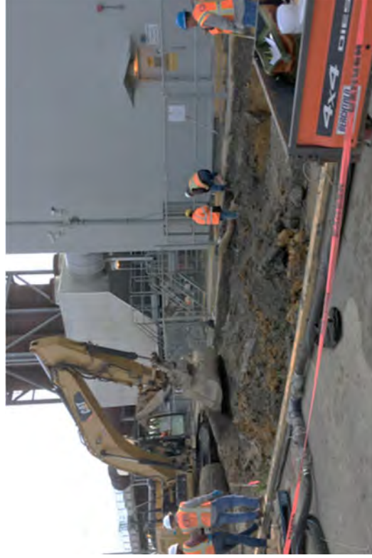
Relocating the fence and re-establishing its ground while RP technicians perform surveys.
