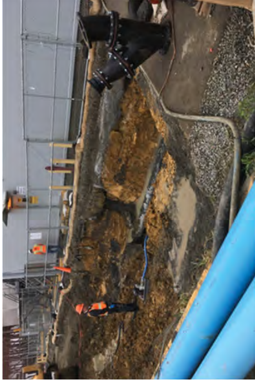
A plumbing contractor monitoring the water level for access to HBGS fire line.
