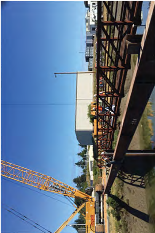
The guide rail for sheet piles in the foreground with the pedestrian bridge in the background.
