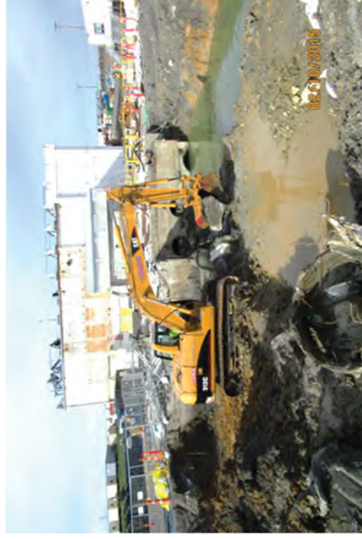
Removing concrete debris. Remnants of Circulating Water Pipe are visible in the foreground.
