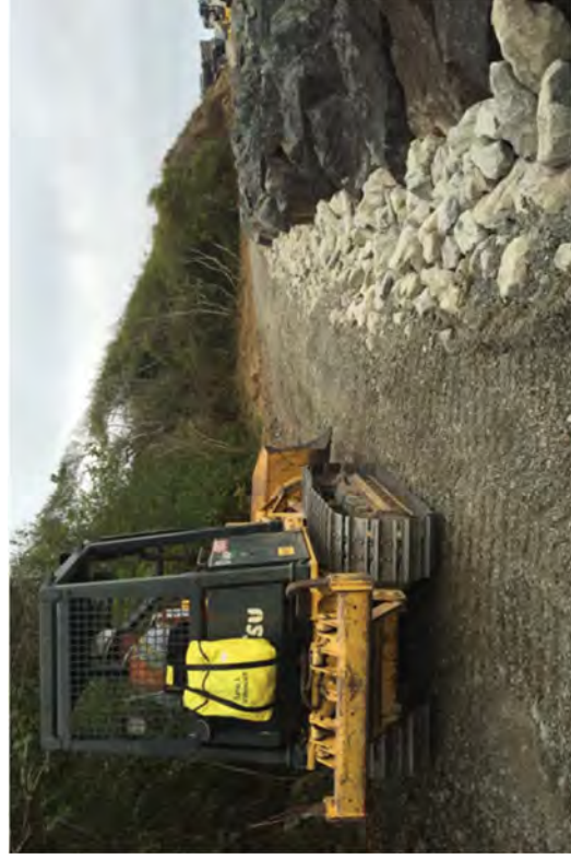
A small front loader spreading and leveling rock for the Coastal Trail.
