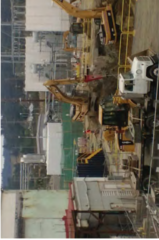
Excavating the southeast area of the Unit 2 footprint in preparation for the cutoff wall to be installed.
