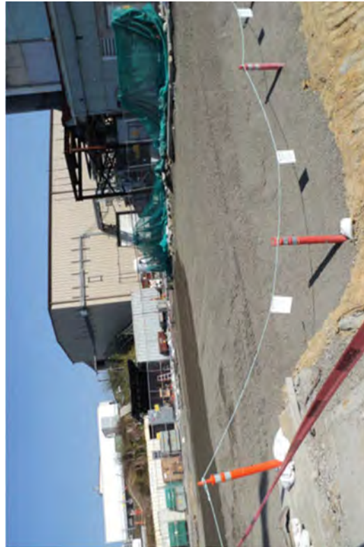
Backfill completed to be within 16 inches of grade at the north end of Unit 2.
