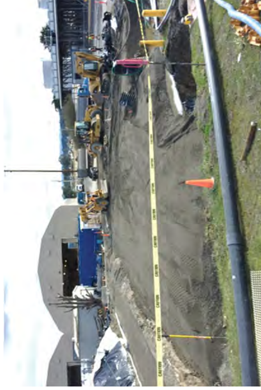
Inspecting sheet pile installation equipment after it arrived onsite while crews continued re-routing the GWTS.
