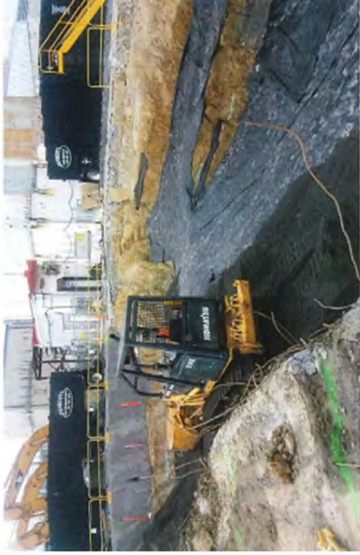
A layer of geotextile material was laid on the flat surface of the FSS area before it was backfilled.
