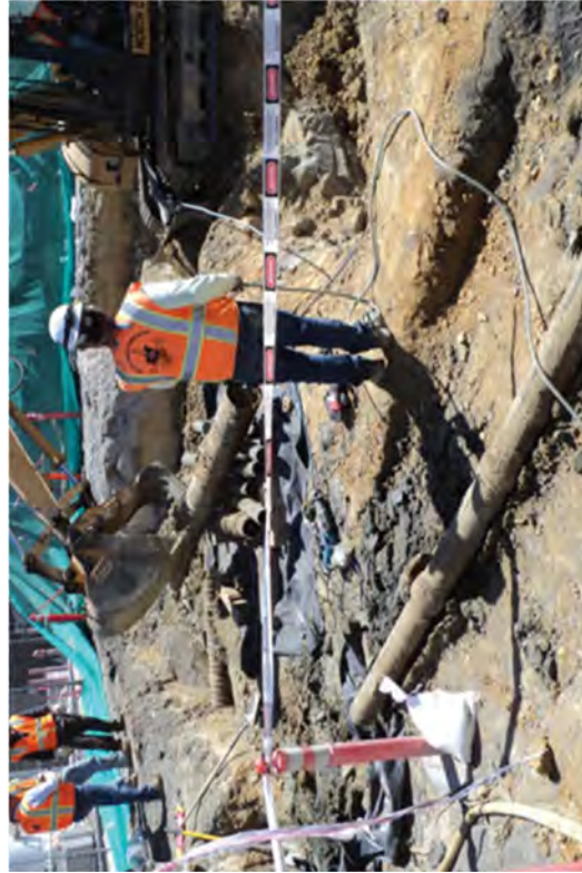
Removing cut steel and corrugated pipe from the north portion of Unit 2's footprint.
