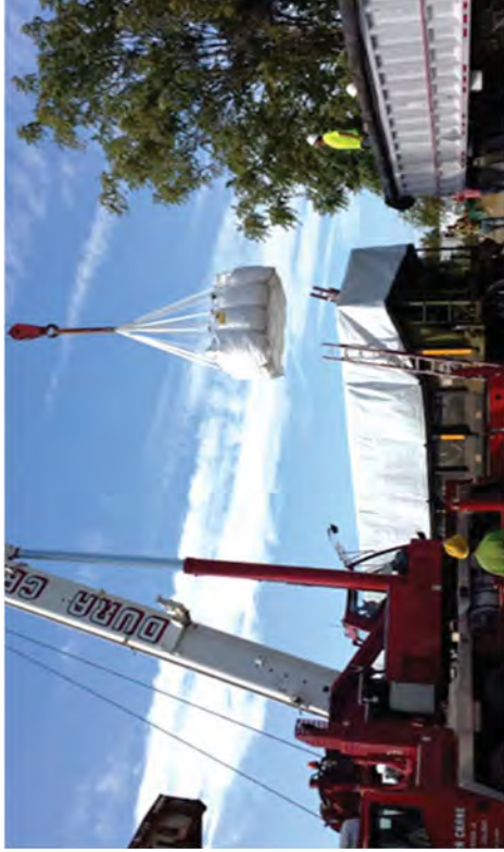
Loading IP-1 bags into a railroad gondola at the railway transfer station.
