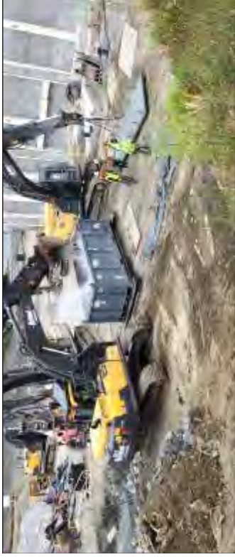
Placing an absorbent in an IM before loading it with concrete and debris.
