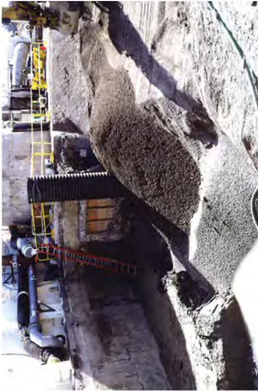
Spreading 1-inch rock over the excavation after a sump and pump were installed.
