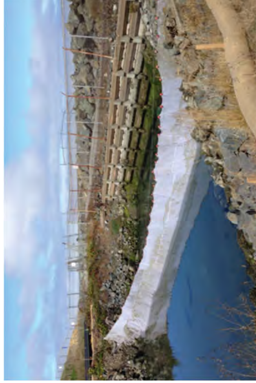
The block net installed. Tidal flow is restricted by sandbags placed inside the Discharge Pipes.
