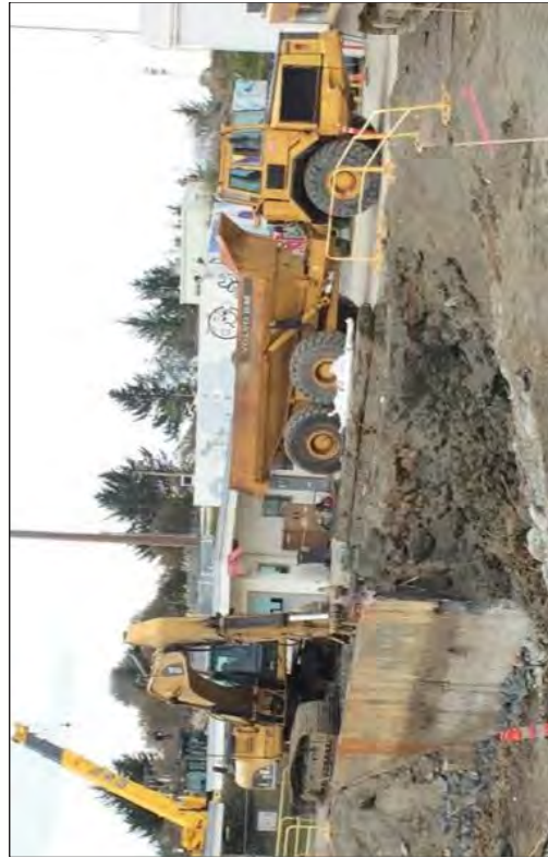
Removing the Intake Canal Headworks around the yard drain sump. The headwall, sump, and some surrounding soil was sent to the SMF as waste because of possible contamination. The overburden soil is stockpiled in the south discharge canal to be reused.
