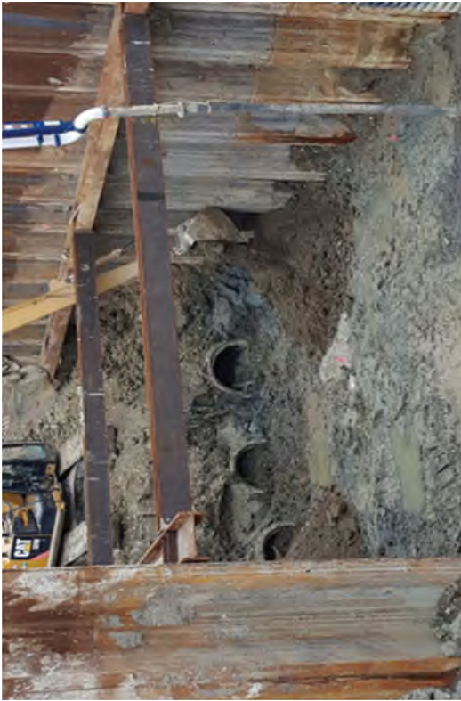
Backfilling the excavation after FSS to reduce the in flow of ground water.
