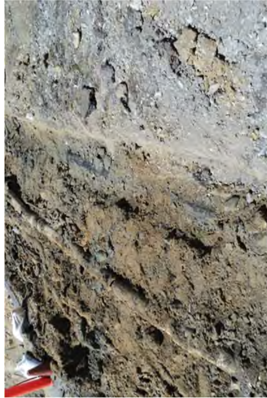
Transite pipe before removal. The steel pipe on the right was chased along the north edge of Unit 2.
