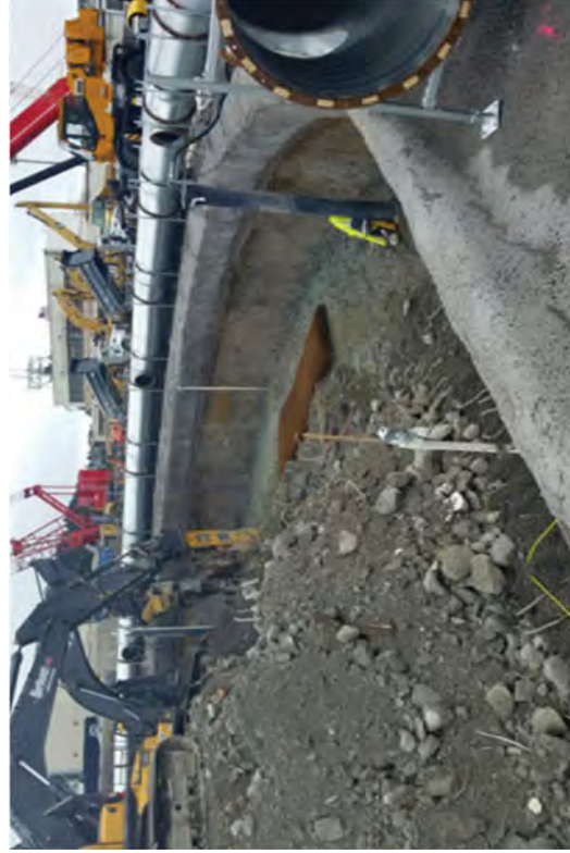
Installing an additional 5 feet of dowel and wire mesh for the portion of shotcrete collar.
