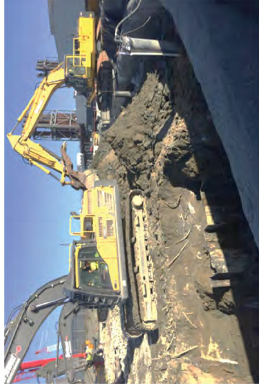
A sheet pile wall at west side of excavation which remained from the plant's initial construction.
