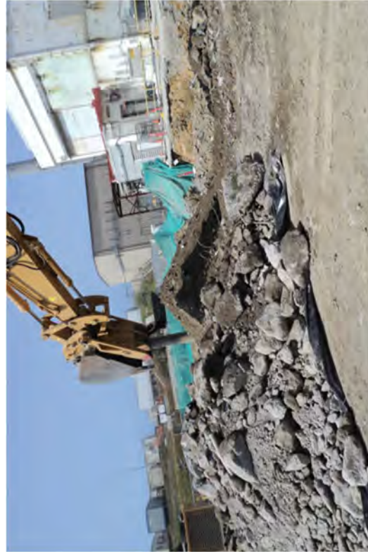
An excavator with a hammer being used to start demolition work on a new area in south central Unit 2.
