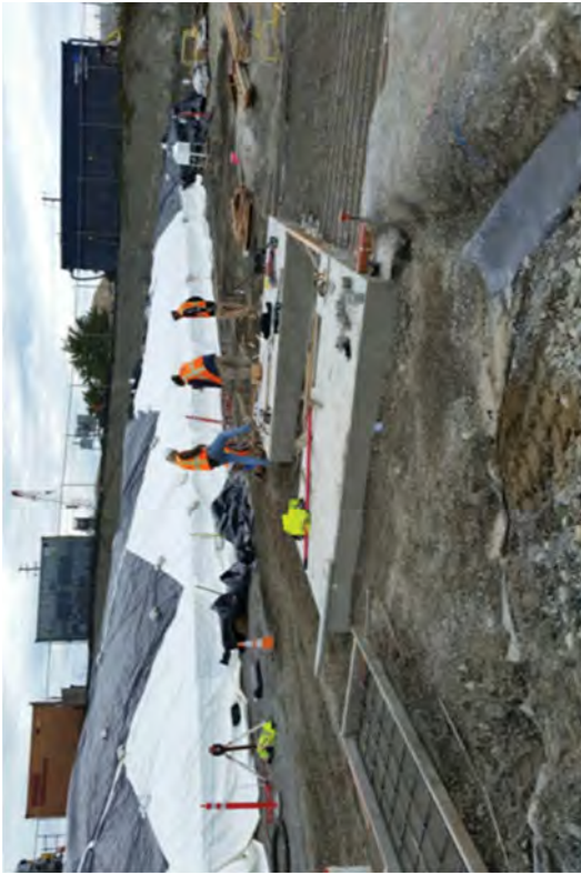
The stair tower pad installed and constructing forms to install the ventilation system.
