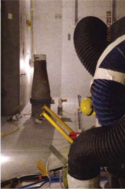
A pipe which needed to be inspected for ACM. The hosing in the foreground supplies the workspaces with proper air ventilation
