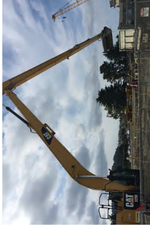
A long reach excavator and dump truck removing gravel from the Unit 2 Intake Structure.
