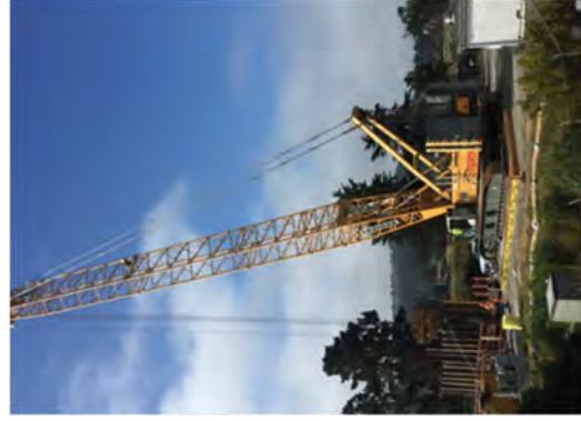
Crew driving sheet piles into the Intake Canal using the 330-ton crane.
