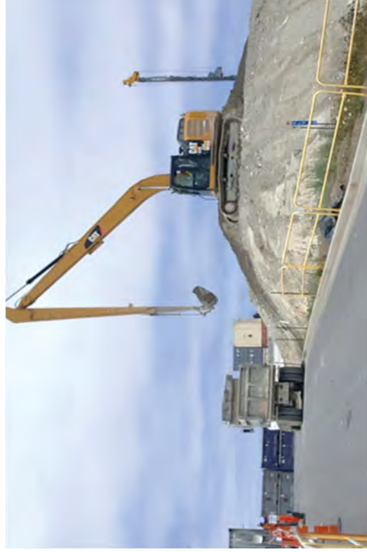
Moving clean fill material from CSM spoils staged in the Discharge Canal to backfill the North Yard.
