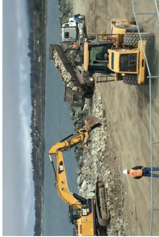
A loader leveling the Coastal Trail area while an excavator spreads rock to create a swale.
