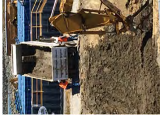
Beginning to stockpile soil that had been screened for re-use in the Discharge Canal.
