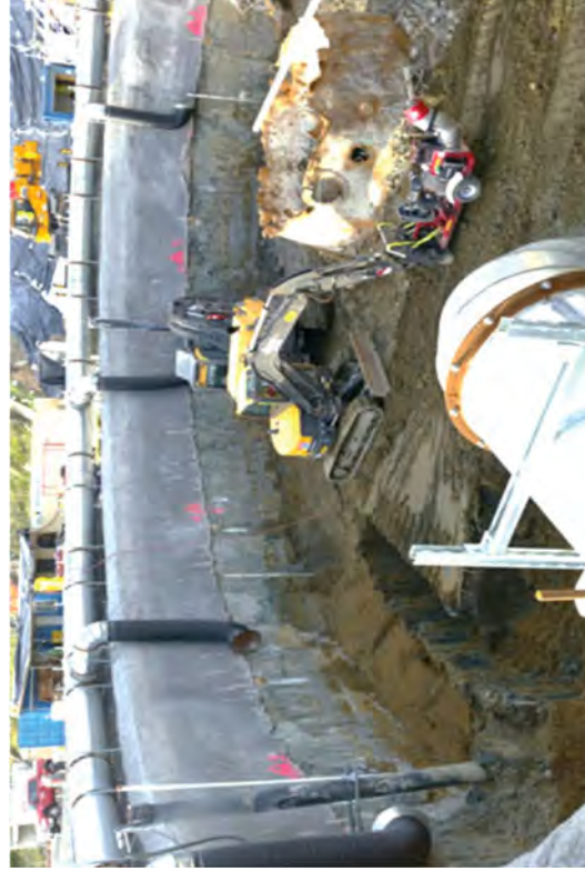
Sheet pile left in place after original plant construction on the west side of the excavation.
