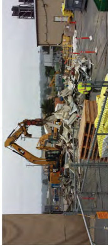
RP characterized and released the entire SRWB for OAD before demolition began.
