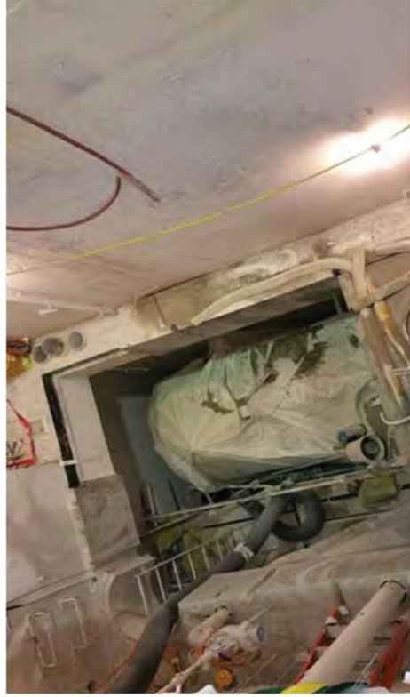
Turbine Building Drain Tank covered for wire saw floor removal of the NFSV.
