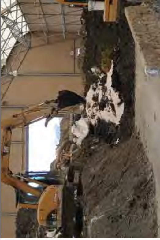
Soils from the Intake Canal in the SMF. Lime was added to help stabilize and dry the loose material.
