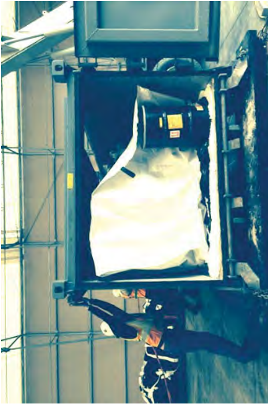
Loading dewatering bags with lead impacted waste into an IM for disposal along with liquid in a 30 gallon drum.
