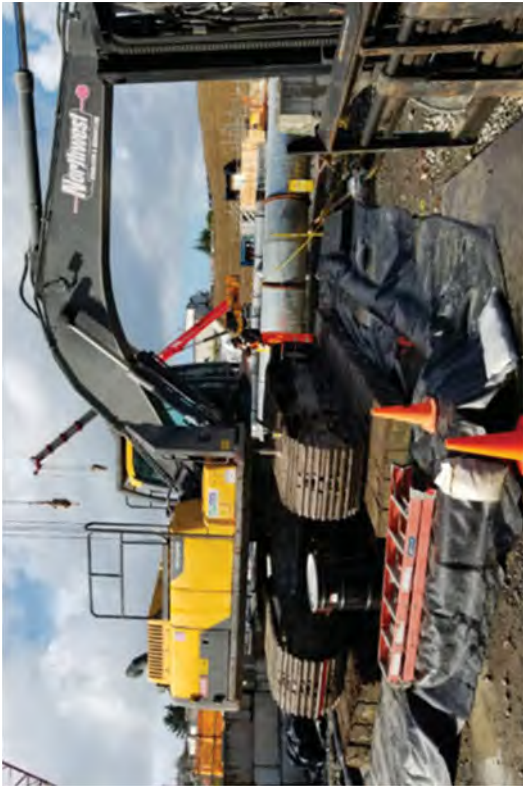
Decontaminating and surveying the excavator after it was removed from the Caisson excavation.
