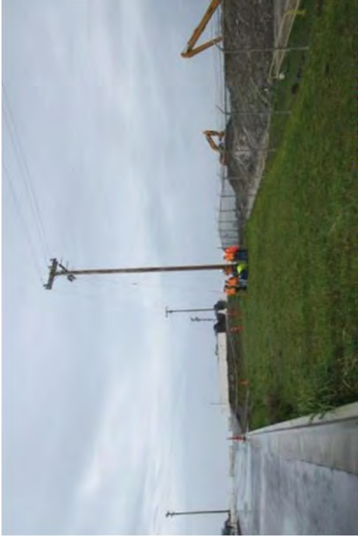
The new power line crossing the center of the Discharge Canal to the new pole at the SMF.
