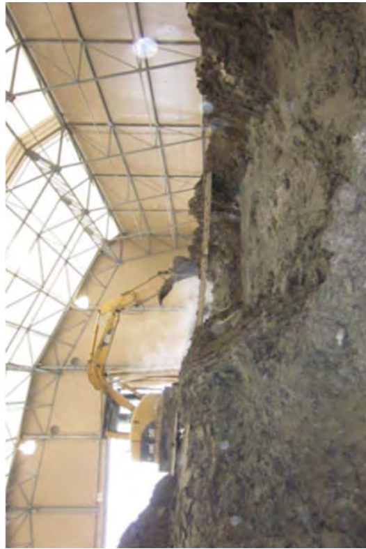
Mixing South Discharge Canal sediment and slurry with the remaining Discharge Canal sediment in SMF. Lime was added to dry and condition it for offsite shipment.
