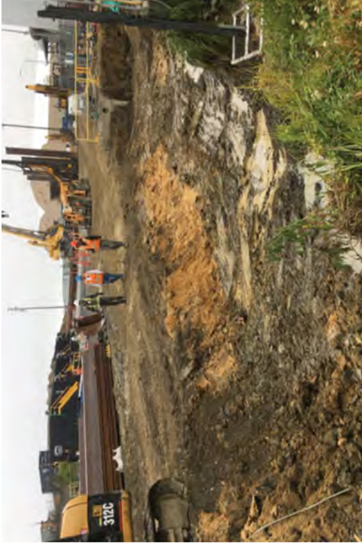
The OWS raceway fully removed and ready for environmental sampling and FSS survey. The LVW sump remains at north end of raceway.
