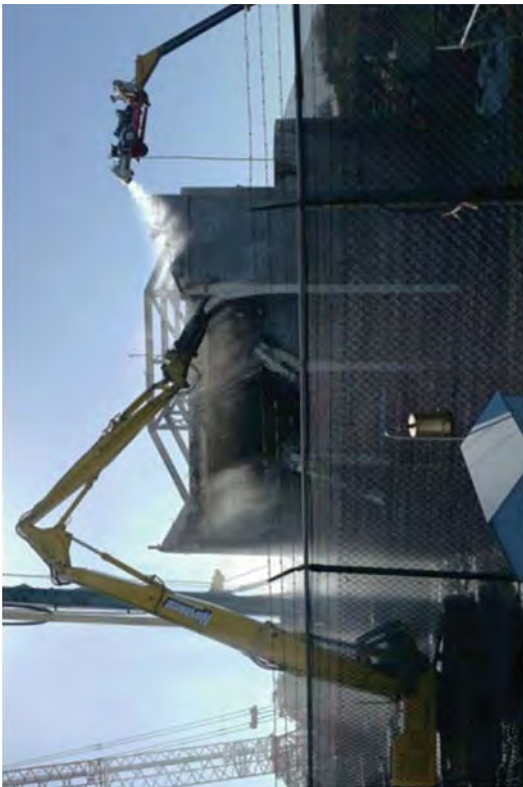
Demolishing the first bay wall of the eastern 40' feet of the RFB.
