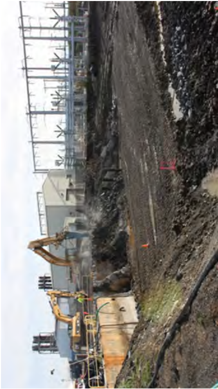
Demolishing the Unit 3 Intake Structure. Water is being sprayed to control dust.
