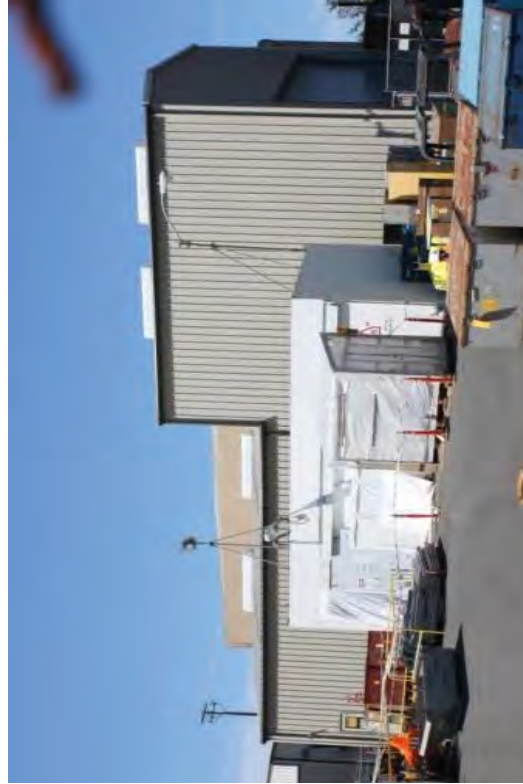
The LLRW Building set-up for Class I containment for friable asbestos abatement in transite panels.
