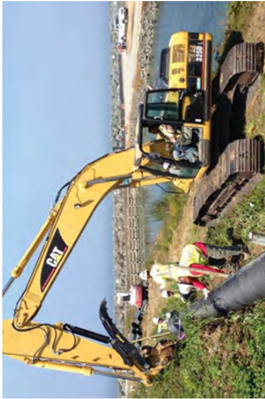
Re-Routing the storm water discharge line from the canal to the Humboldt Bay.
