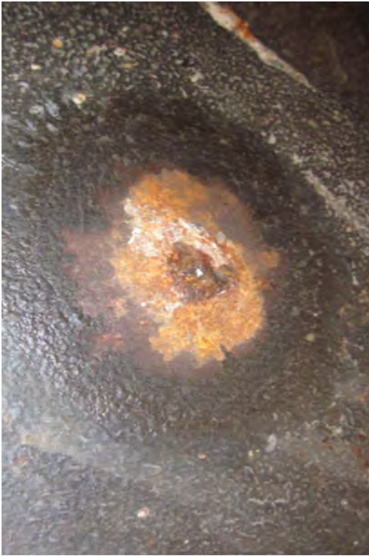
A returned IMI had this puncture with water dripping from it. It was originally thought to be rust degradation.
