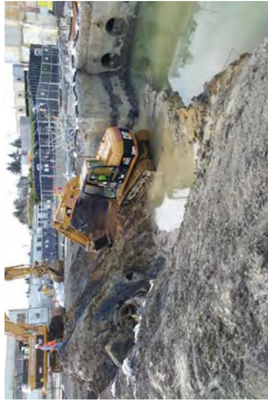
An excavator prepping the HMS trench for FSS and backfilling. The rainy season caused considerable amounts of water runoff to collect in the trench.
