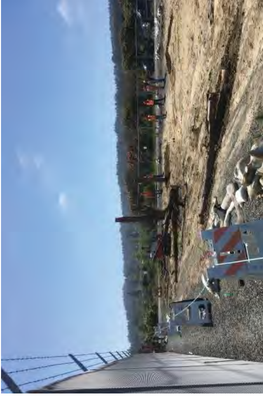
Anchoring snag features in Intake Canal.
