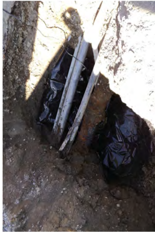
A drain pipe exposed and prepared for an air gap and plug to be installed.
