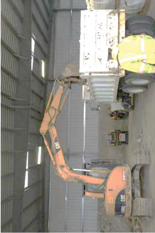
Loading metal from the Intake Canal headworks that was staged in WMF for transfer to and loading into end dumps at Parking Lot B.
