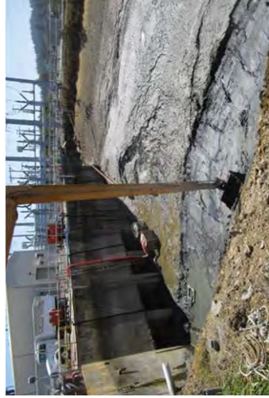
The front of the Intake Structure with gate area. The pumps were used to finish draining the canal and for dewatering from rain.
