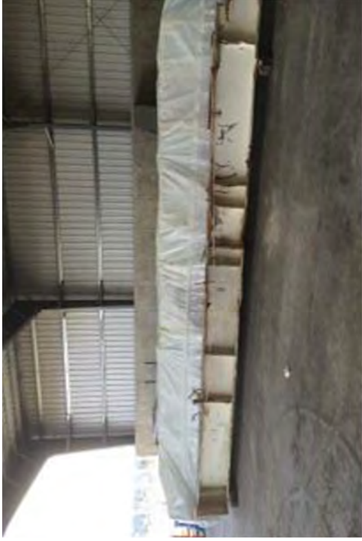
Structural steel from the RFB prepared for shipment to a waste facility on a flatbed trailer.
