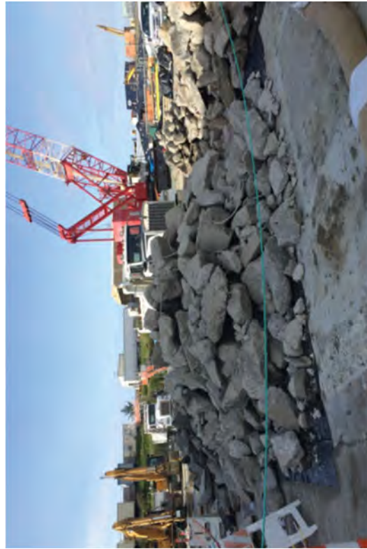
Demolishing and stockpiling the Unit 1 concrete pad before transferring the concrete for processing.
