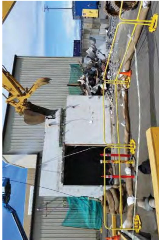
An excavator demolishing the LLRW Building while a high pressure sprayer is used to control dust.
