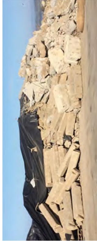
Concrete logs from the Discharge Canal coffer Dam which was moved to the SMF and then to this re-use concrete stockpile.
