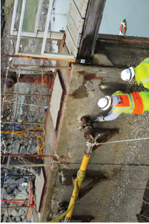
A crew cutting the LRW discharge line from the Discharge Canal Headworks
