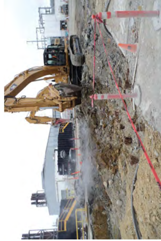
Workers controlling dust using a pressure washer when the excavator hammer is operating.
