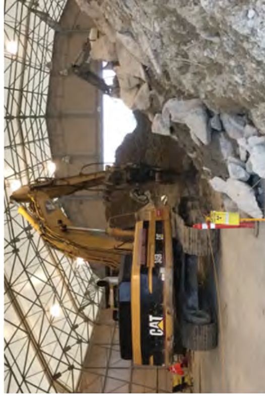
An excavator equipped with a hydraulic ram/concrete crusher size reducing Tremie concrete in the SMF.
