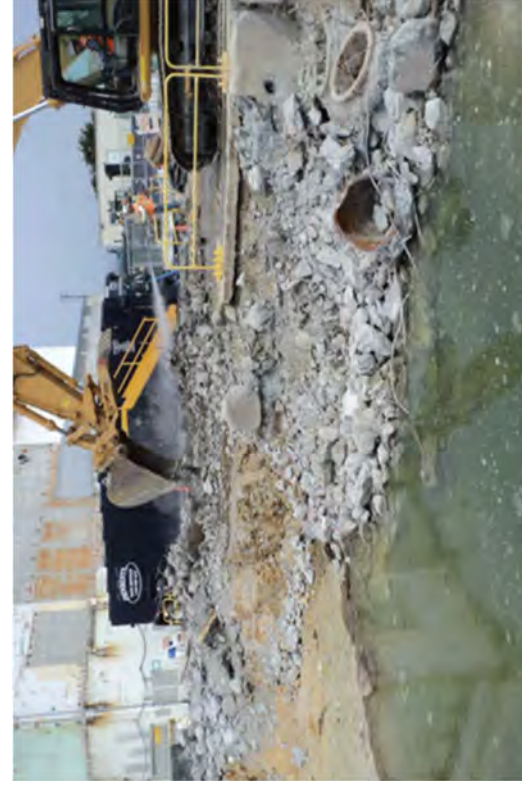
While using dust control measures, rubble is loaded directly into intermodals from the excavation per RP instructions.
