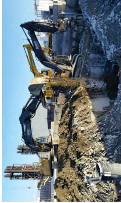
Concrete debris is placed in the west suppression chamber to fill the void.
