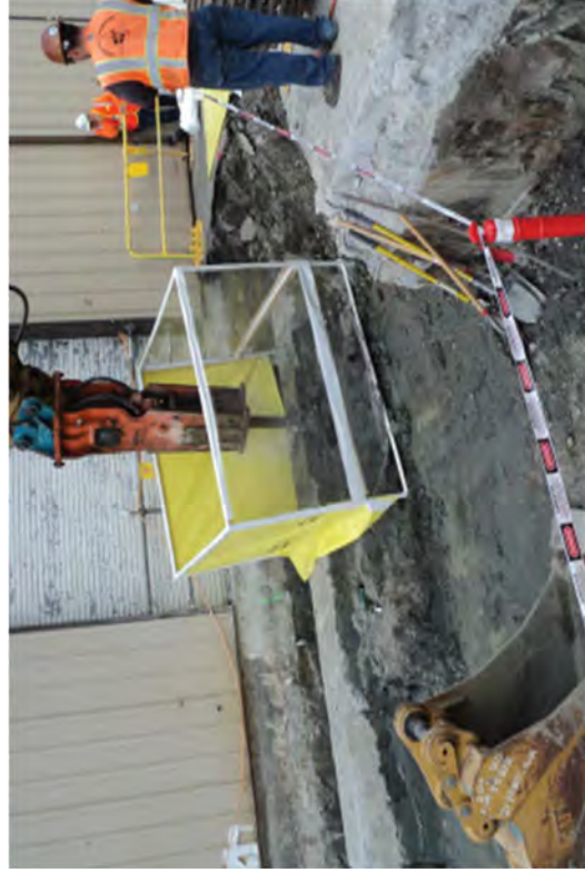
Gently fracturing the raceway to minimize the risk for projectiles while water is sprayed to mitigate airborne dust.
