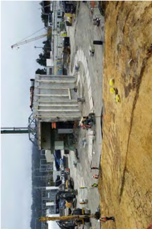
Protective plating was placed over the top of the CSM wall. Protection was also installed on the monitoring wells and their associated equipment.
