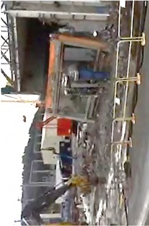
The 75-Ton crane after its planned and controlled drop from the RFB.
