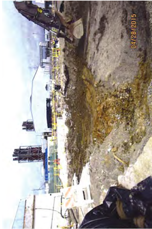
The excavation at a depth of 3 feet below grade at the west end of the TB foundation.
