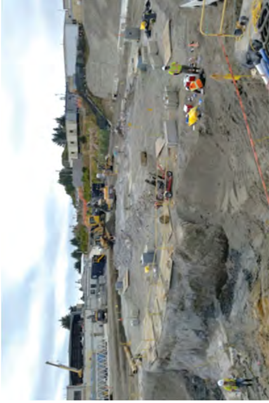
Grading and installing a K-rail in the area outside of the CSM wall.
