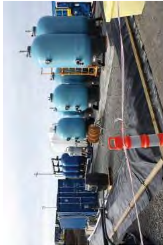
The GWTS installation.
