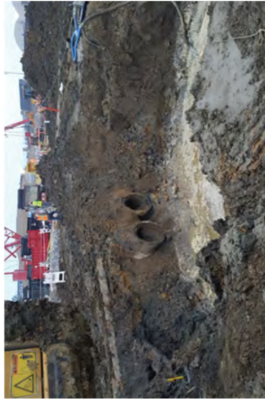
Circulating Water Lines underneath the footprint of Building 5.
