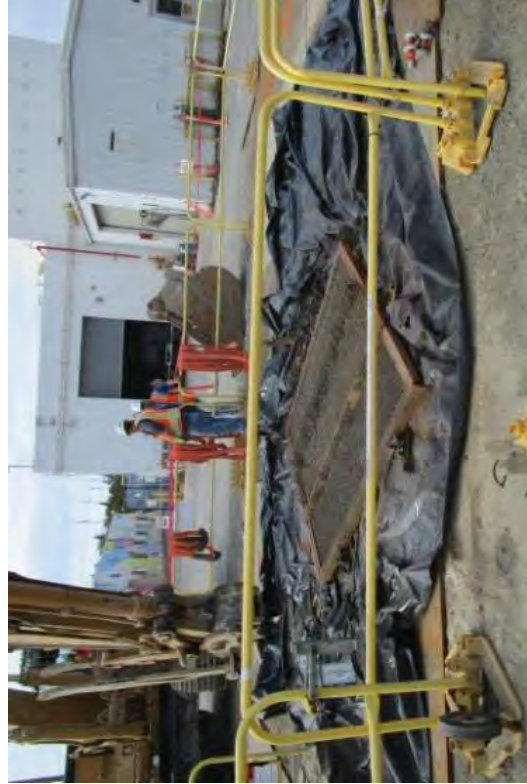
An intake screen that had been left in place.
