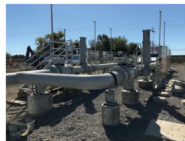
Figure 16 – M&C Complex Station-Above Ground
