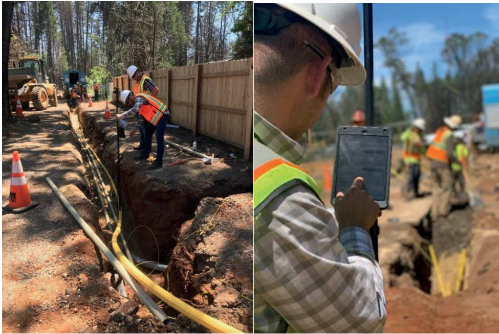
Figure 60 – Capturing material information and geometry of a Joint Trench Project during the reconstruction of Paradise on June 4, 2019.
