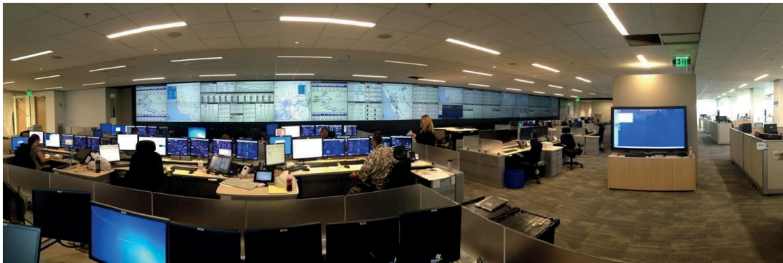
Figure 39 – PG&E’s Gas Control Center Features a 90 Foot-Long Video Wall With Current Operational Information to Augment The Gas SCADA System
