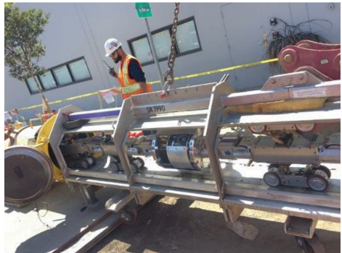
Figure 59 – Insertion of the Explorer In Line Inspection robot in its launcher on line L-105N in Oakland on August 23, 2019
