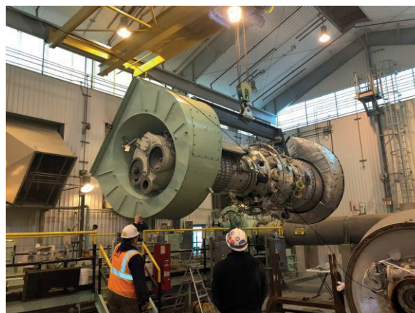
Figure 14 – Delevan Compressor Station Turbine Exchange
