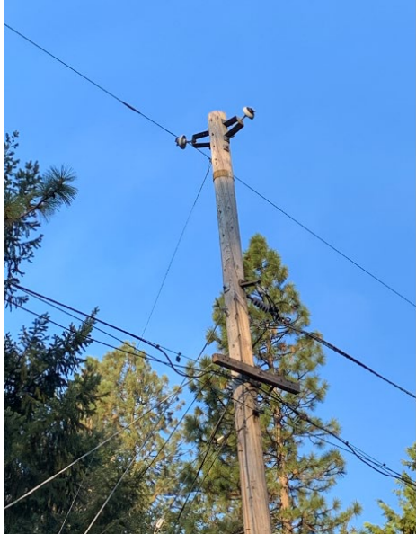
Figure 11: Image of Vegetation Related Damage in Butte County – Broken Insulator and Floating Conductor
