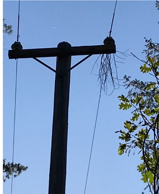
Figure 2 – Vegetation Debris Near 98 Gamble Rd, Oroville
