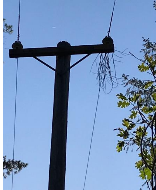
Figure 2 – Vegetation Debris Near 98 Gamble Rd, Oroville
