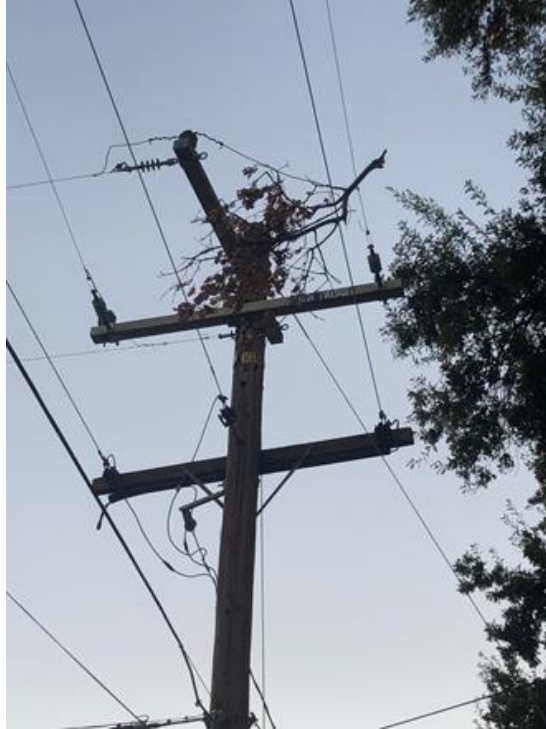
Figure 3 – In Los Molinos, Tehama County Branch Flew Into Primary Conductors
