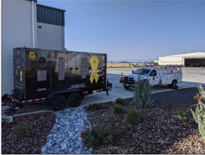
Figure 8 – Mobile Generation at PSPS-Critical Helicopter Hangar
