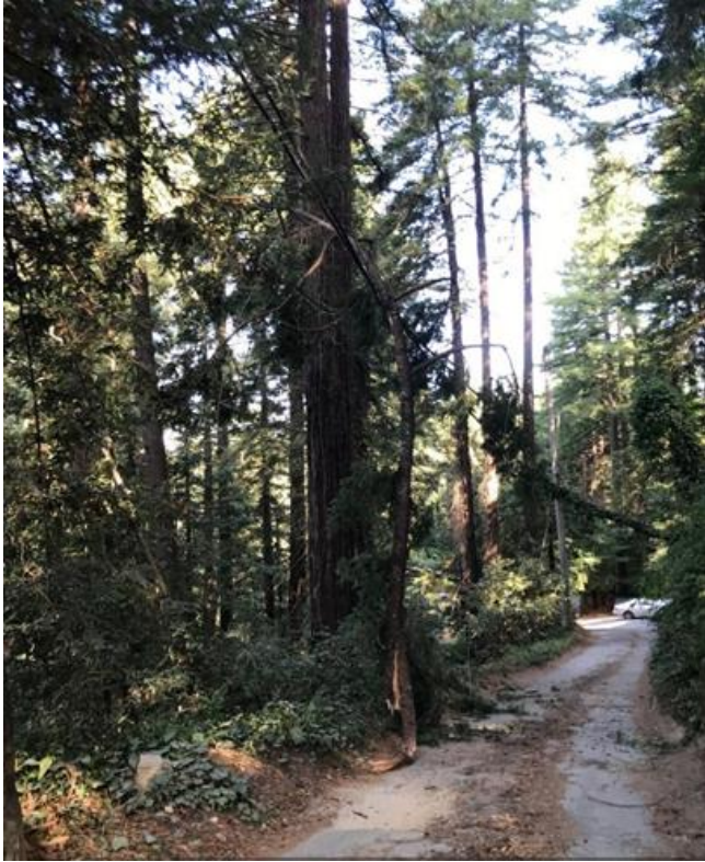
Figure 11 – Near Felton, Santa Cruz County Branch Fell Into Primary and Secondary Conductors
