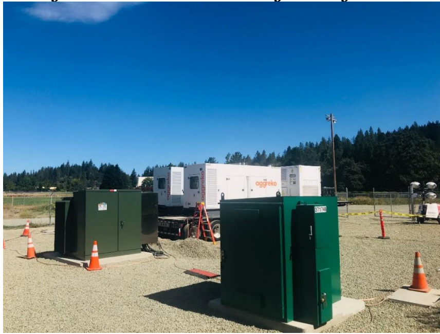
Figure 2 – Mobile Generation Staged at Angwin PIH
