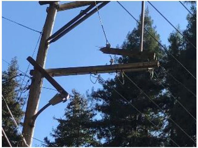
Figure 20: Damage in Santa Cruz County – Broken Secondary Arm
