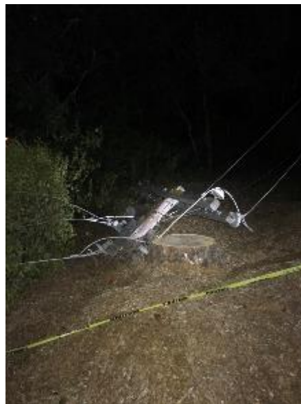
Figure 18: Vegetation-Caused Damage in Napa County – Broken Pole, Lines Down Due to Fallen Tree
