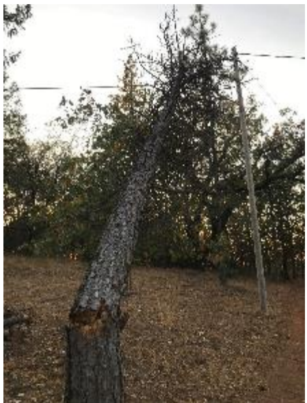
Figure 16: Vegetation Hazard in El Dorado County-Tree Fell on Service Line
