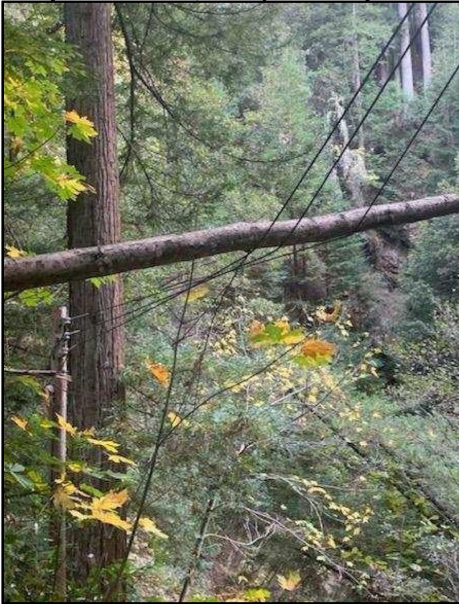
Figure 8: Tree fell onto conductors; Unincorporated area of Santa Cruz County
