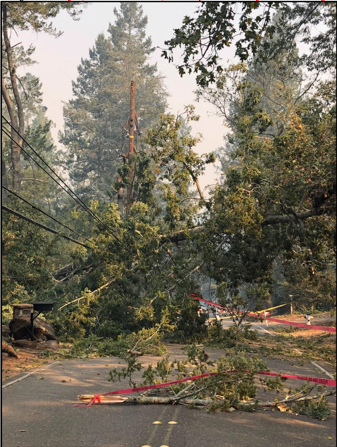
Figure 6: Tree fell, broken conductors; Unincorporated area of Sonoma County
