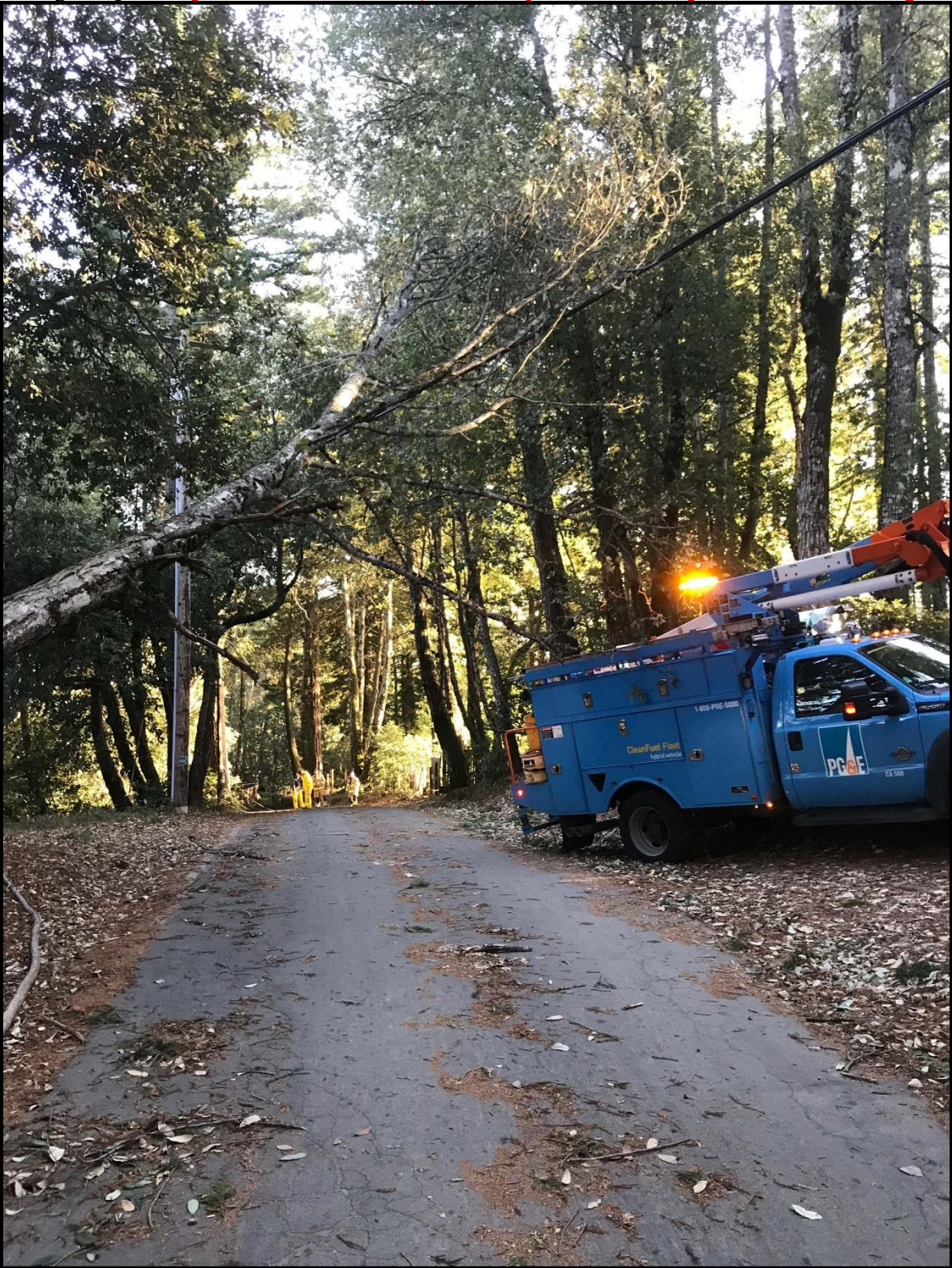
Figure 3: Tree fell onto conductors; Unincorporated area of Santa Cruz County
