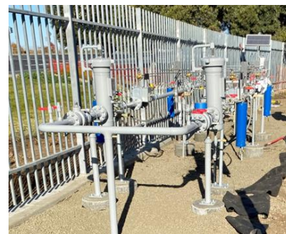
Figure 20 – Large Volume Customer Transmission Station
