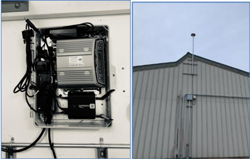
Figure 65 – Installation of GNSS Case Station in Placerville, CA showing the base station (left) and the external antenna (right)
