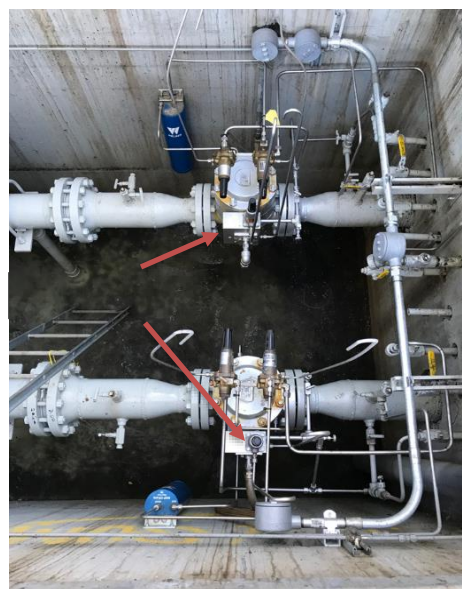
Figure 41 – Photo Pointing to Slam Shut Installations
