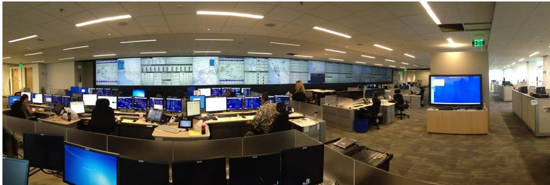
Figure 45 - PG&E’s Gas Control Center Features a 90 Foot-Long Video Wall with Current Operational Information to Augment The Gas SCADA System
