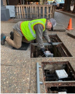
Figure 22 – PG&E Employee Working on Customer Connected Equipment
