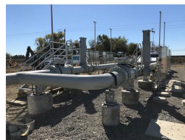
Figure 19 – M&C Complex Station-Above Ground
