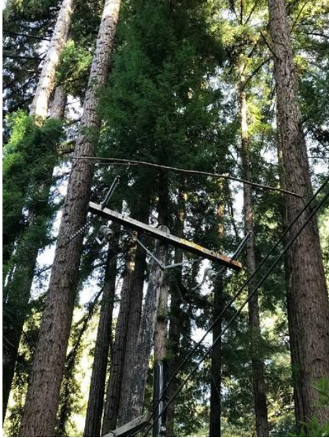
Figure 10 – In Boulder Creek, Santa Cruz County Branch in Contact Cross Phase Conductors
