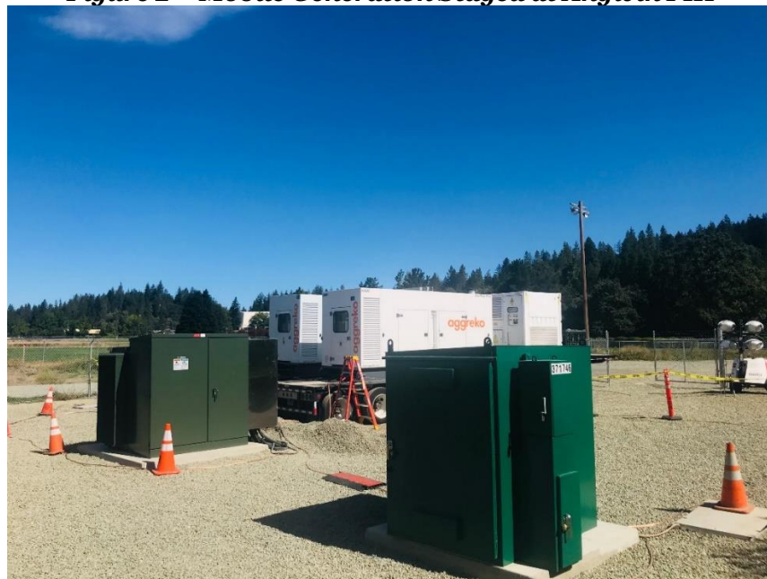
Figure 2 – Mobile Generation Staged at Angwin PIH
