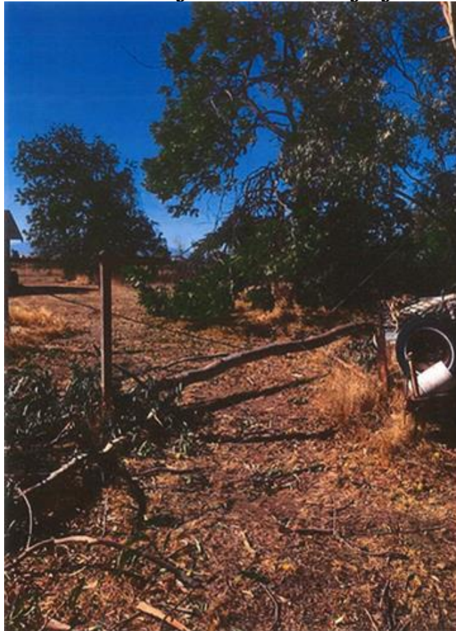
Figure 2 – In Artois, Glenn County Branch Fell Onto Secondary Conductors Bringing Down the Lines
