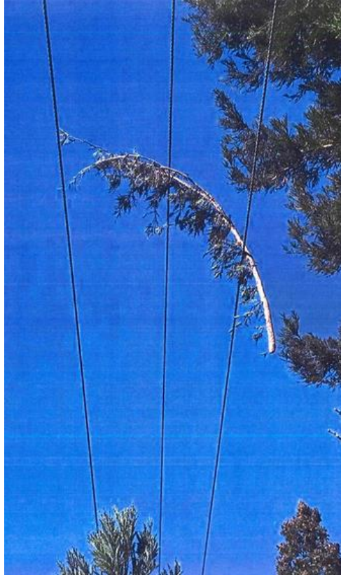
Figure 4 – In Cottonwood, Shasta County Branch Flew Into Primary Conductors
