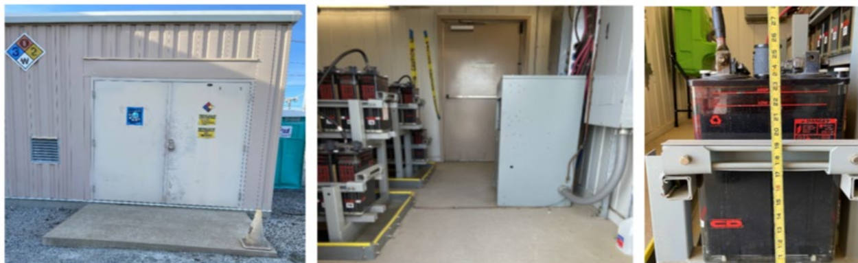
Figure 3.1.1-32. (left) Battery room in the Ravenswood Substation; (middle) inside the battery room with the battery charger on the right, ground level, and DC batteries on the left; and (right) batteries showing the height from ground level inside the battery room. The vent is the tall round cylinder behind the measuring tape.
