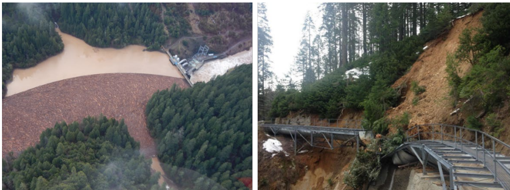
Figure 3.1.3-4. Woody tree debris captured by log boom in 2017 at the Pit 6 dam (left); landslide damage to PG&E's water conveyance (right).
