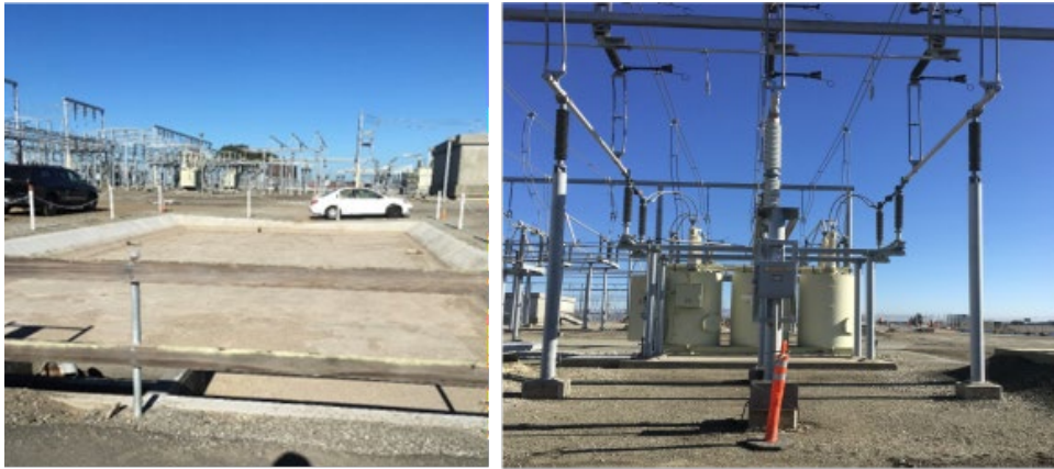
Figure 3.1.1- 31. Ravenswood Substation spill retention pond (left) and oil-filled circuit breakers (right).
