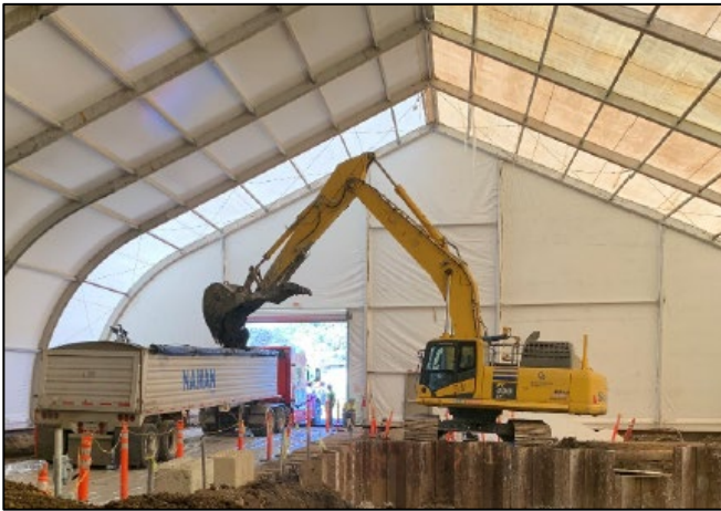
Soil was excavated inside of a tent to control dust and odors.
