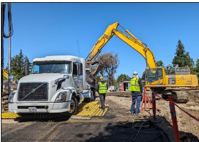
Excavated soil was loaded onto trucks for off-hauling to a licensed disposal facility.
