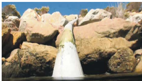
Segment 3 at 39:38 run time with cable in conduit running up shore revetment.
