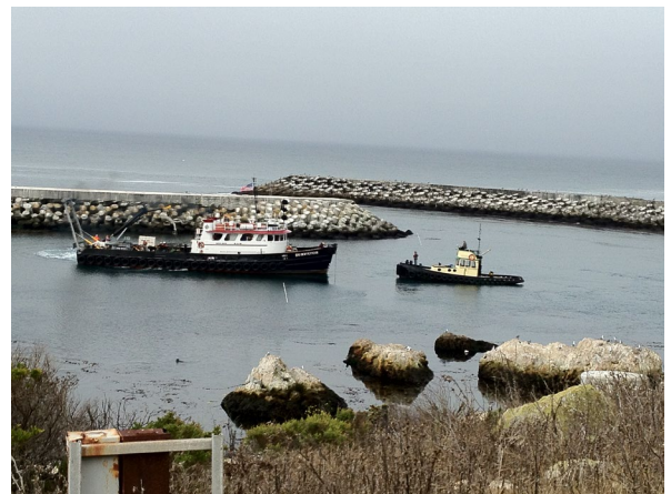
(d) Surveyor (large boat) lays cable in intake. Tugboat stays between boat and intake structure on the right (not shown)
