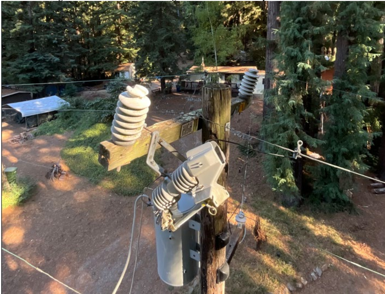
Figure 16: Wind Related-Damage in Santa Cruz County – Broken tie wire
