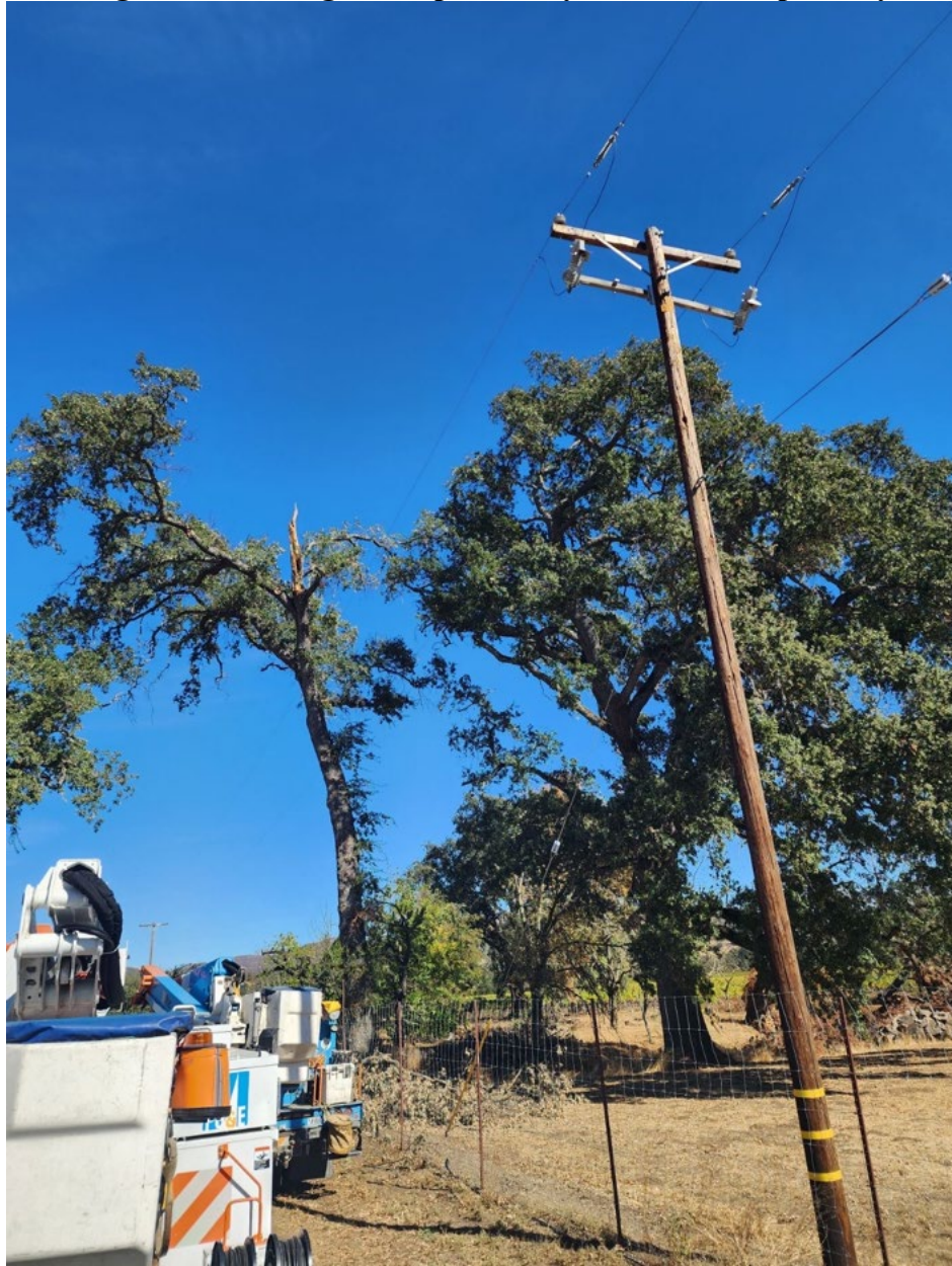
Figure 17: Vegetation-Damage in Napa County – Tree fell on primary conductor
