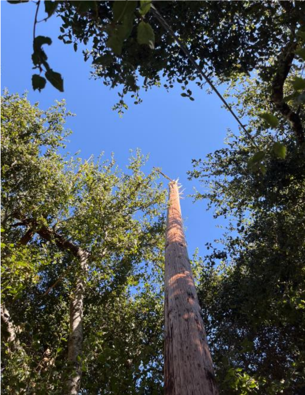
Figure 28: Vegetation-Damage in Santa Cruz County – Broken pole top
