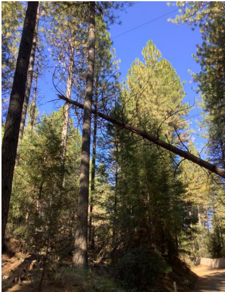
Figure 24: Vegetation-Damage in Butte County – Tree fell on primary line, broke pole top and crossarm
