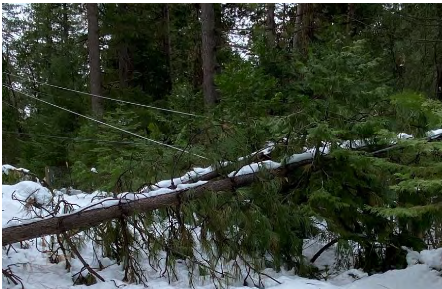
FIGURE PG&E-22-11-3: COVERED CONDUCTOR EFFECTIVENESS – EXAMPLE 3
