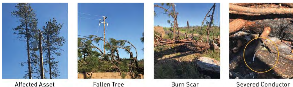
FIGURE PG&E-22-11-1: COVERED CONDUCTOR EFFECTIVENESS – EXAMPLE 1
