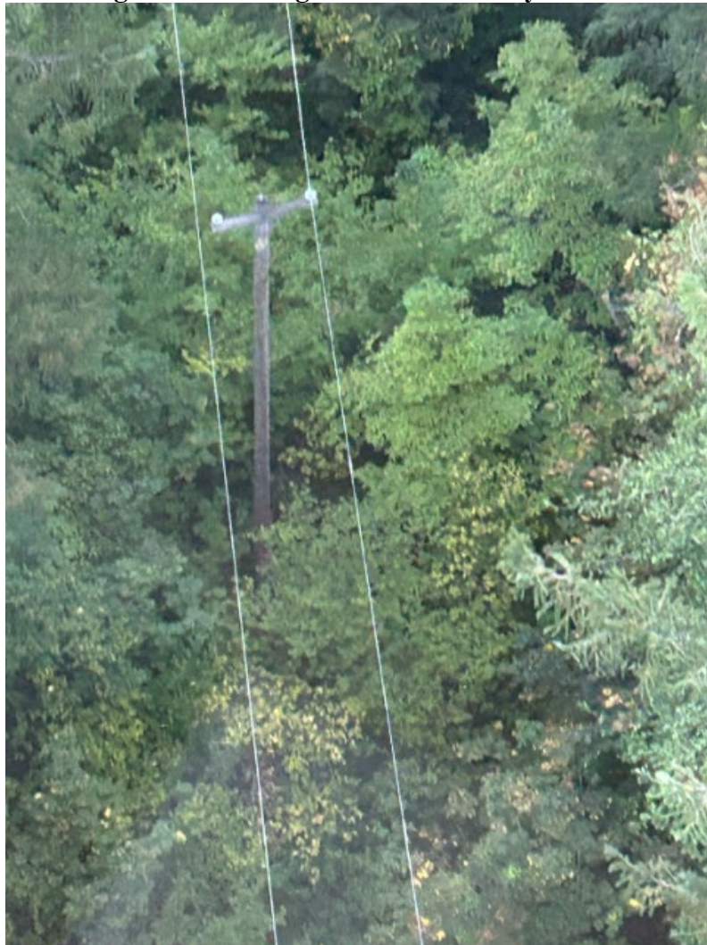
Figure 13: Vegetation-Damage in Shasta County – Broken Tie Wire
