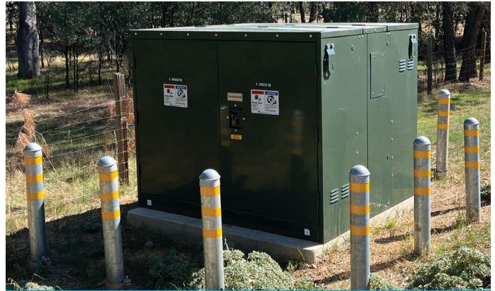
Pad Mounted Transformer Switch with Bollards
