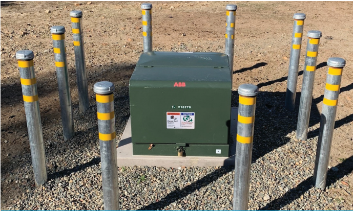
Pad Mounted Transformer with Bollards
