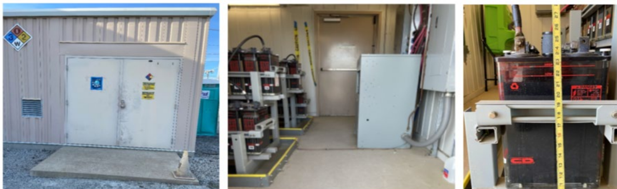
Figure 3.1.1-32. (left) Battery room in the Ravenswood Substation; (middle) inside the battery room with the battery charger on the right, ground level, and DC batteries on the left; and (right) batteries showing the height from ground level inside the battery room. The vent is the tall round cylinder behind the measuring tape.
