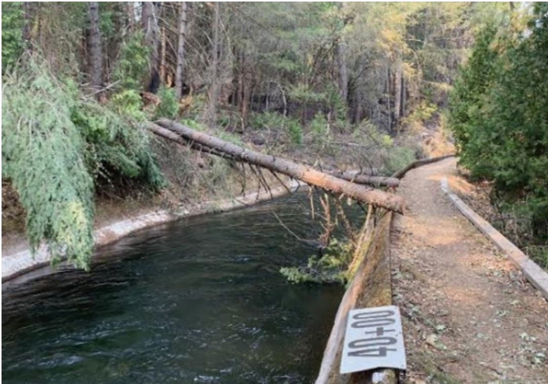
Figure 3.1.3-9. In summer 2021, the River Fire in Nevada and Placer counties, California, in damaged PG&E's Bear River Canal. Impacts included damaged signage, trees, and other debris deposited into water conveyances and culverts, blocked roads and paths providing access to hydro assets, and increased slope stability issues.
