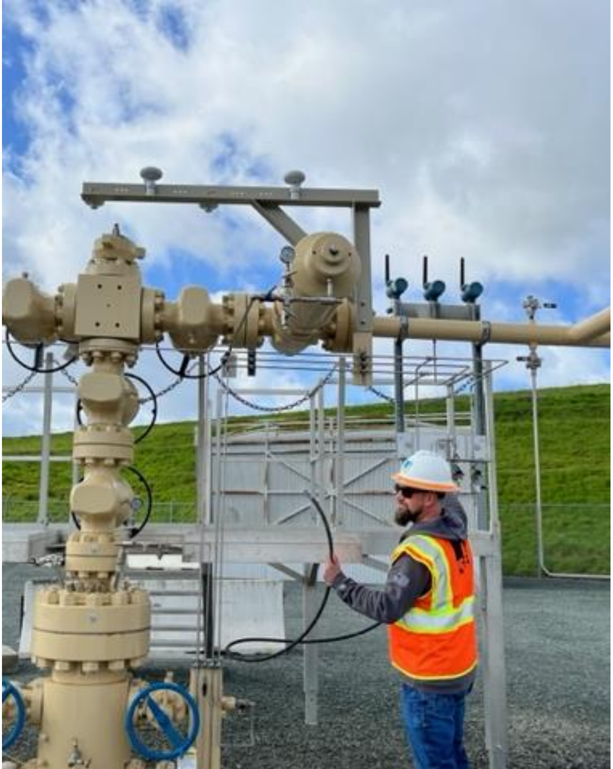
Figure 4: The near field fixed monitoring project is testing the technical specifications and leak detection capabilities of various methane sensors for continuous monitoring of wellheads at underground storage facilities. Incorporating fixed methane monitors can reduce operating risks through early detection of high-risk methane leaks, potentially preventing loss of containment.
