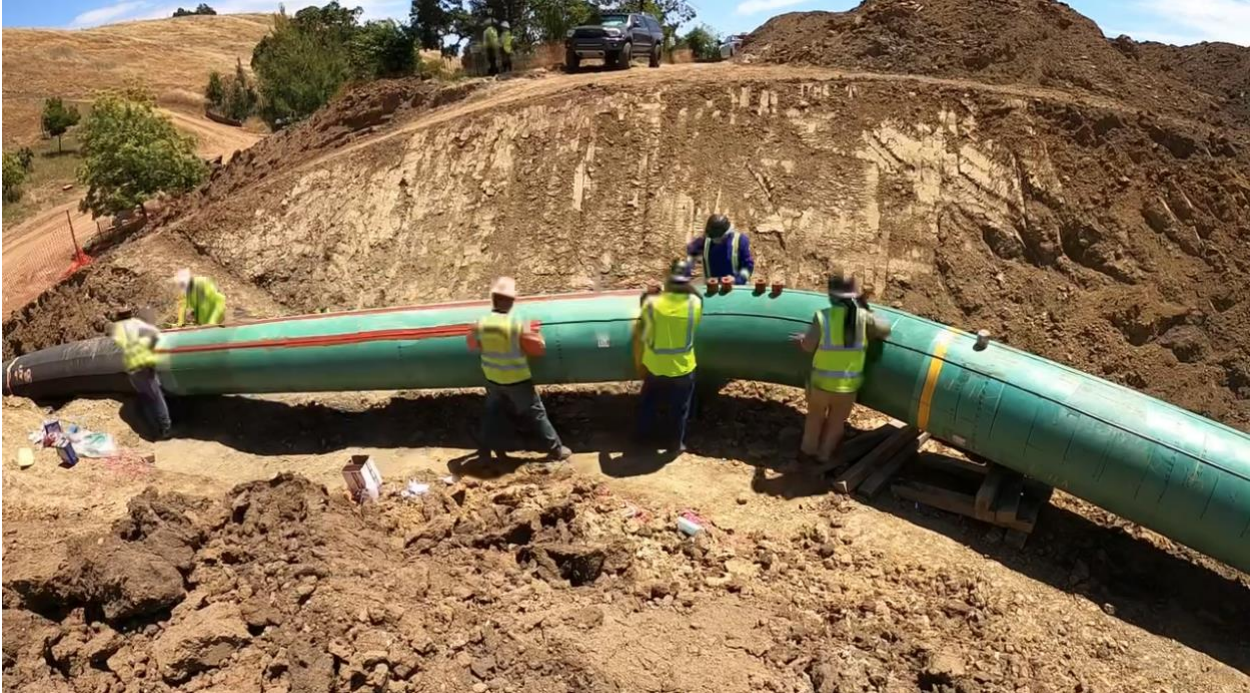
Figure 3: Funded by a US Department of Transportation/PHMSA University grant and Small Business Innovation Research funds, the project involved the first of its kind installation of a distributed fiber optic sensor monitoring system to assess pipeline strain associated ground movement at the Calaveras fault-crossing south of San Jose. The image captures the installation of the fiber optic sensor on the pipeline.
